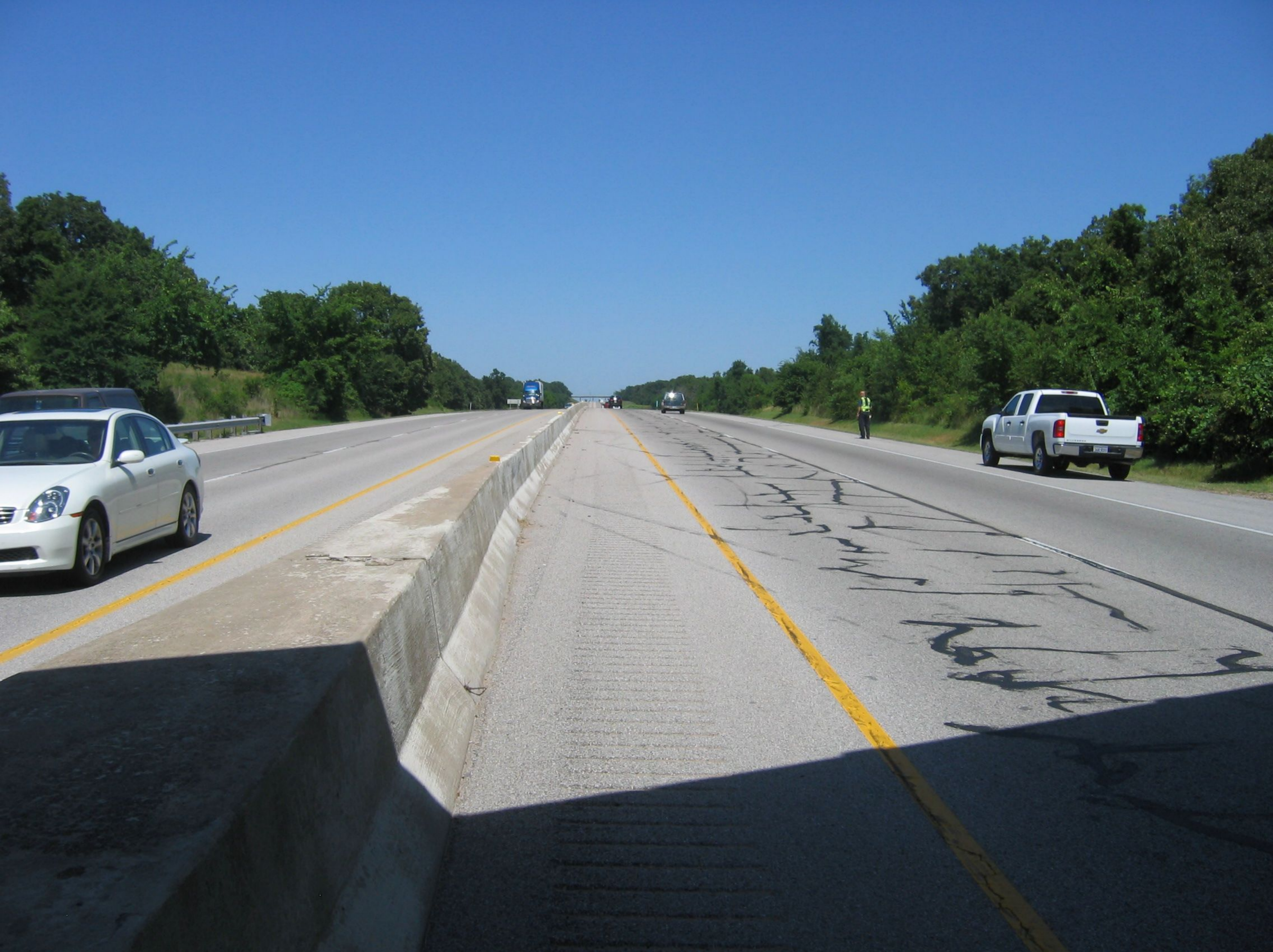
HWY Photo 21, Additional View of Passenger Car Tire Marks into Median Barrier
