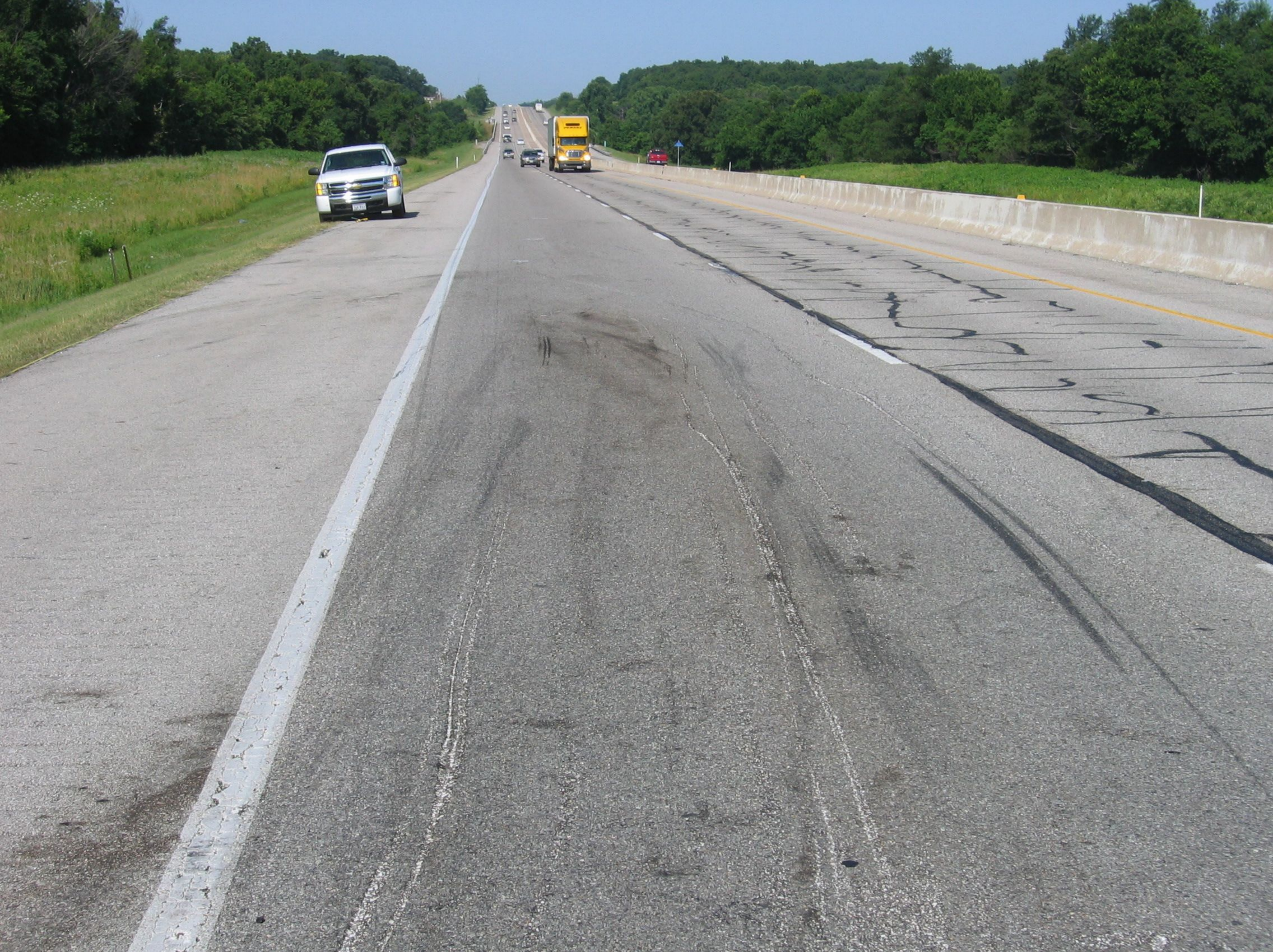
HWY Photo 16, Continued Opposite Direction View of Gouges and Tire Marks
