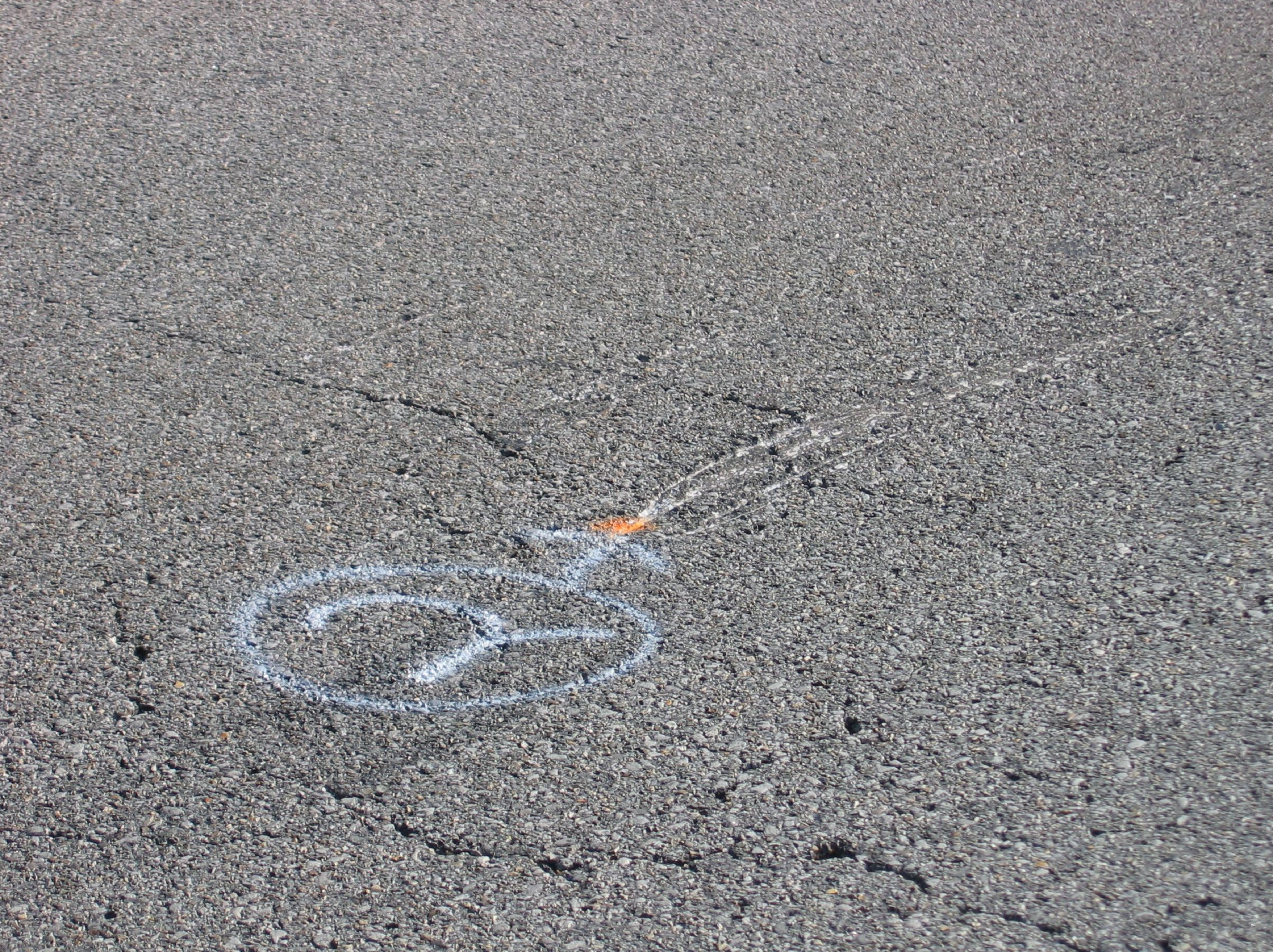
HWY Photo 12, Close-up View of 2nd Impact Area
