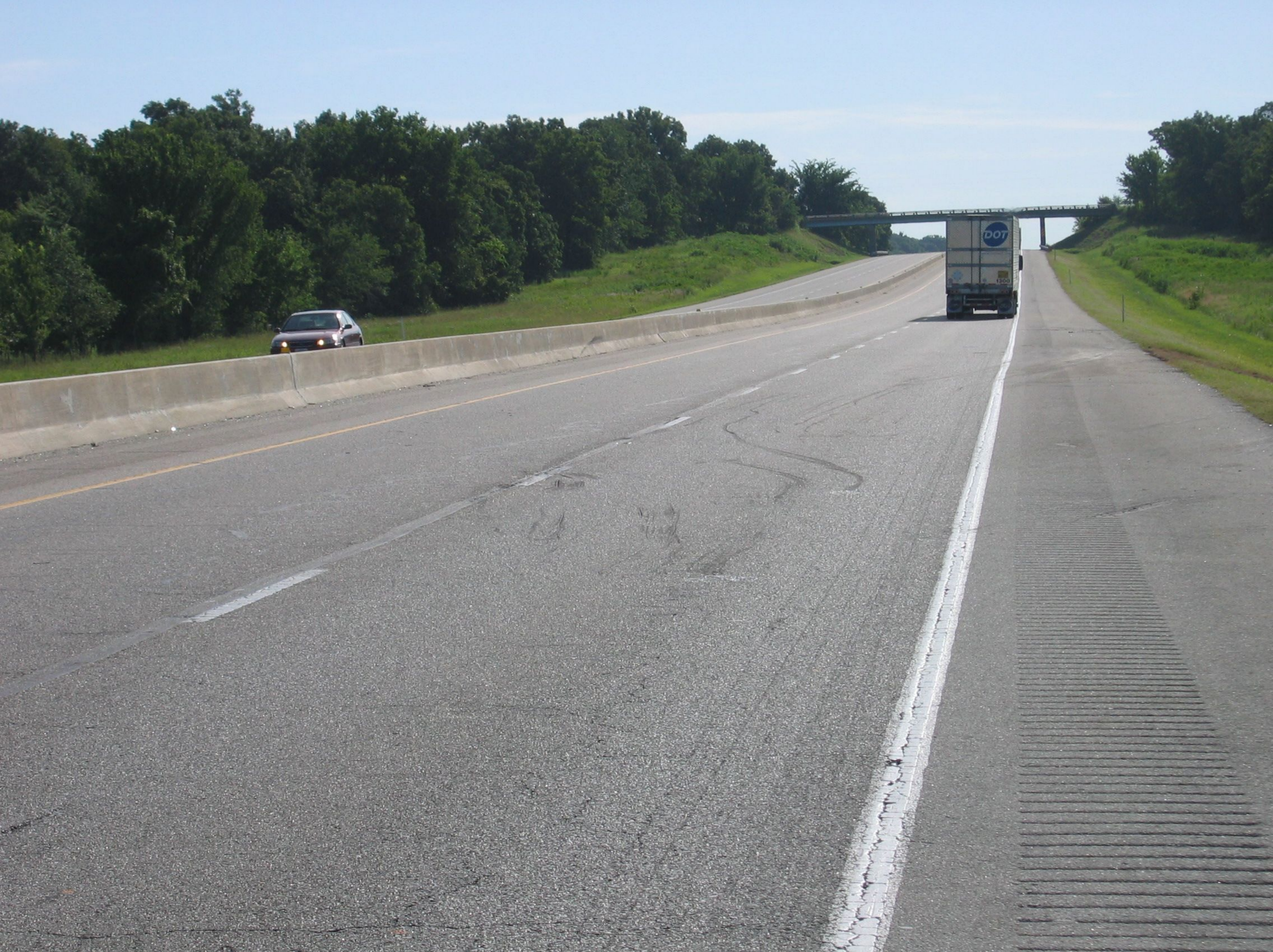
HWY Photo 10, View of Gouges in Pavement Where Impact occurred.
