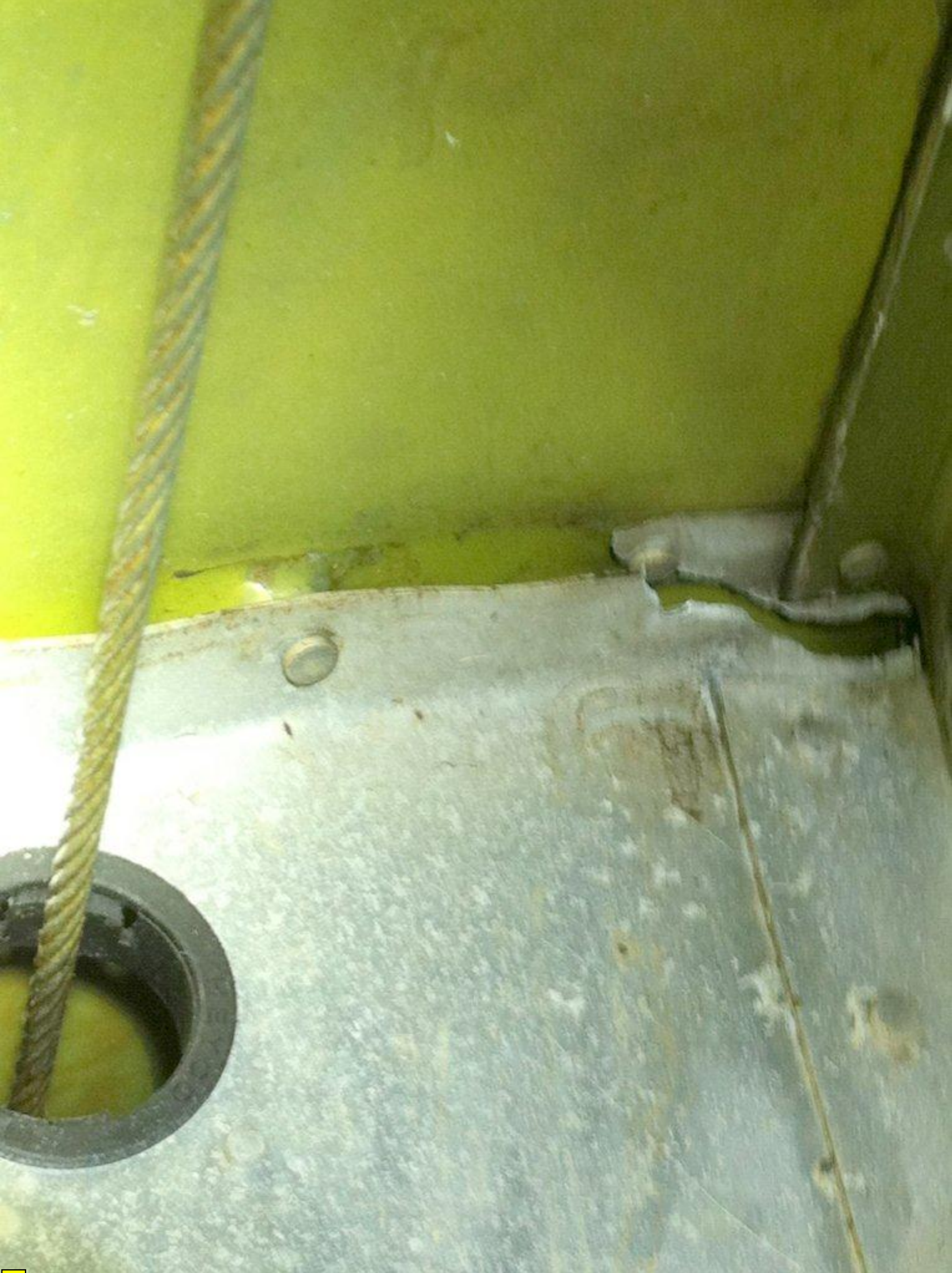
Fractured Rib Flange
