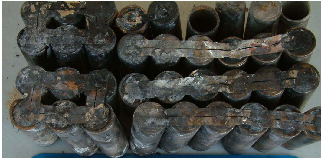
Figure 29: 36-cell lithium-ion battery pack with multiple vented cells
