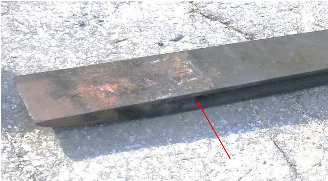
Figure 21. Localized thermal damage (highlighted with red arrow) to surface of nose piece rail.
