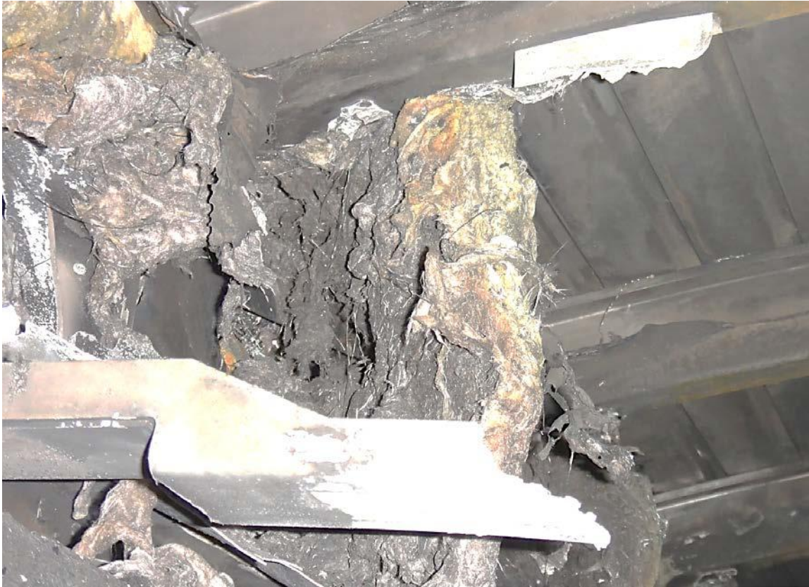
Figure 24. Damaged cable run hanger located above the toilet.
