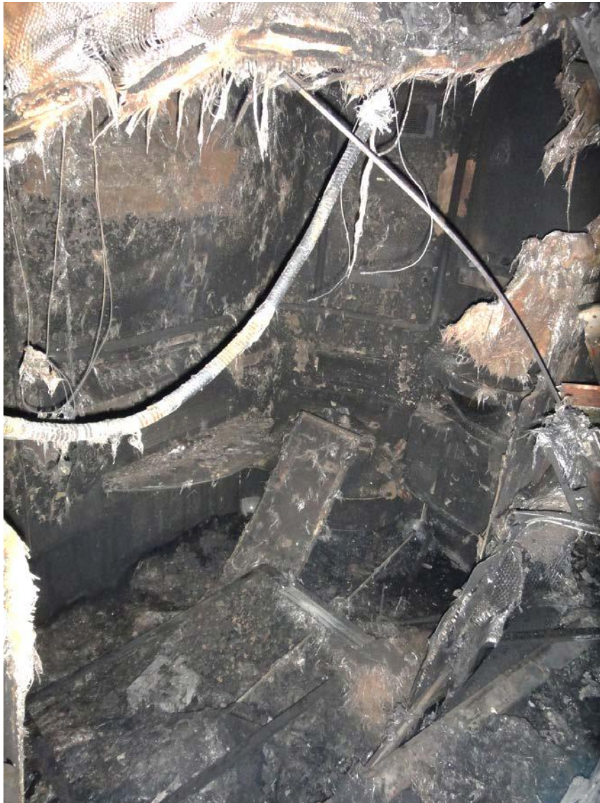
Figure 25. Damaged toilet module.
