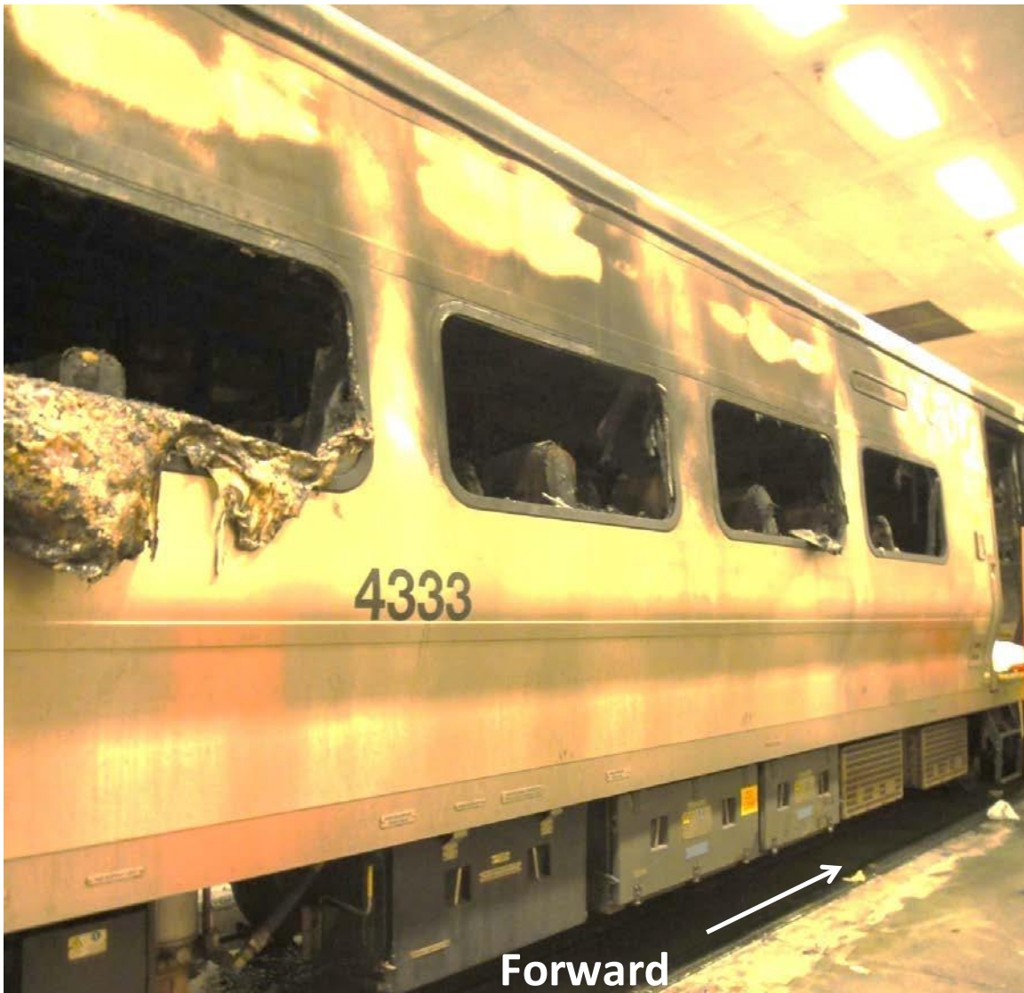
Figure 12. Right side exterior from second (R2) to fifth (R5) passenger compartment windows.
