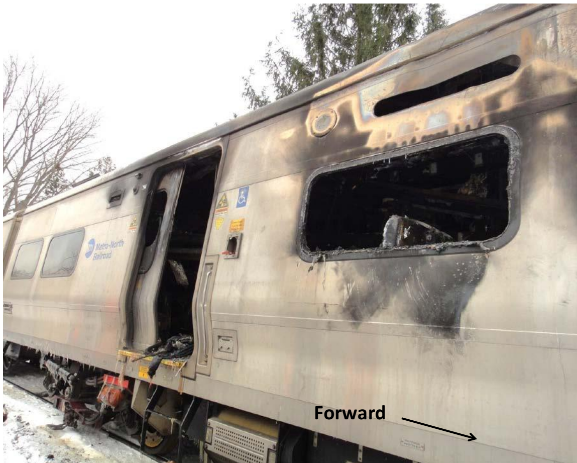
Figure 14. Right side exterior including seventh (R7), eighth (R8) and ninth (R9) windows and rear passenger door.
