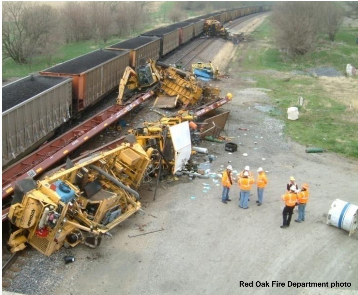
Figure 8. View of wreckage from highway overpass facing west.
