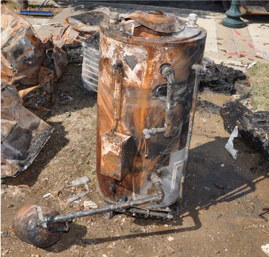
Figure 14. Hot water heater at the accident scene after the explosion. (Photograph provided by ATF.)
