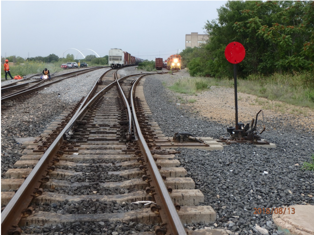
Figure 2 This is the switch that governs movements into track 400 or for a diverging route into tracks 401 or 402. Photo shows switch target (red) is perpendicular to track 400 indicating that the switch is lined for diverging route for tracks 401 or 402.
