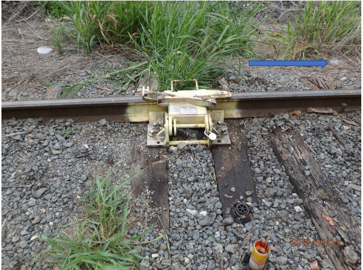
Figure 4 NTSB Photo, on the left is the yellow derail in track 400. The blue arrow points to white paint on the ground, the location where the conductor switch keys were found.
