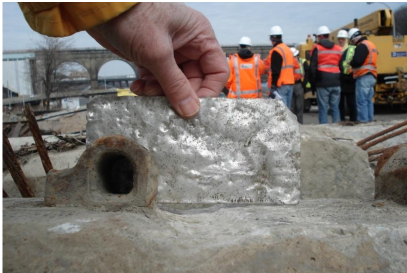
Figure 14: Groove worn into field side of rail seat
