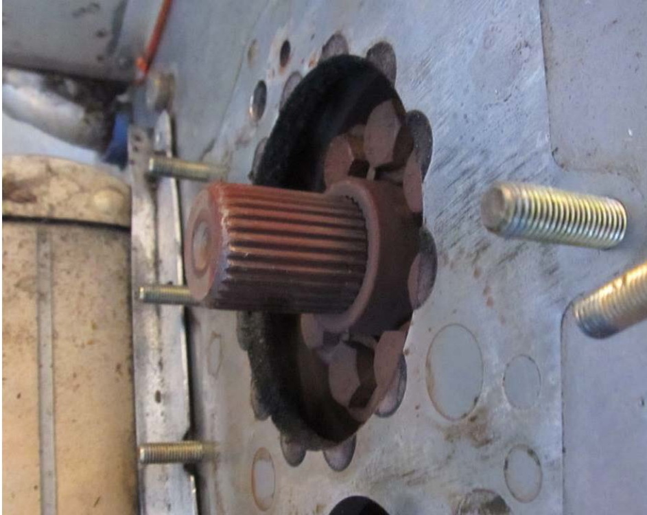
Photo 3 – The spline shaft is inserted into the drive disk adapter. A puller was used to remove the spline shaft and bearing. Red dust coated the spline shaft. Much of the dust could be picked up with a magnet. Examination indicated that the dust was the consistent with fretting corrosion.
