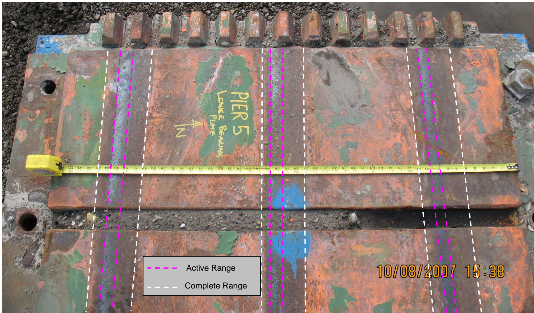
Figure 45. Roller wear indications in the lower bearing sole plate at Pier 5.
