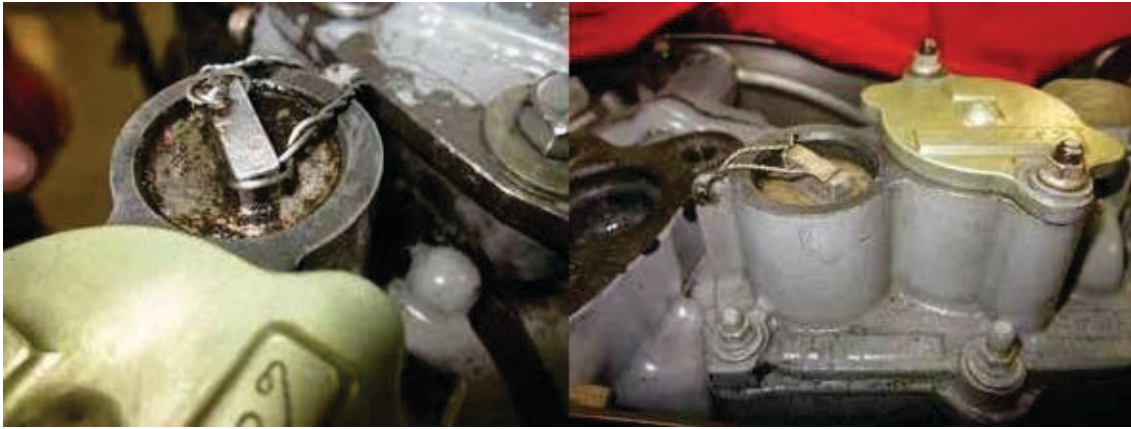
Figure 16, Oil Pressure Regulator (N405MR) Figure 17, Regulator set to nominal setting
