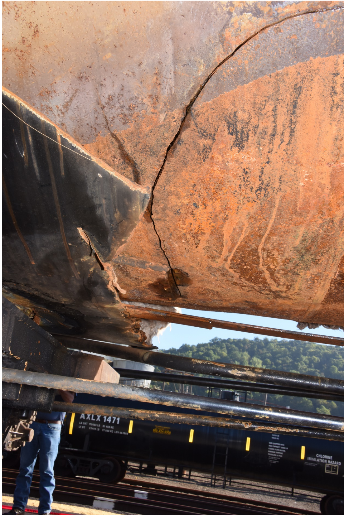
Tank car AXLX1702 shell crack as found after jacket and insulation removal, August 29, 2016
