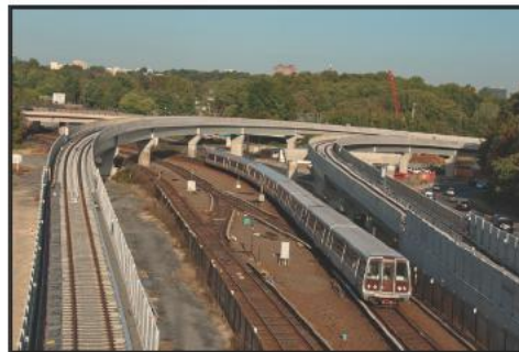
The new Silver Line, currently under construction, will connect with the Orange Line at East Falls Church.
