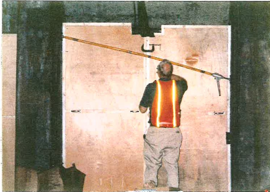
WOOD DAMPER AT N.Y. AVE FAN SHAFT
