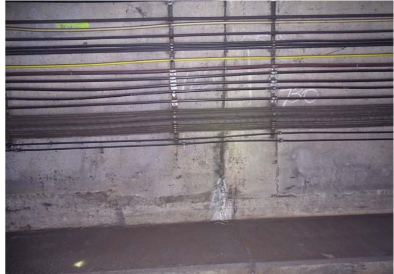
Photograph No. 114 Station 72+60 - crack and stain on the east wall.
