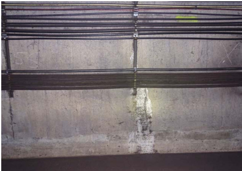
Photograph No. 215 Station 73+00 - crack and efflorescence on west wall.
