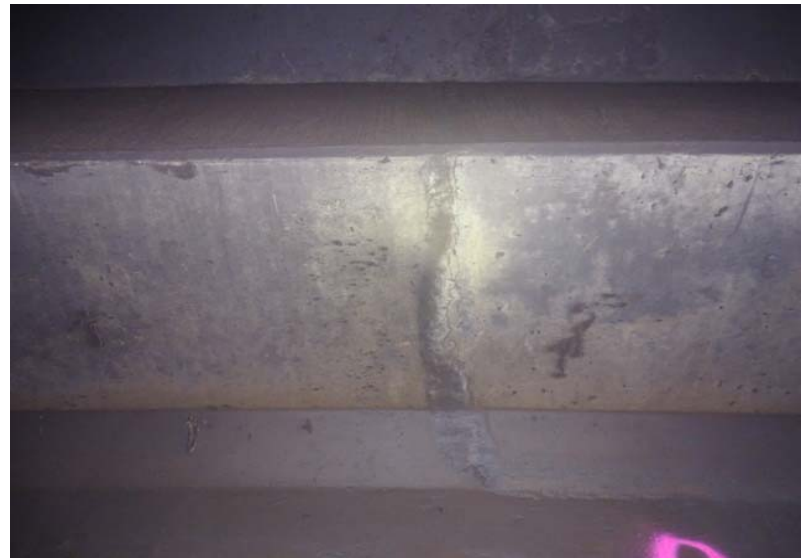
Photograph No. 316 Station 74+50 - crack on catwalk.
