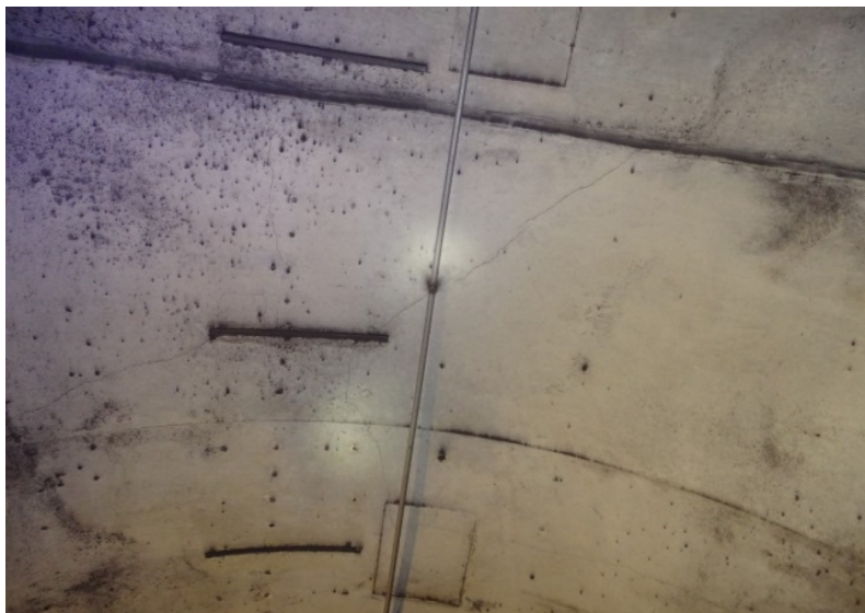
Photograph No. 347 Station 78+35 - crack in ceiling.
