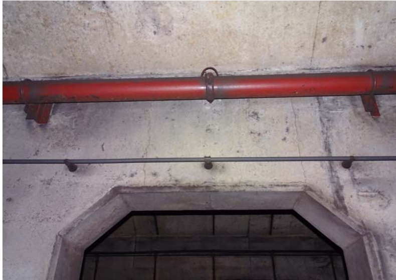
Photograph No. 89 Station 72+00 - cracks above west arch.
