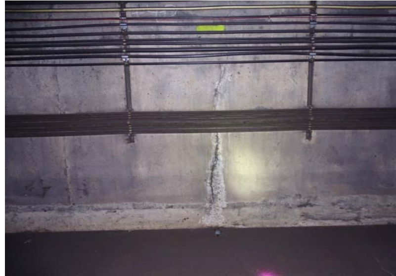
Photograph No. 162 Station 72+20 - crack and efflorescence on west wall.
