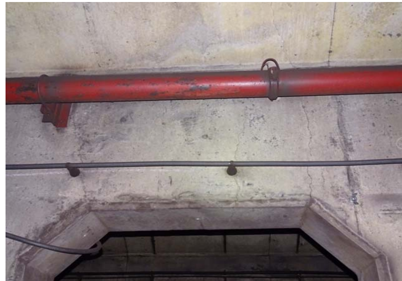
Photograph No. 108 Station 72+40 - cracks above west arch.
