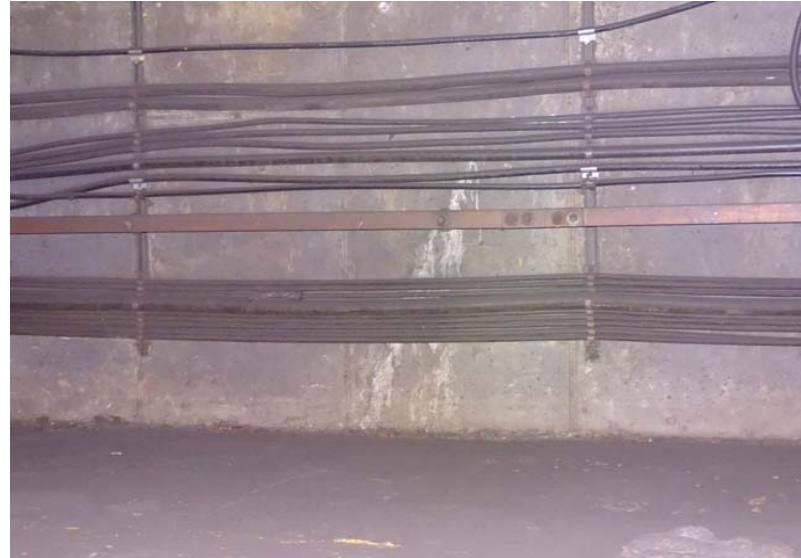
Photograph No. 42 Station 70+40 - crack and efflorescence on the west wall.
