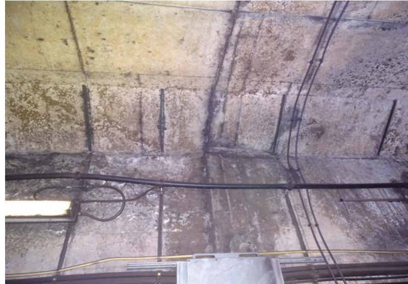
Photograph No. 42 Station 70+80 - stains on the east wall.
