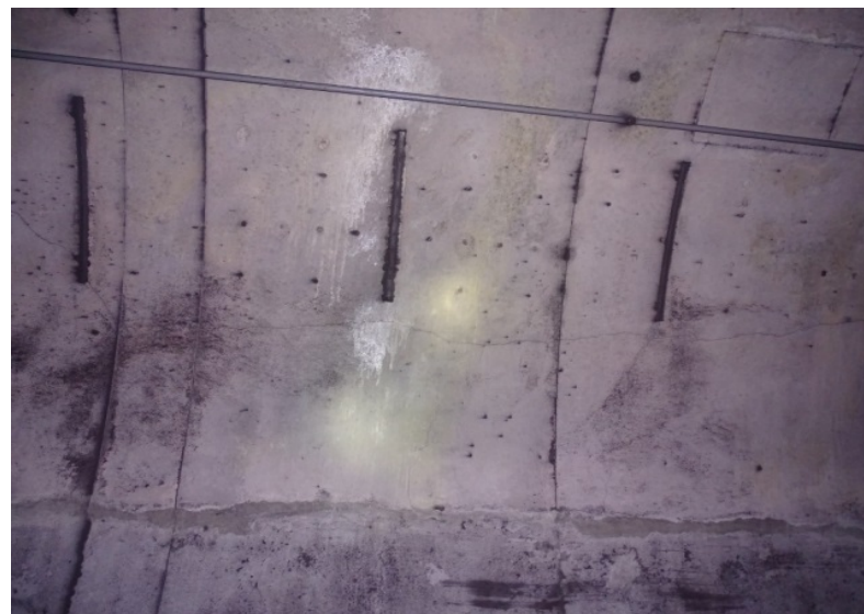
Photograph No. 340 Station 78+18 - transverse crack in east wall.
