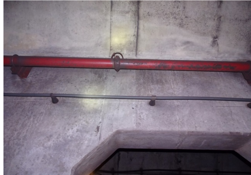
Photograph No. 246 Station 75+95 - vertical crack above west arch.
