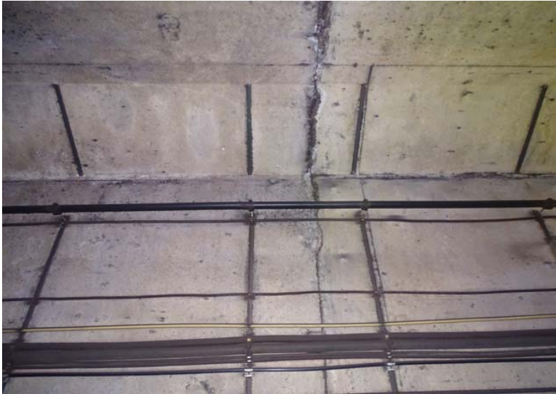
Photograph No. 113 Station 72+60 - crack on the east wall.
