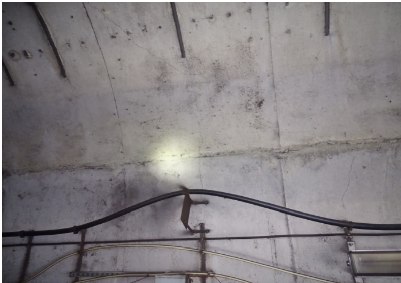
Photograph No. 371 Station 75+27 - vertical crack in upper portion of west wall.
