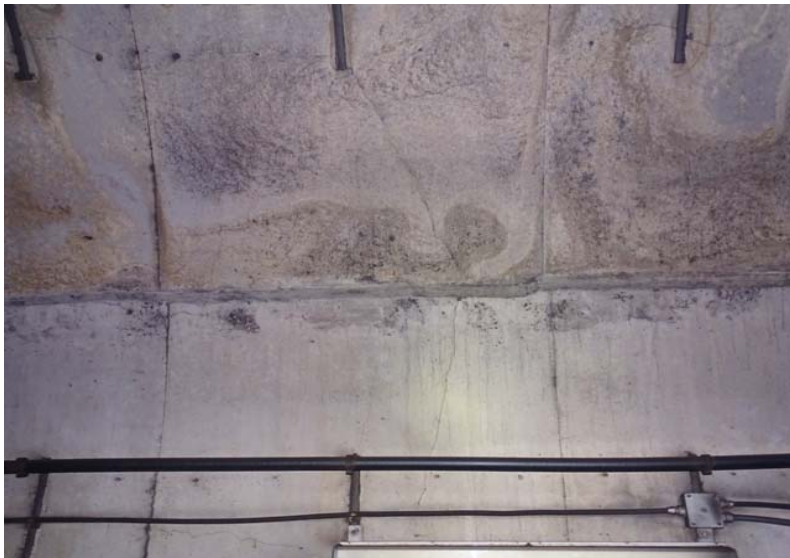
Photograph No. 307 Station 74+40 - crack on west wall.
