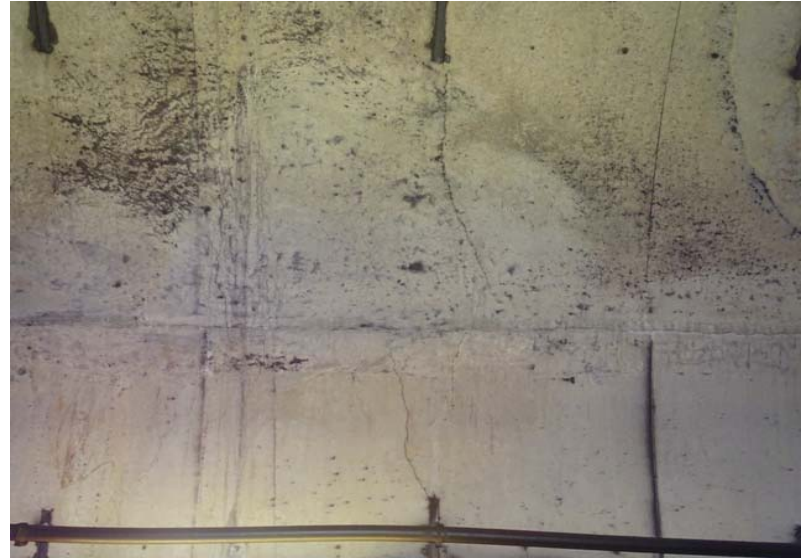
Photograph No. 182 Station 74+40 - cracks on the east wall.
