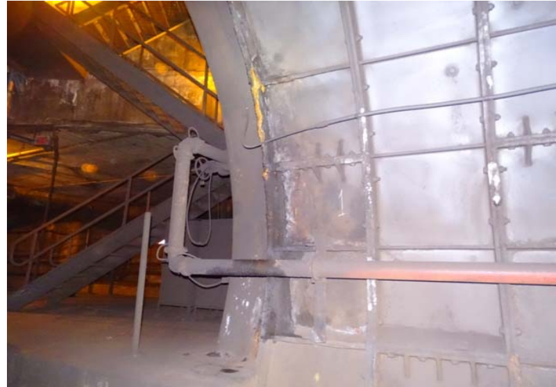
Photograph No. 30 Station 70+20 - stains and corrosion on the west wall.
