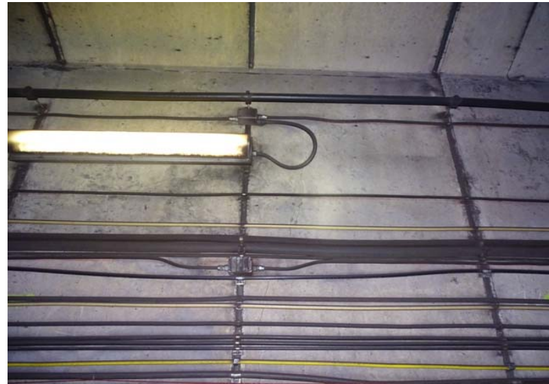
Photograph No. 102 Station 72+40 - crack on the east wall.
