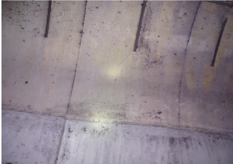
Photograph No. 293 Station 76+90 - vertical crack in east wall.
