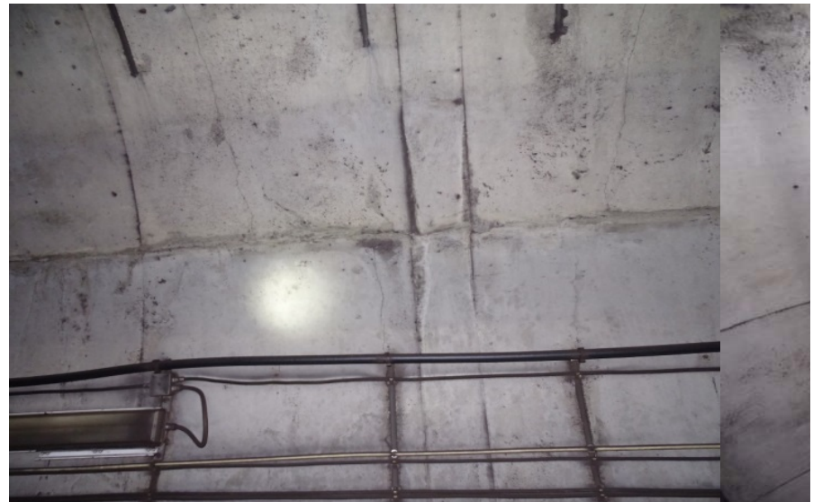
Photograph No. 364 Station 75+15 - crack in upper portion of west wall.
