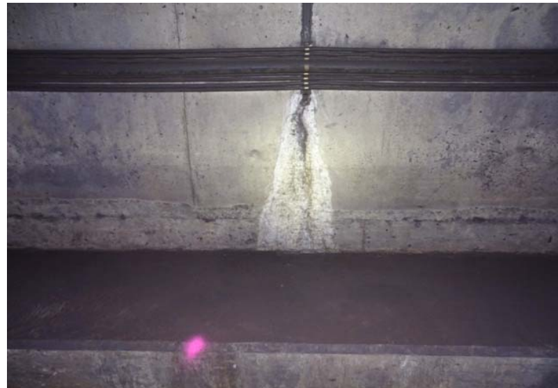
Photograph No. 188 Station 72+60 - crack and efflorescence on west wall.
