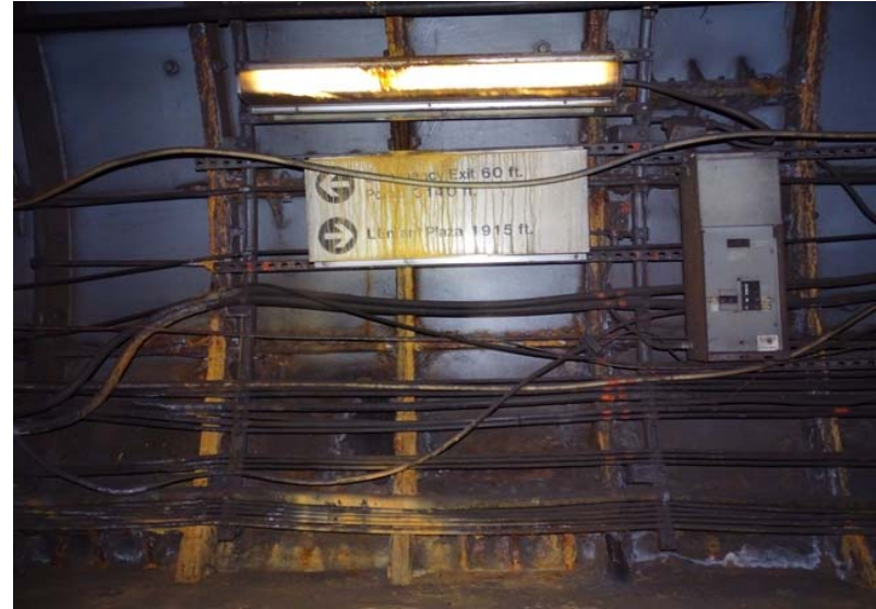
Photograph No. 34 Station 70+30 - stains and corrosion on the west wall.
