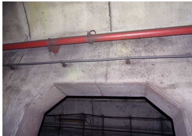
Photograph No. 362 Station 78+70 - vertical cracks above west arch.
