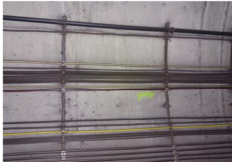
Photograph No. 192 Station 74+60 - crack on the east wall.
