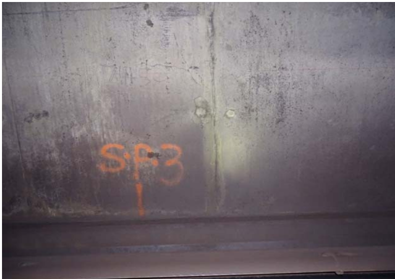
Photograph No. 311 Station 74+50 - crack on east wall.
