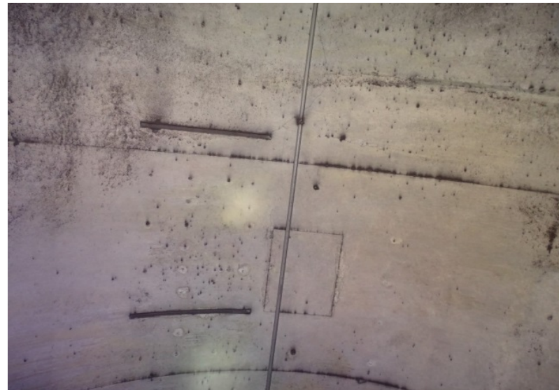
Photograph No. 292 Station 76+82 - transverse crack in ceiling.
