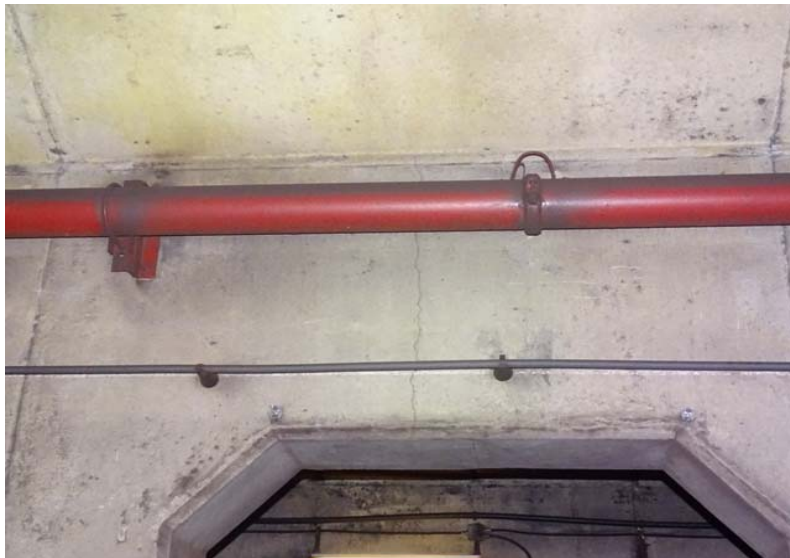
Photograph No. 99 Station 72+20 - crack above west arch.
