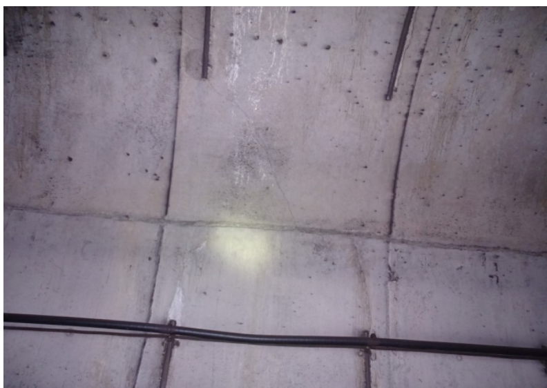
Photograph No. 243 Station 75+87 - vertical crack in east wall.
