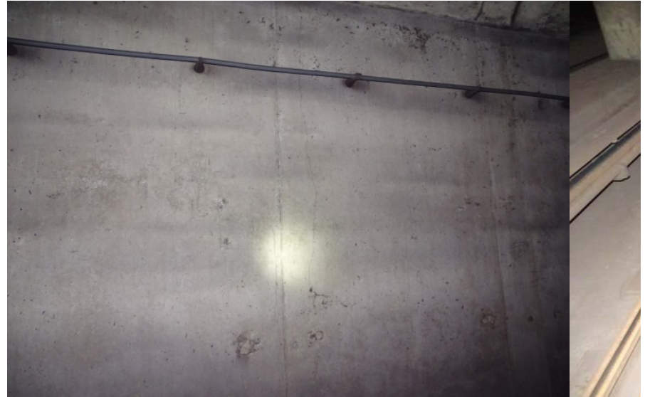
Photograph No. 350 Station 75+07 - vertical crack on east wall.
