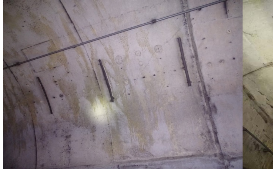
Photograph No. 494 Station 77+00 - diagonal crack in upper portion of east wall.
