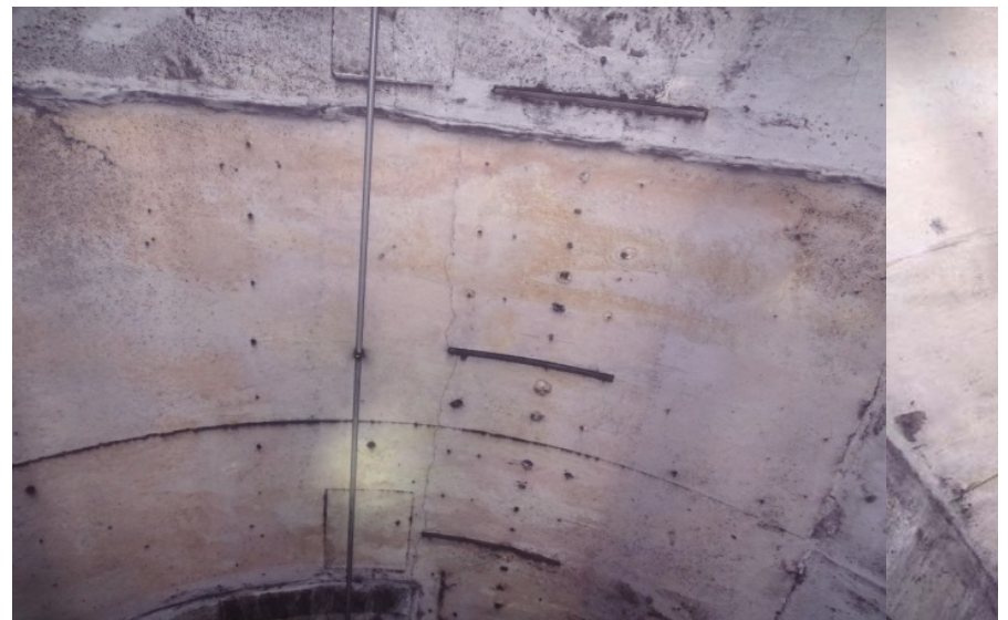
Photograph No. 544 Station 77+90 - transverse crack in ceiling.
