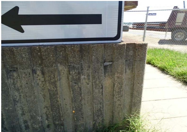
Photograph No. 195 Vent shaft exterior, northwest side, close up of separation.
