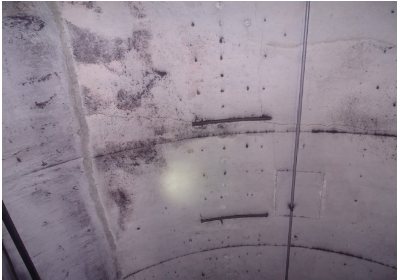
Photograph No. 217 Station 75+20 - crack in ceiling.
