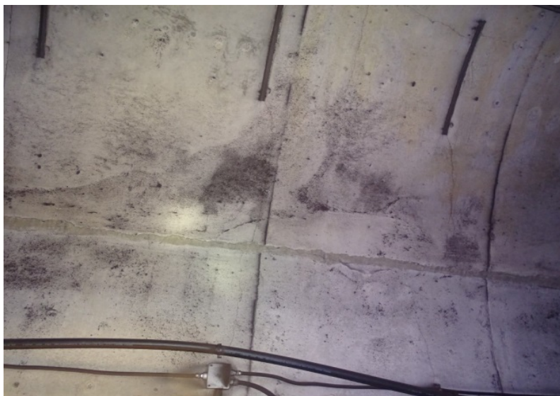
Photograph No. 367 Station 78+82 - vertical crack on east wall.
