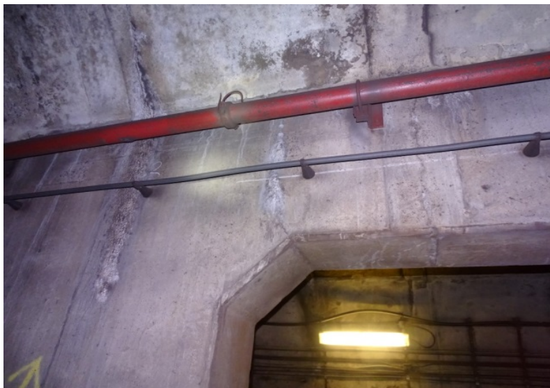
Photograph No. 305 Station 77+21 - vertical crack and efflorescence above west arch.
