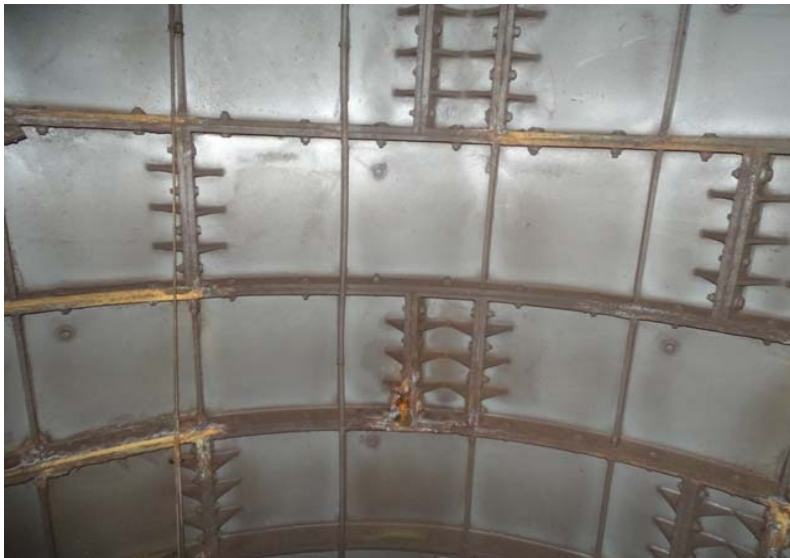
Photograph No. 27 Station 70+20 - corrosion on the ceiling.
