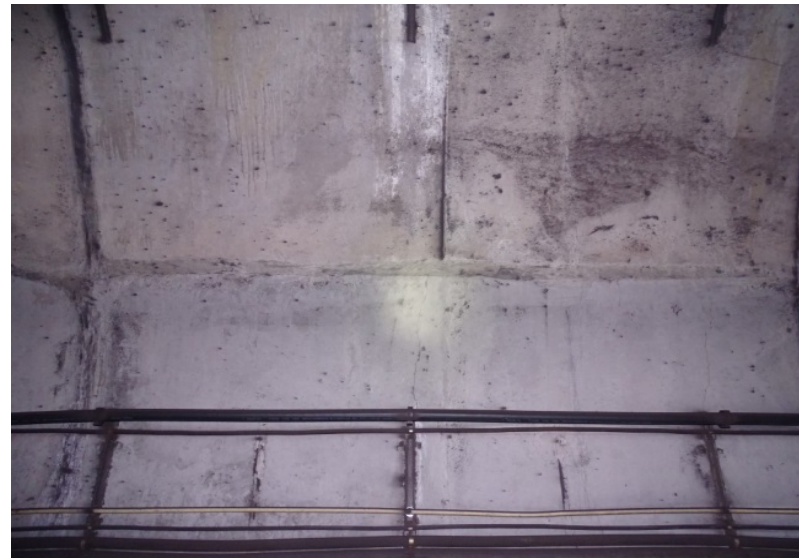
Photograph No. 280 Station 76+61 - crack in east wall.
