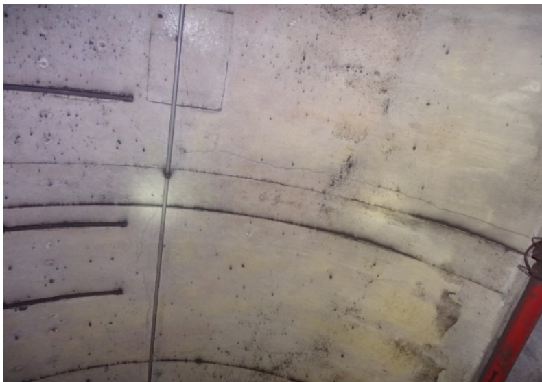
Photograph No. 229 Station 75+55 - transverse crack in ceiling.
