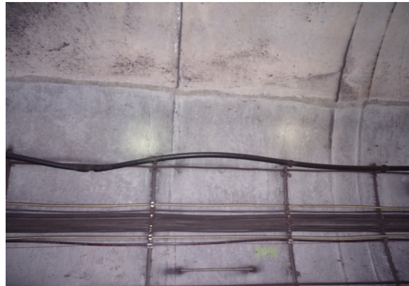
Photograph No. 228 Station 75+50 - vertical crack in east wall.
