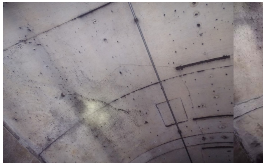
Photograph No. 444 Station 76+28 - crack in ceiling.
