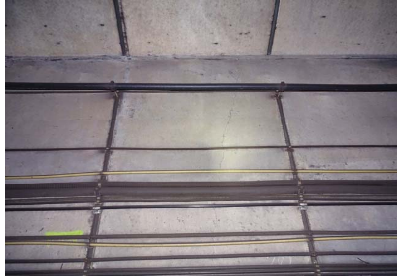
Photograph No. 74 Station 71+80 - crack on the east wall.
