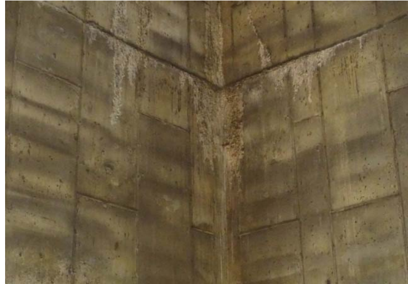
Photograph No. 66 Main room, northeast corner, close up of efflorescence.
