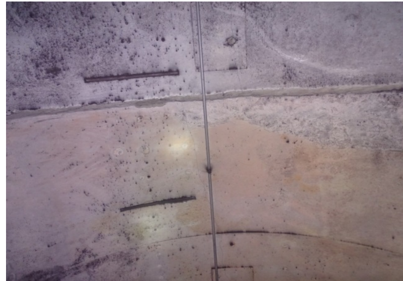
Photograph No. 334 Station 77+90 - crack in ceiling.
