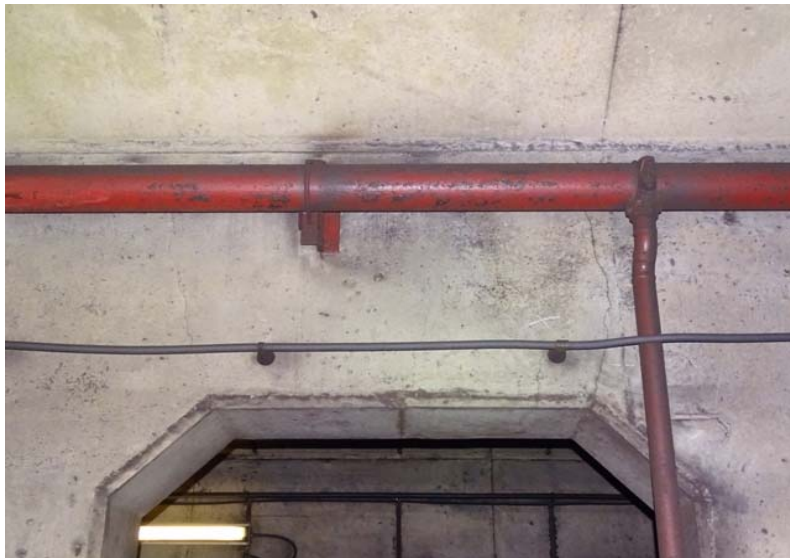
Photograph No. 135 Station 73+00 - cracks above west wall.
