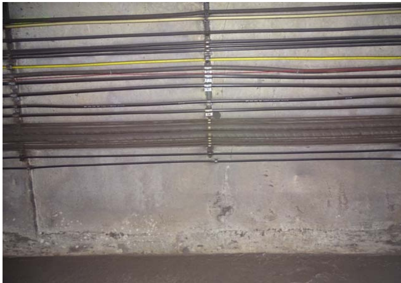
Photograph No. 103 Station 72+40 - crack on the east wall.
