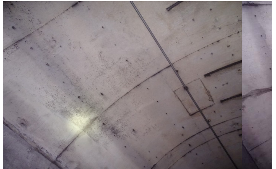
Photograph No. 524 Station 77+53 - crack in ceiling.
