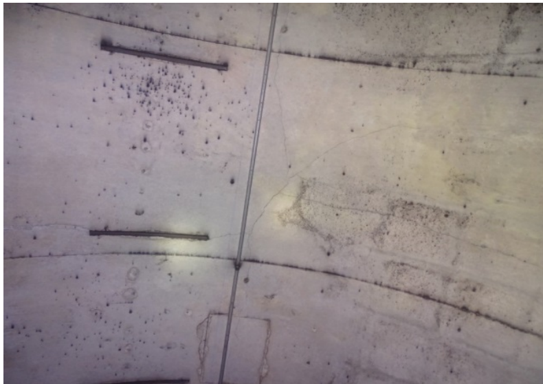
Photograph No. 235 Station 75+66 - cracks in ceiling.
