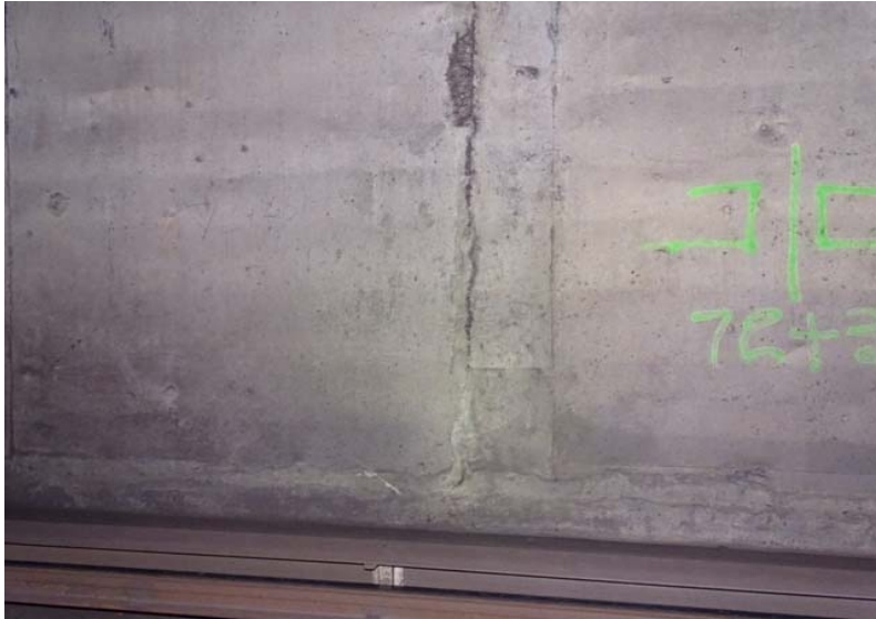
Photograph No. 165 Station 72+30 - crack on east wall.
