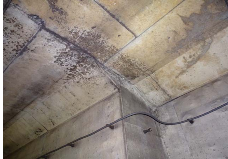
Photograph No. 126 Station 71+80 - stains and efflorescence at the upper portion of the east wall.
