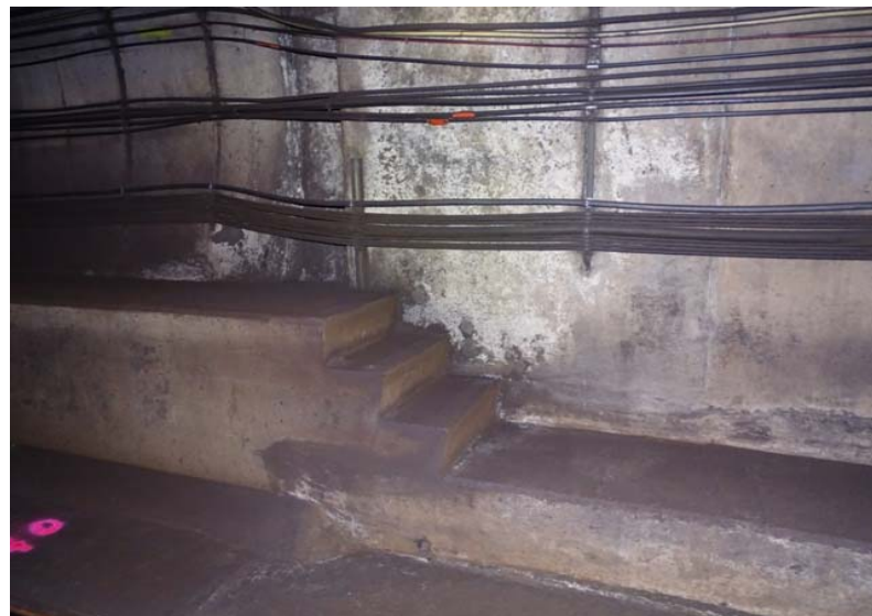
Photograph No. 300 Station 74+30, lower portion of west wall. Note the stains and efflorescence.
