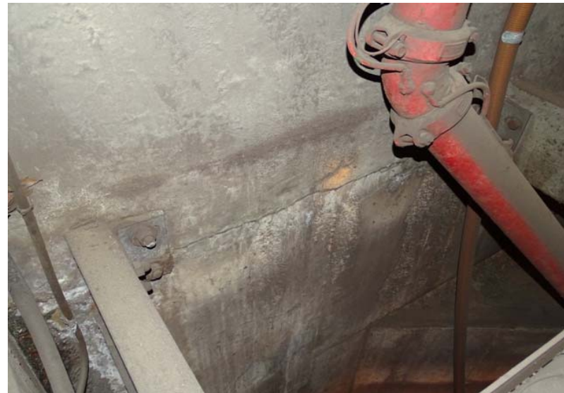
Photograph No. 116 Main room, upper level, north wall, looking down at crack and efflorescence.
