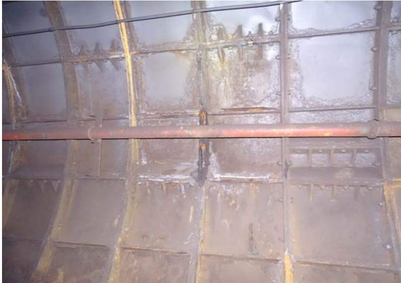
Photograph No. 29 Station 70+20 - active leak and stains on the west wall.
