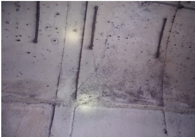
Photograph No. 263 Station 76+37 - vertical crack in east wall.
