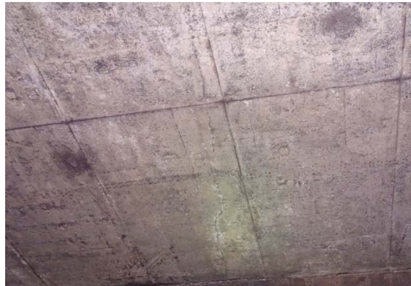
Photograph No. 52 Station 70+60 - crack on the ceiling, looking west.
