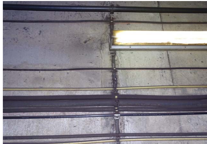
Photograph No. 152 Station 73+60 - cracks on the east wall.
