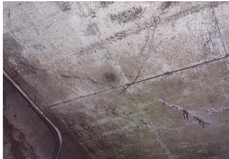
Photograph No. 64 Station 70+80 - cracks on the ceiling.
