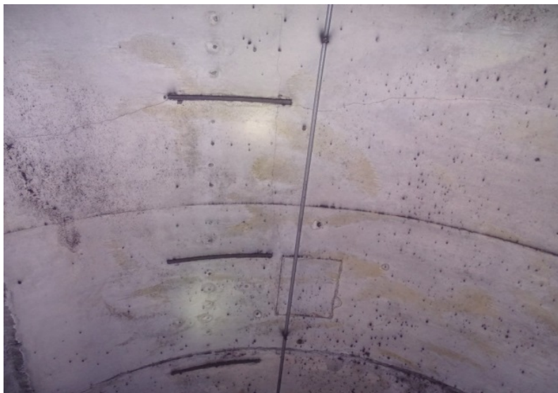
Photograph No. 313 Station 77+30 - transverse crack in ceiling.
