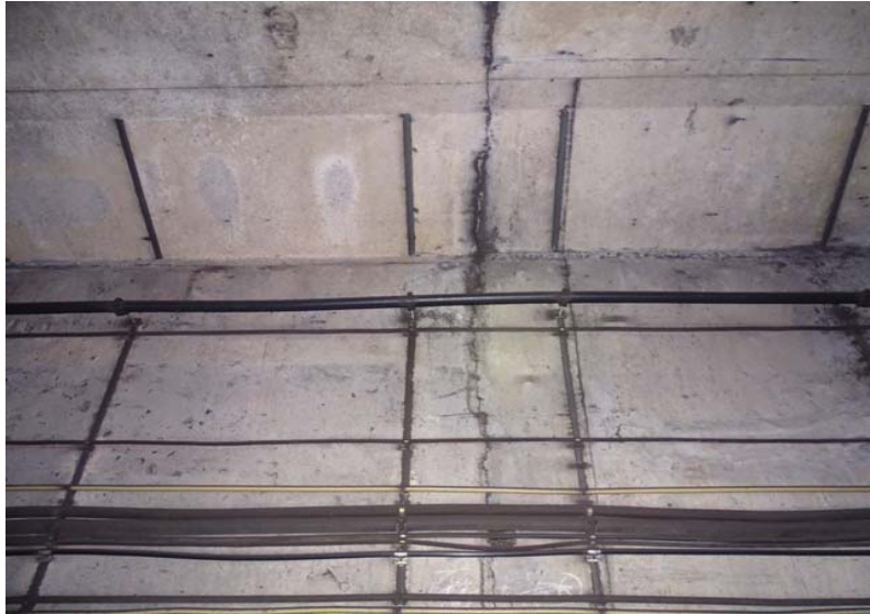
Photograph No. 93 Station 72+20 - crack on the east wall.
