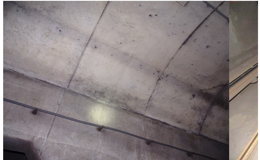
Photograph No. 442 Station 76+22 - vertical crack in east wall.
