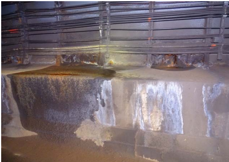
Photograph No. 19 Station 70+00 - active leaks, stains, and efflorescence on the west wall.
