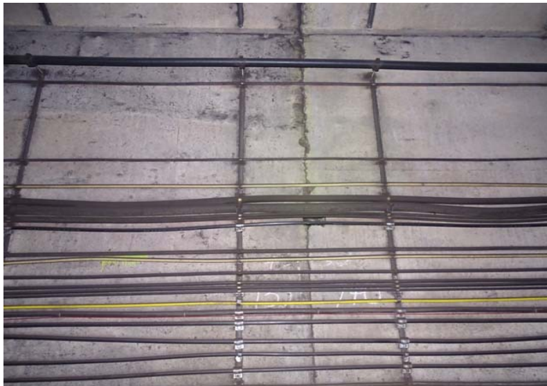
Photograph No. 155 Station 73+60 - damaged concrete at a construction joint on the east wall.
