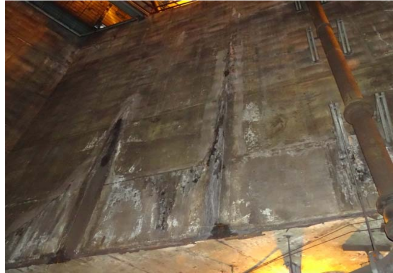
Photograph No. 34 Main room, southwest wall. Note the cracks, stains, and efflorescence.
