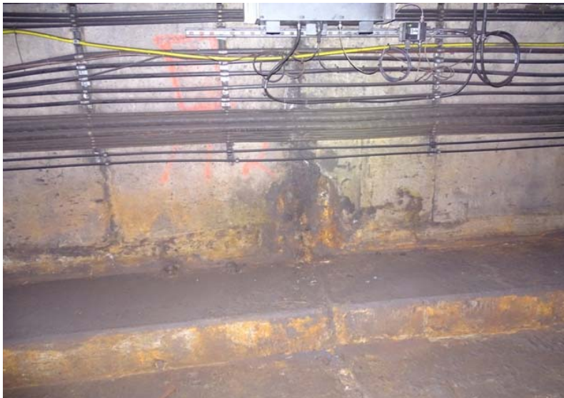
Photograph No. 43 Station 70+80 - stains on the east wall.
