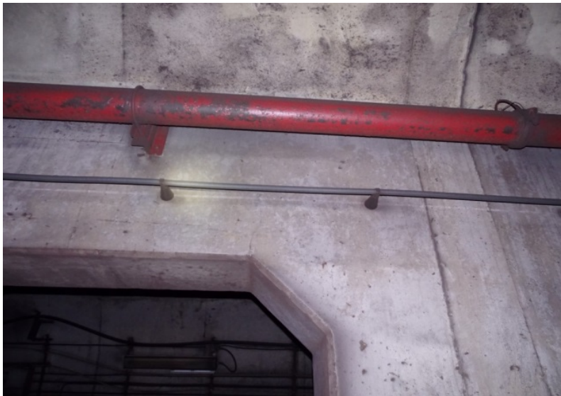
Photograph No. 211 Station 75+15 - crack above west arch.
