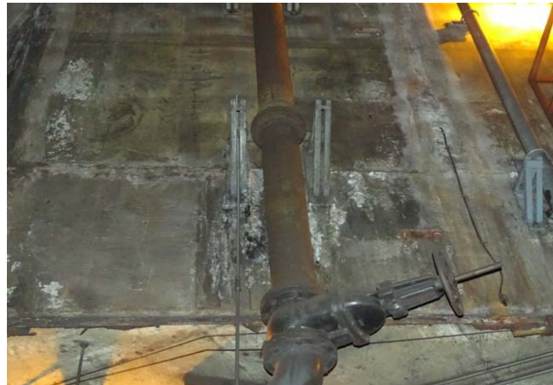
Photograph No. 36 Main room, southwest wall. Close up of the stains and efflorescence.
