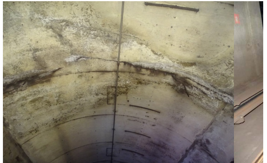
Photograph No. 504 Station 77+20, ceiling. Note cracks and stalagmites.
