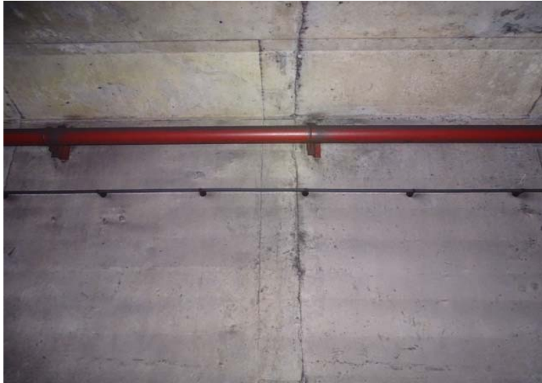
Photograph No. 97 Station 72+20 - crack on the west wall.
