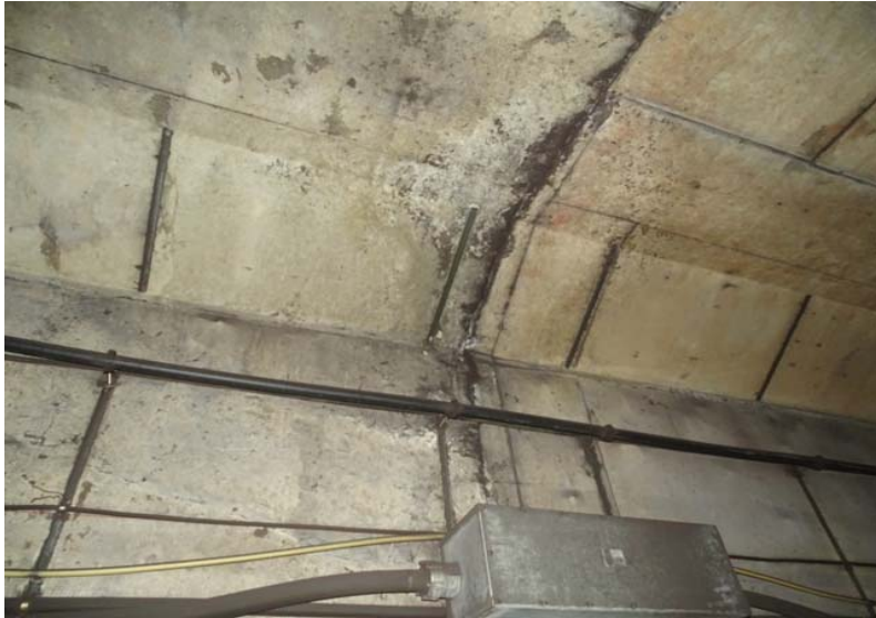
Photograph No. 65 Station 71+60 - stains on the east wall.
