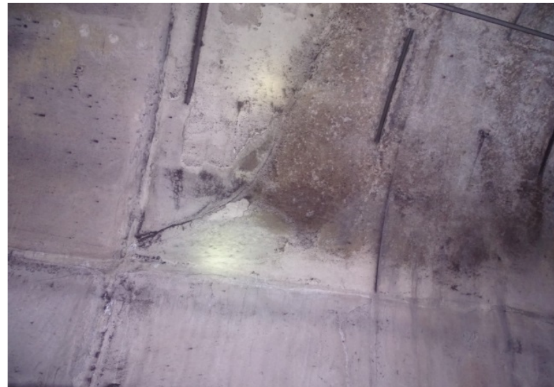
Photograph No. 300 Station 77+00 - crack in east wall.
