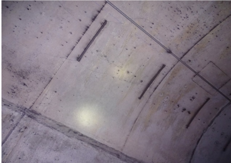
Photograph No. 253 Station 76+05 - crack in ceiling.
