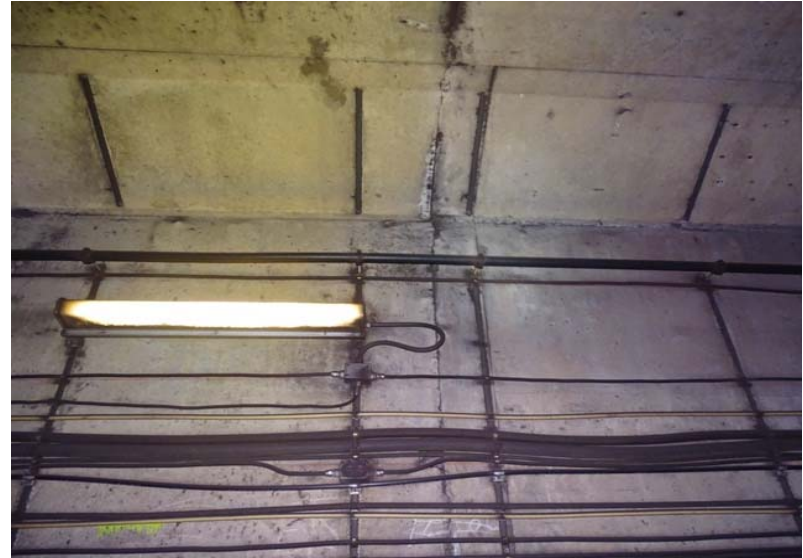
Photograph No. 138 Station 73+20 - crack and stains on the east wall.
