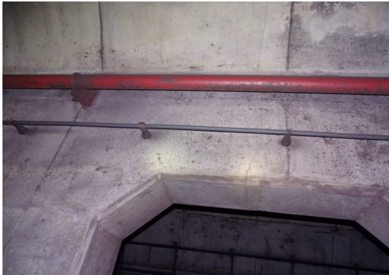
Photograph No. 345 Station 78+20 - vertical crack above west arch.
