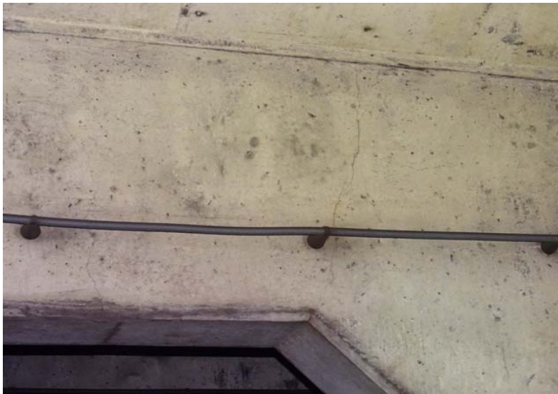
Photograph No. 219 Station 73+10 - cracks above east arch.
