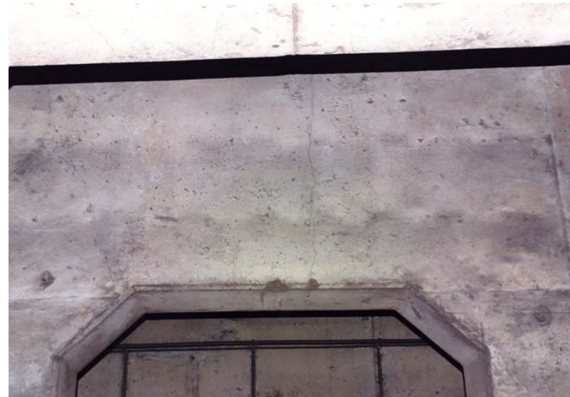
Photograph No. 16 Storage area, section 2, upper middle portion. Note the cracks.
