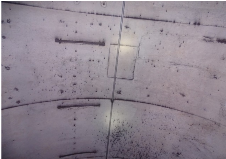
Photograph No. 259 Station 76+22 - crack in ceiling.
