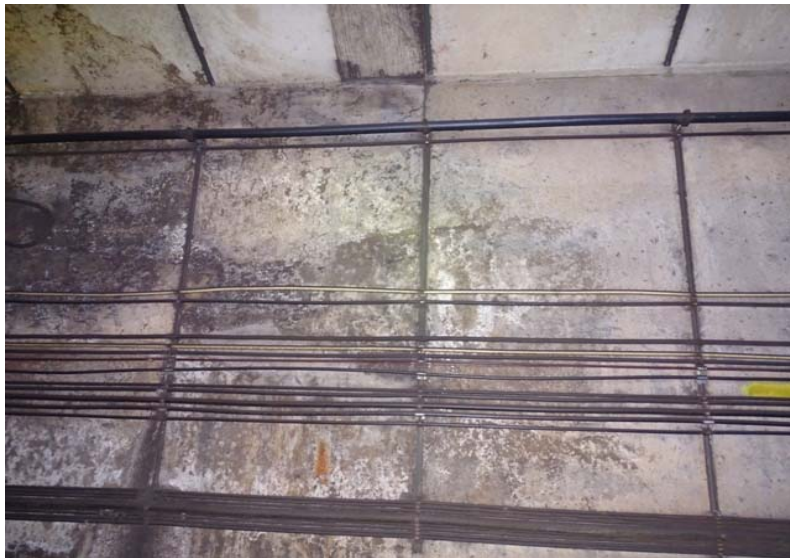
Photograph No. 111 Station 71+50, upper portion of west wall. Note the stains.
