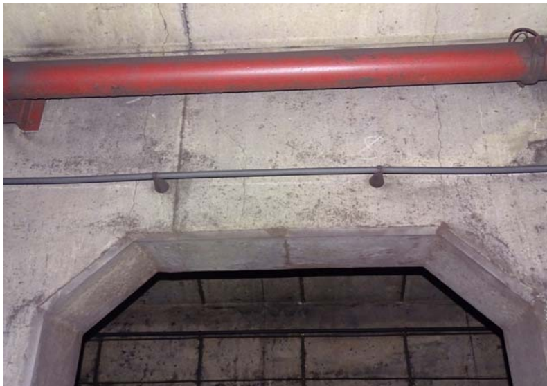
Photograph No. 171 Station 74+00 - cracks above west arch.
