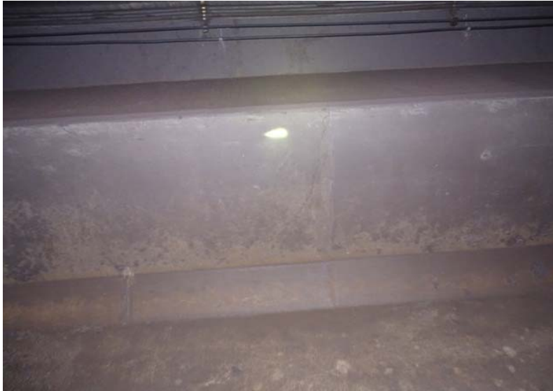
Photograph No. 193 Station 74+60 - crack on the catwalk.
