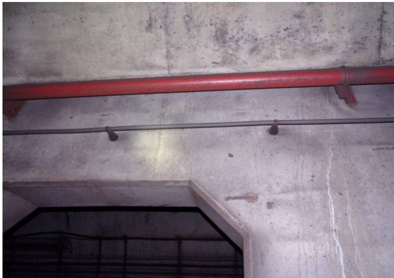
Photograph No. 283 Station 76+61 - crack above west arch.
