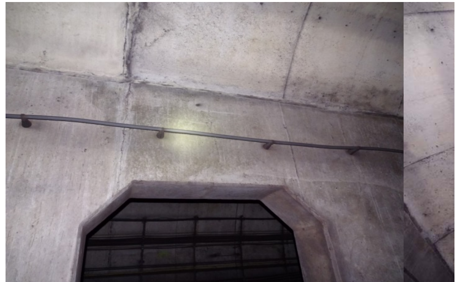
Photograph No. 436 Station 76+15 - three vertical cracks in east wall.
