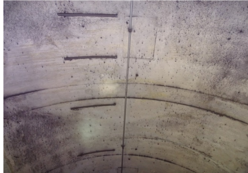
Photograph No. 286 Station 76+75 - typical transverse crack in ceiling.
