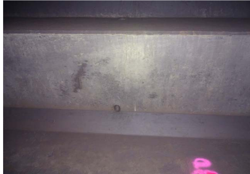
Photograph No. 338 Station 74+80 - crack on catwalk.
