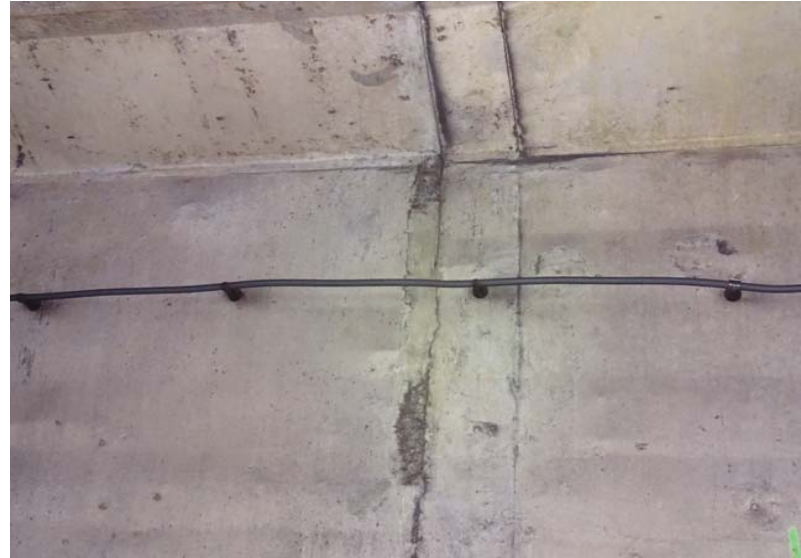
Photograph No. 166 Station 72+30 - damaged concrete on east wall.
