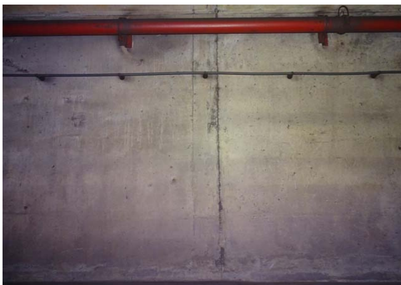
Photograph No. 143 Station 73+20 - crack and stains on the west wall.
