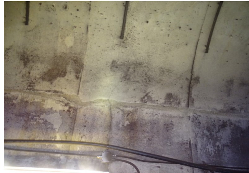
Photograph No. 352 Station 78+43 - vertical crack in east wall.
