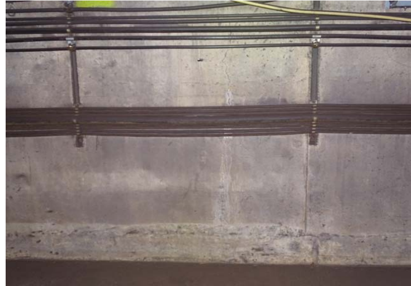
Photograph No. 146 Station 72+00 - crack and efflorescence on west wall.
