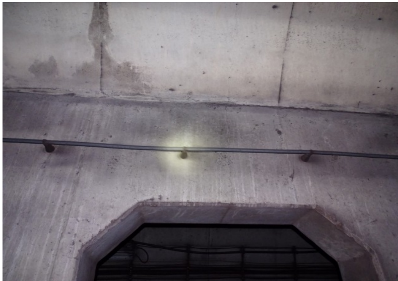
Photograph No. 531 Station 77+67 - vertical crack above east arch.
