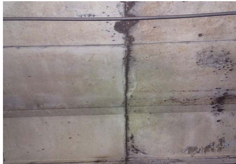
Photograph No. 160 Station 73+60 - damaged concrete on the ceiling, looking west.
