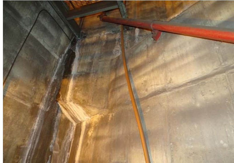
Photograph No. 78 Main room, northwest corner. Note the efflorescence.
