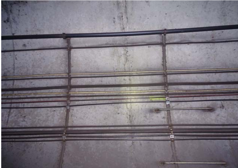
Photograph No. 345 Station 74+90 - crack on west wall.
