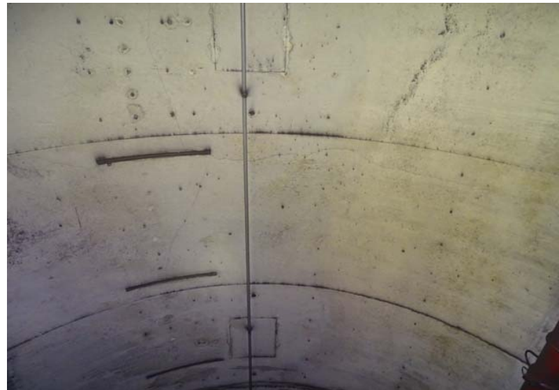
Photograph No. 200 Station 74+80 - cracks on the ceiling.
