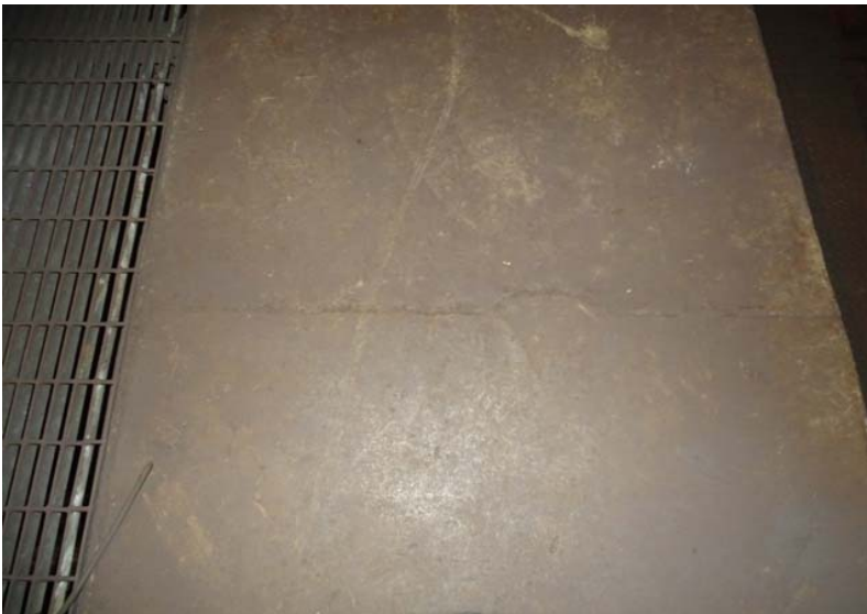
Photograph No. 47 Platform. Close up of condition of concrete.
