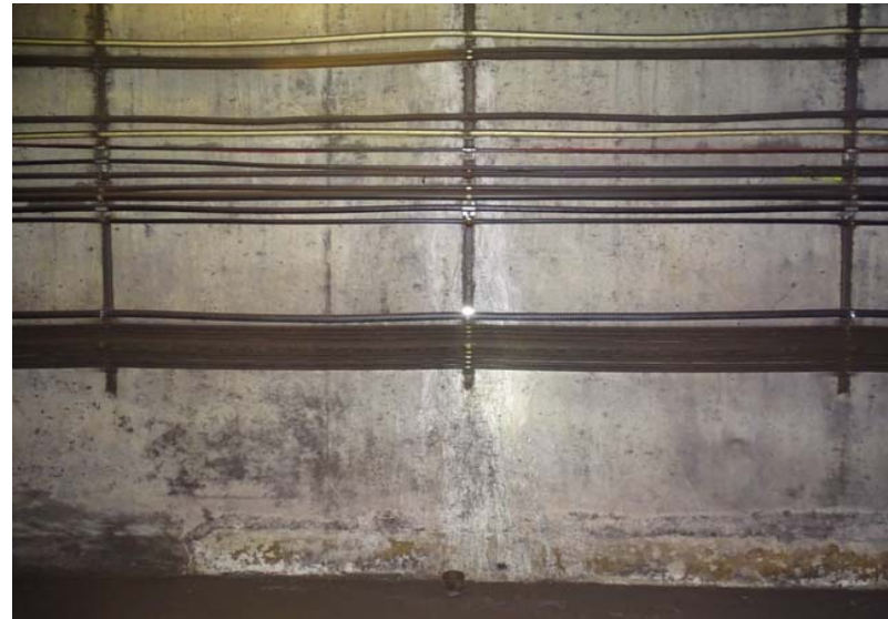
Photograph No. 250 Station 73+50 - efflorescence on west wall.
