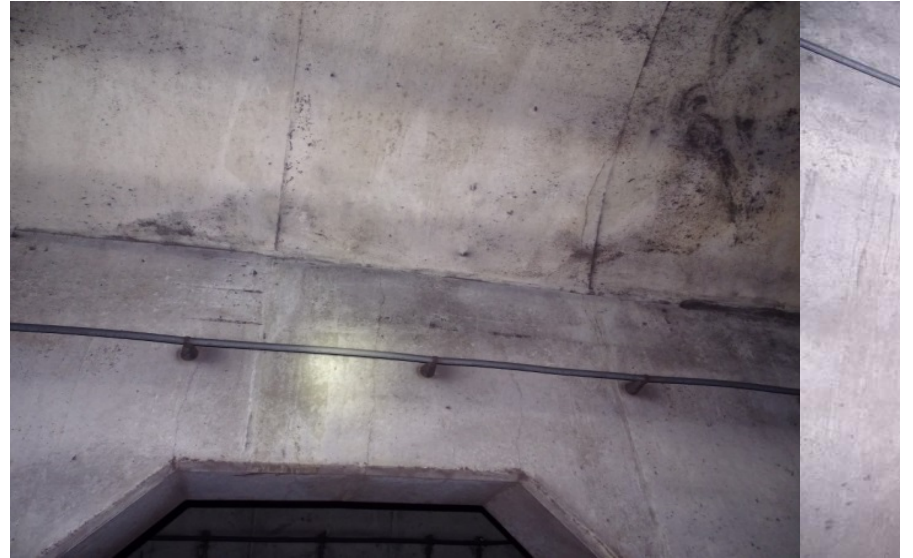
Photograph No. 474 Station 76+70 - vertical crack in east wall.
