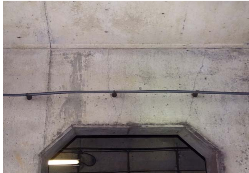
Photograph No. 204 Station 72+90 - cracks above east arch.
