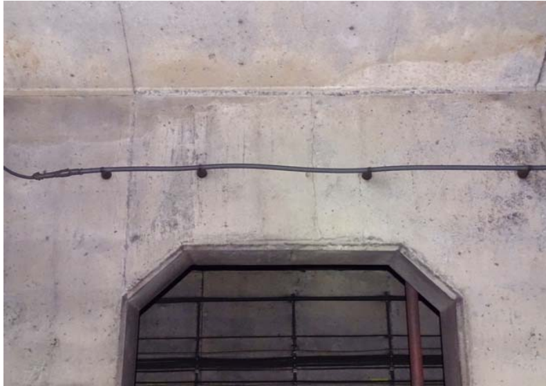
Photograph No. 133 Station 71+90 - cracks above east arch.
