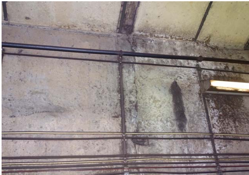
Photograph No. 97 Station 71+30 - crack and stains on the west wall.
