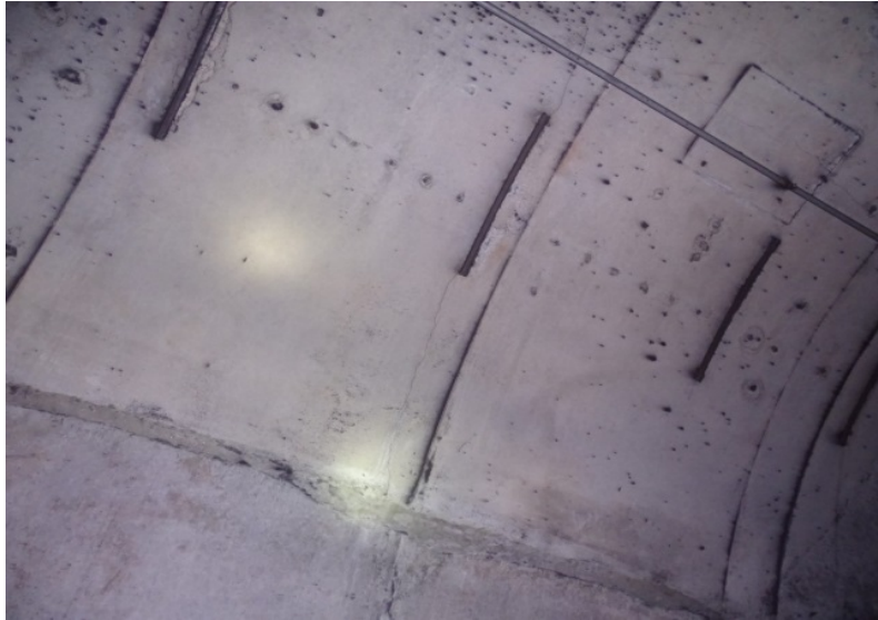
Photograph No. 261 Station 76+30 - vertical crack in east wall.
