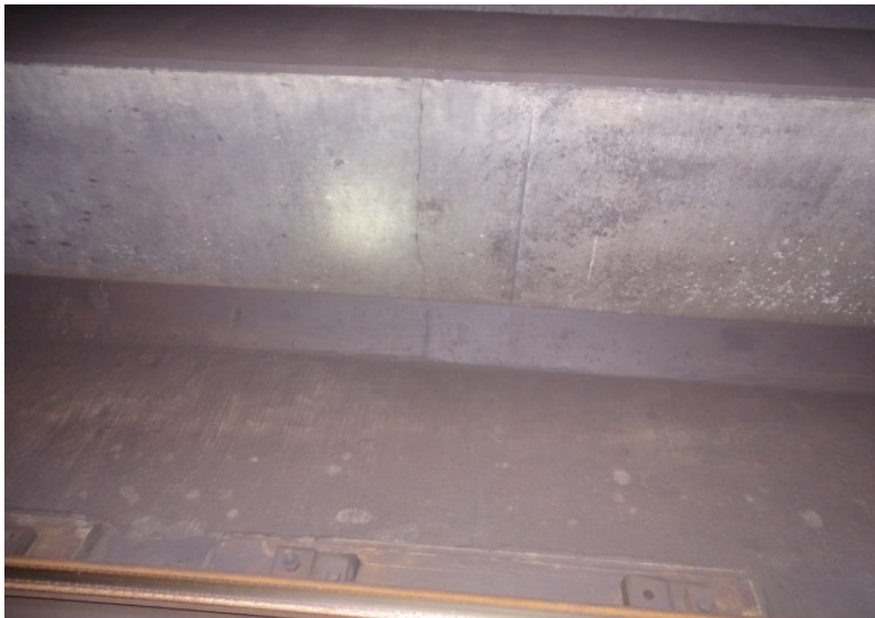
Photograph No. 467 Station 76+60 - crack in safety walkway.
