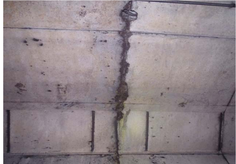
Photograph No. 154 Station 73+60 - damaged concrete on the ceiling, looking east.
