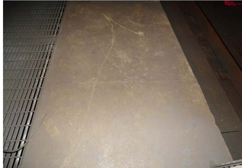
Photograph No. 46 Platform. Close up of condition of concrete.
