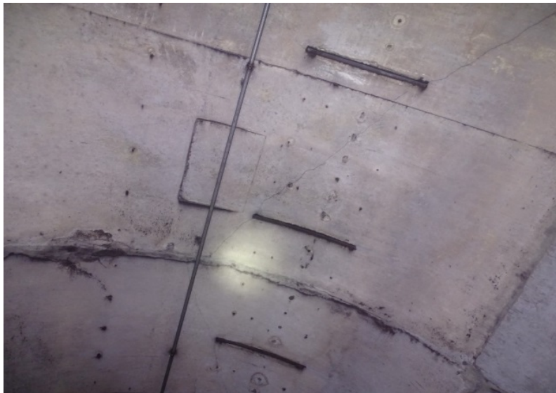
Photograph No. 435 Station 76+15 - crack in ceiling.
