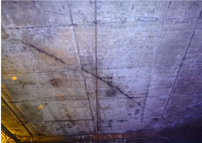
Photograph No. 57 Station 70+70, ceiling. Note the crack.
