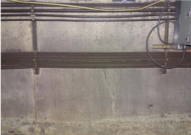
Photograph No. 145 Station 72+00 - crack on west wall.
