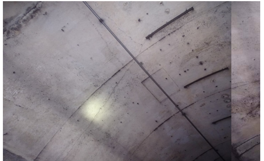
Photograph No. 468 Station 76+65 - crack in ceiling.
