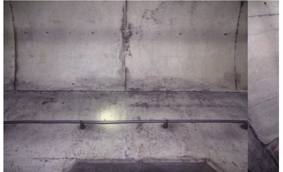
Photograph No. 550 Station 78+20 - vertical crack above east arch.
