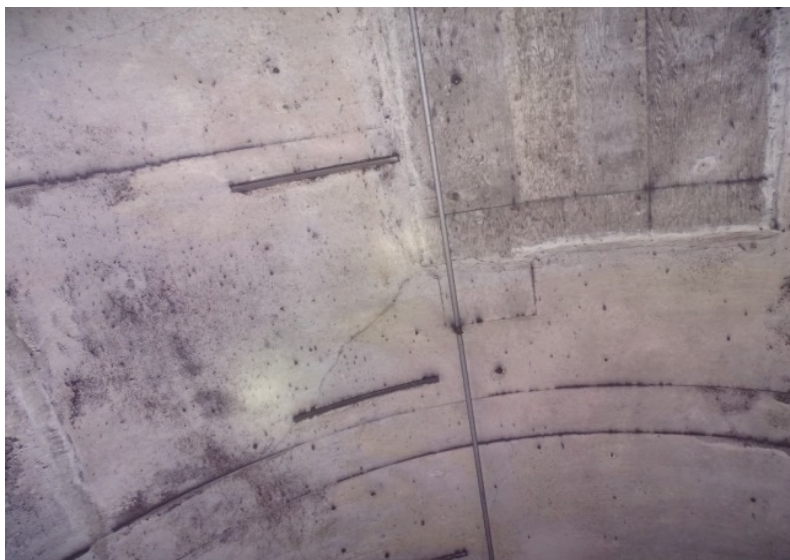
Photograph No. 339 Station 78+12 - crack in ceiling.
