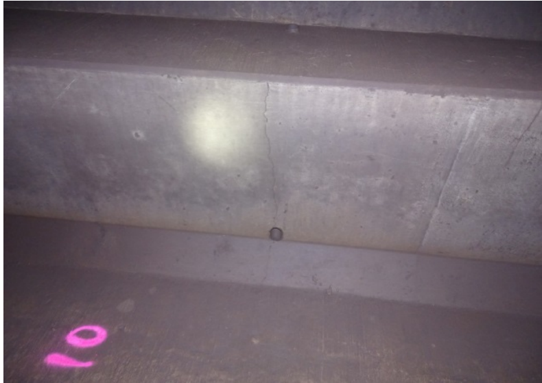
Photograph No. 429 Station 76+08 - crack in west safety walkway.
