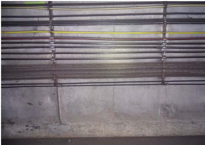
Photograph No. 75 Station 71+80 - crack on the east wall.
