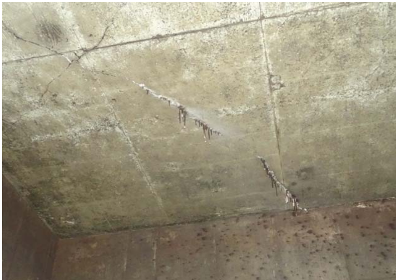
Photograph No. 63 Station 70+80 - crack and efflorescence on the ceiling.
