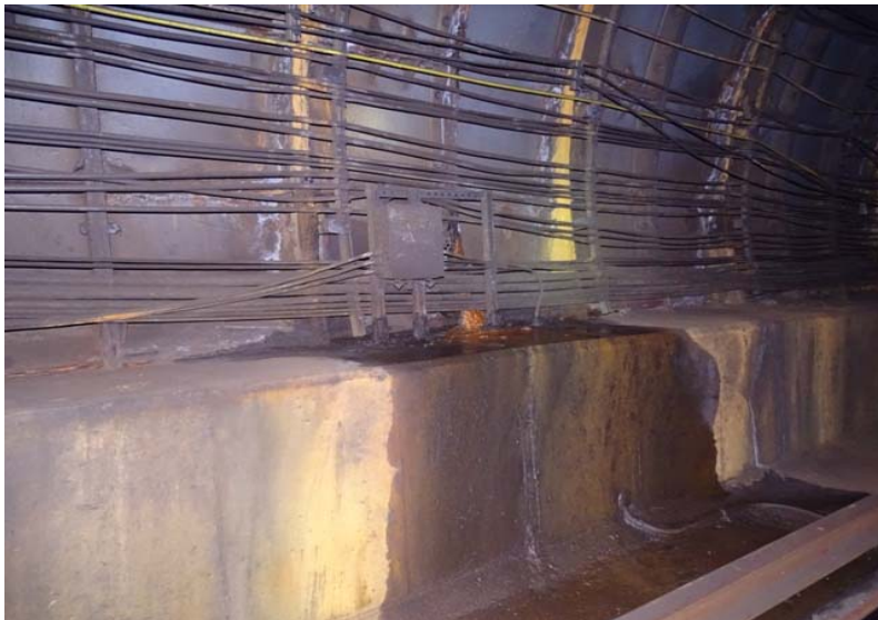
Photograph No. 11 Station 69+80 - active leak on the east wall.
