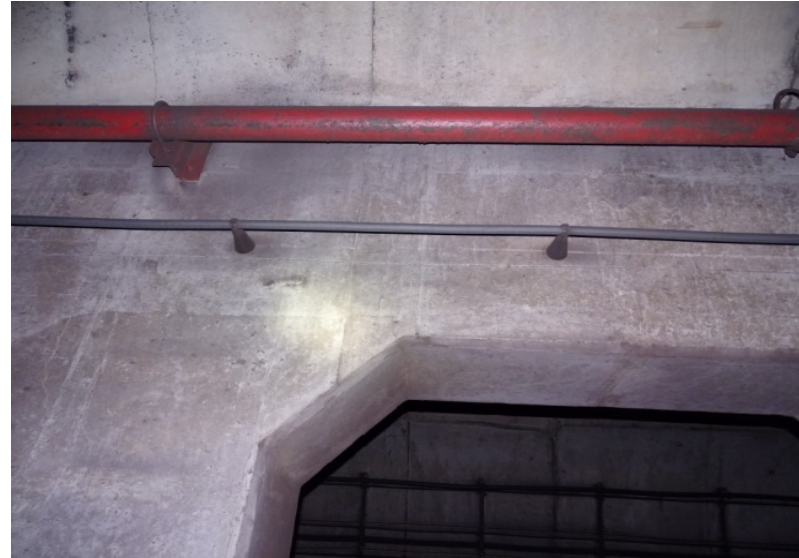
Photograph No. 258 Station 76+22, crack above west arch.
