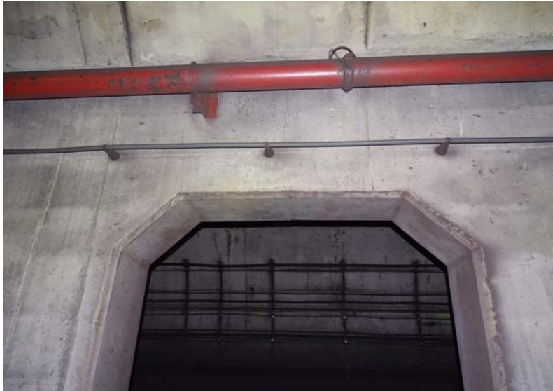
Photograph No. 189 Station 74+40 - cracks above west arch.
