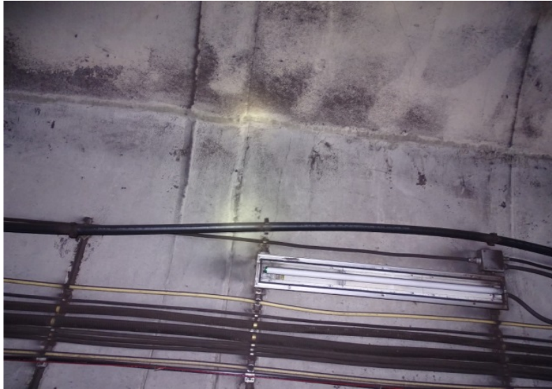
Photograph No. 325 Station 77+61 - vertical crack in ceiling.
