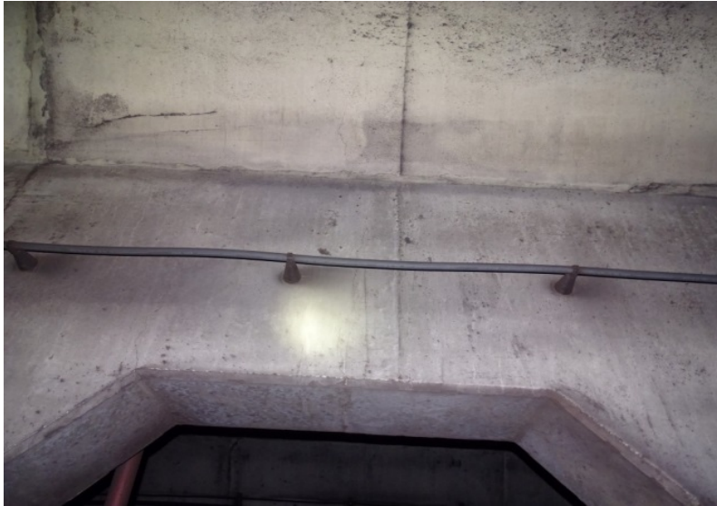
Photograph No. 517 Station 77+40 - vertical crack above east arch.
