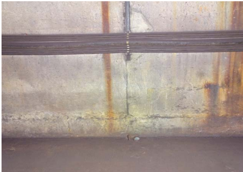
Photograph No. 91 Station 71+20 - previous concrete repair and cracks on west wall.
