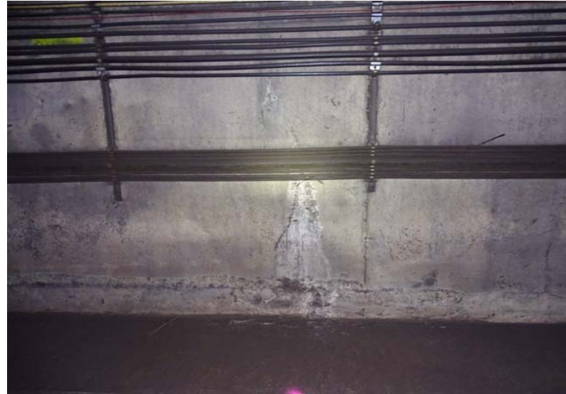
Photograph No. 182 Station 72+50 - crack on west wall.
