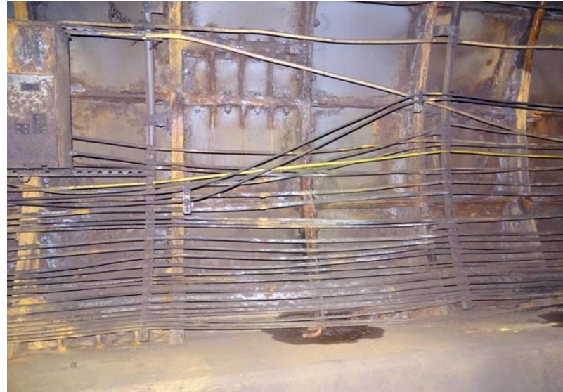
Photograph No. 18 Station 70+00 - active leak and corrosion on the east wall.
