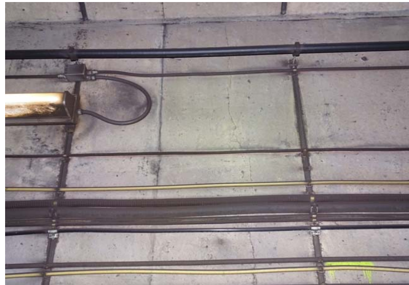
Photograph No. 84 Station 72+00 - crack on the east wall.
