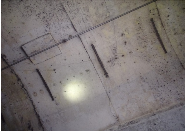
Photograph No. 405 Station 75+75 - crack in ceiling.
