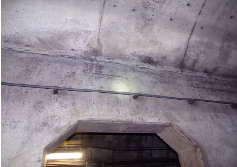
Photograph No. 557 Station 78+40 - vertical crack in east wall.
