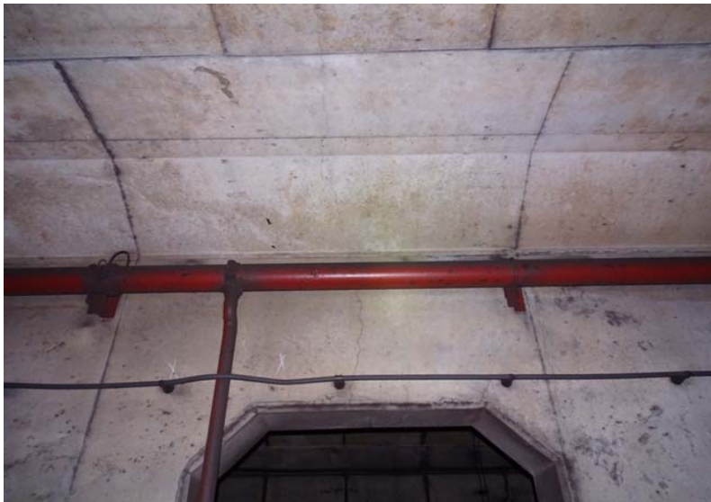
Photograph No. 79 Station 71+80 - crack above west arch.
