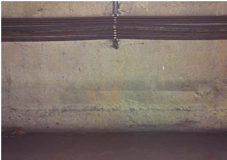
Photograph No. 83 Station 71+10 - crack on the west wall.
