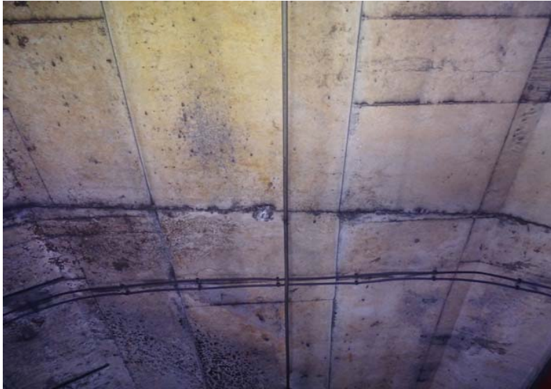
Photograph No. 45 Station 70+80 - stains at a construction joint on the ceiling.
