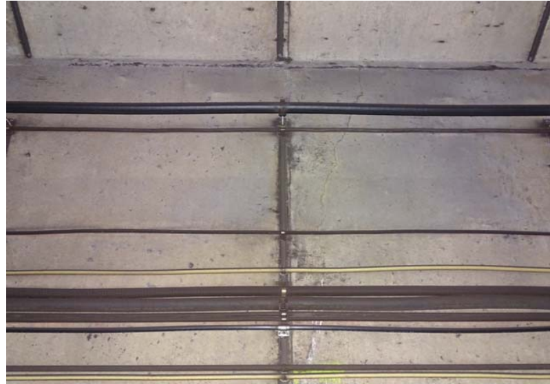
Photograph No. 122 Station 72+80 - crack on the east wall.
