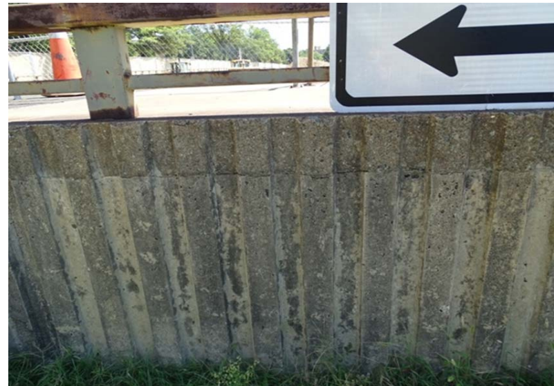
Photograph No. 196 Vent shaft exterior, northwest side, close up of separation.
