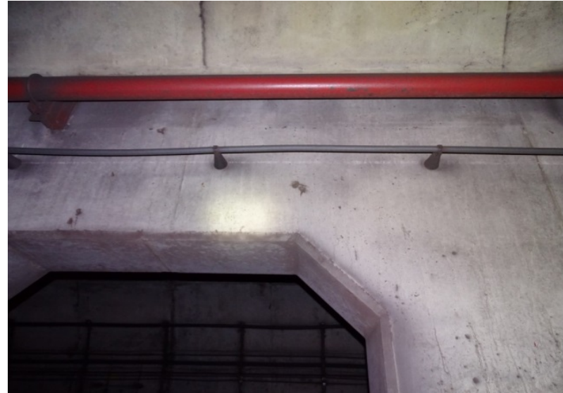
Photograph No. 294 Station 76+91 - vertical crack above west arch.
