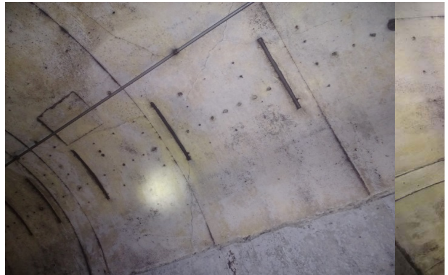
Photograph No. 384 Station 75+49 - crack in ceiling.
