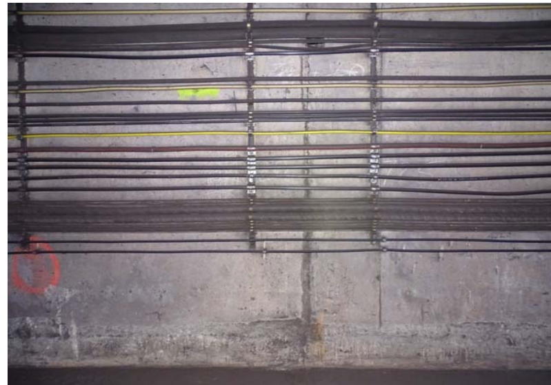
Photograph No. 92 Station 72+20 - crack on the east wall.
