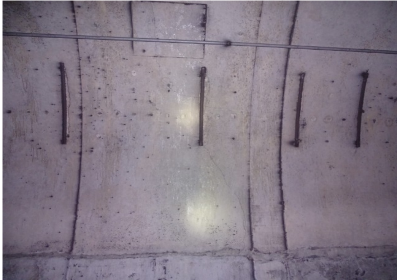
Photograph No. 245 Station 75+95 - crack in ceiling.
