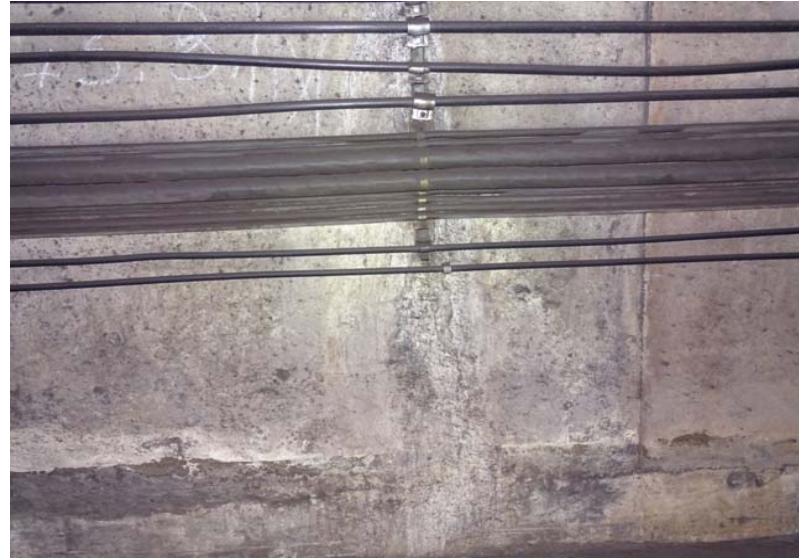
Photograph No. 174 Station 74+20 - crack and stains on the east wall.
