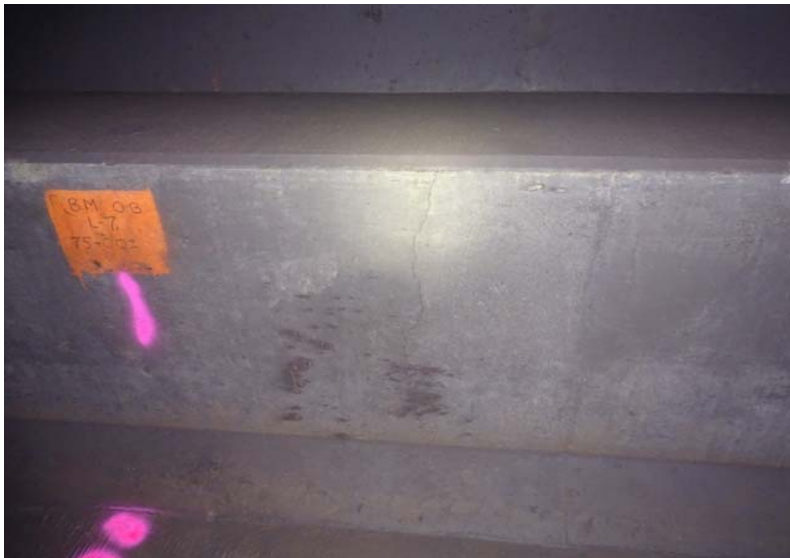
Photograph No. 347 Station 74+90 - crack on catwalk.
