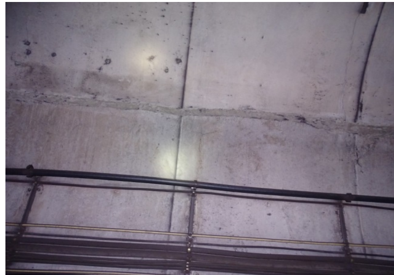
Photograph No. 260 Station 76+25 - vertical crack in east wall.
