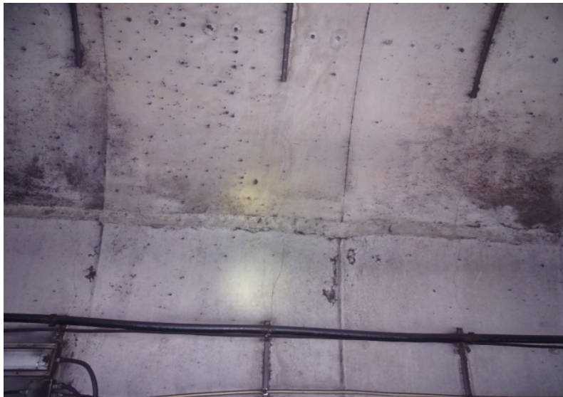
Photograph No. 271 Station 76+45 - vertical crack in east wall.
