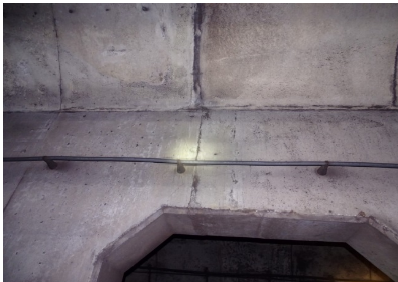
Photograph No. 543 Station 77+90 - vertical crack in east arch.
