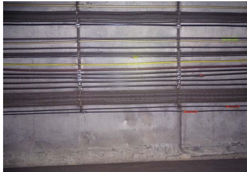
Photograph No. 76 Station 71+80 - cracks on the east wall.
