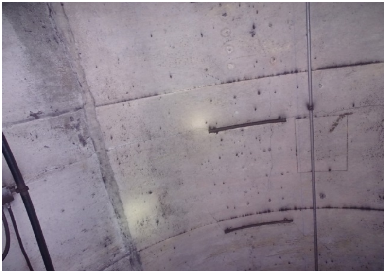
Photograph No. 251 Station 76+02 - transverse crack in ceiling.
