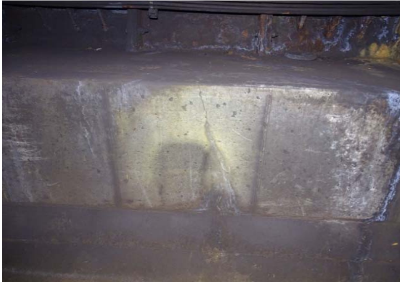
Photograph No. 5 Station 69+70 - crack in the concrete catwalk.
