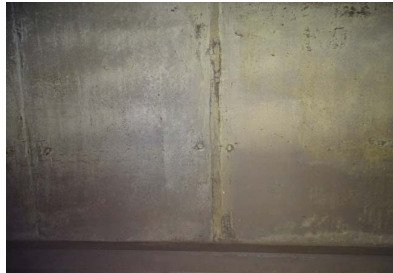
Photograph No. 188 Station 74+40 - previous repair at the joint.
