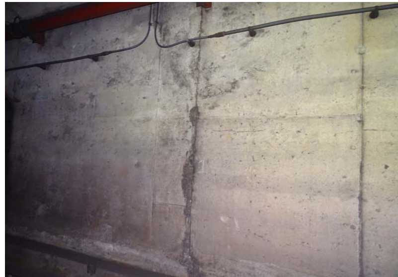
Photograph No. 48 Station 70+80 - damaged concrete at the west wall.
