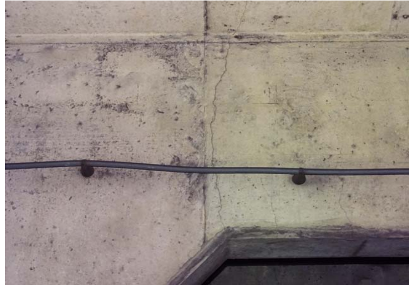
Photograph No. 218 Station 73+10 - cracks above east arch.
