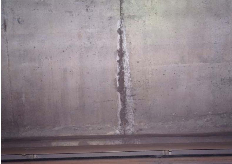
Photograph No. 161 Station 73+60 - stains and efflorescence on the west wall.
