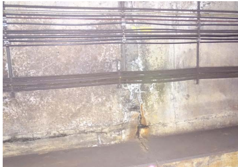
Photograph No. 98 Station 71+30 - crack and stains on the west wall.
