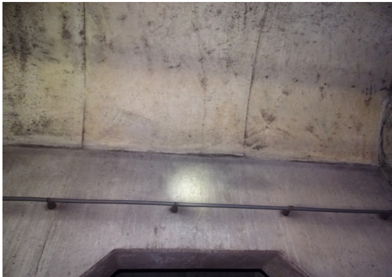
Photograph No. 403 Station 75+70 - vertical crack in east wall.
