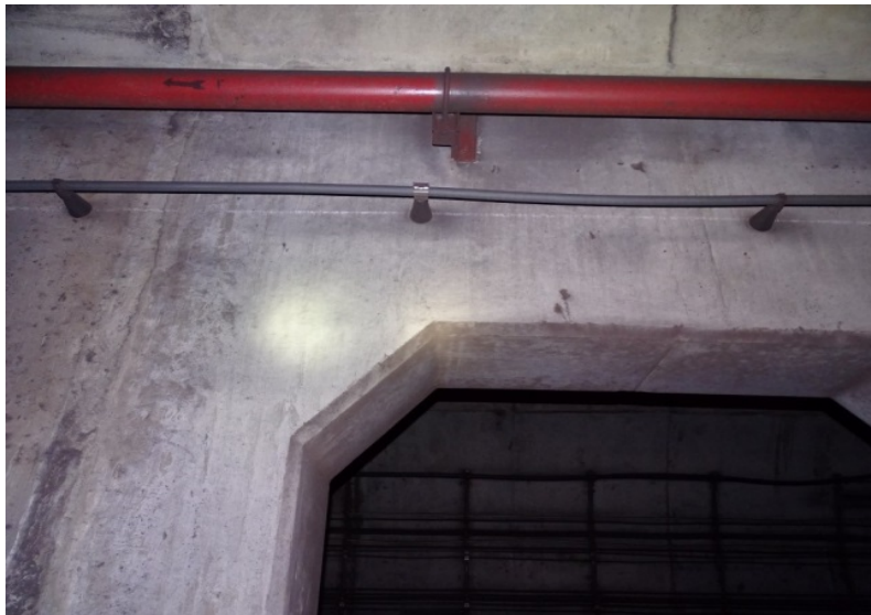
Photograph No. 295 Station 76+95 - vertical crack above west arch.
