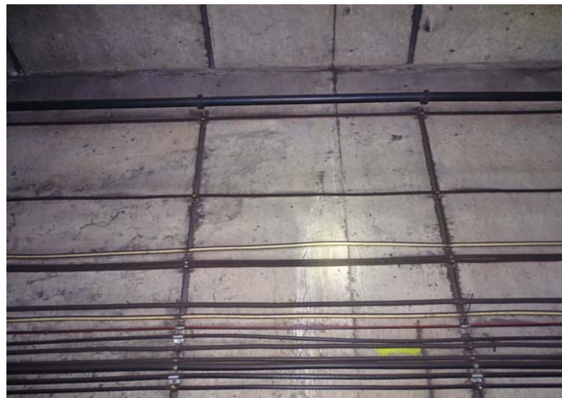
Photograph No. 286 Station 74+10 - crack and efflorescence on west wall.
