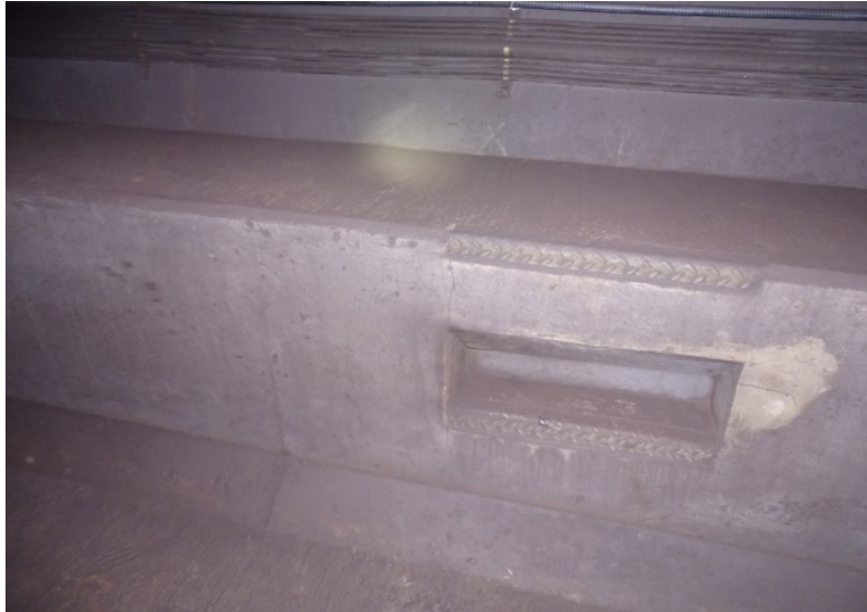
Photograph No. 537 Station 77+70 - crack in west walkway.
