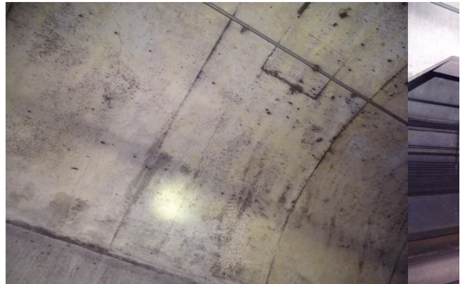
Photograph No. 396 Station 75+60 - crack in east portion of ceiling.
