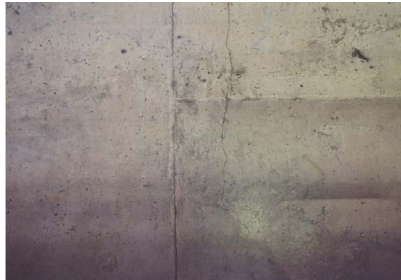
Photograph No. 108 Station 71+50 - crack on the east wall.
