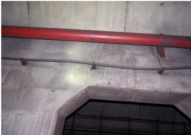
Photograph No. 227 Station 75+45 - crack above west arch.
