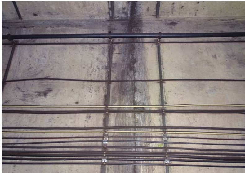
Photograph No. 231 Station 73+20 - stains and efflorescence on west wall.
