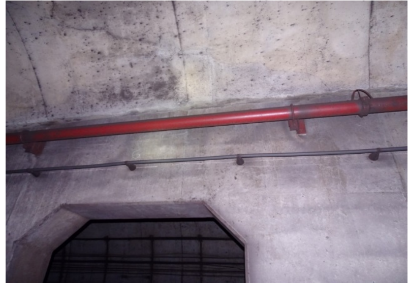
Photograph No. 270 Station 76+41 - crack above west arch.
