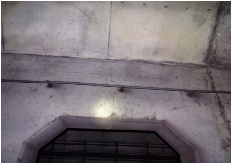
Photograph No. 487 Station 76+95 - vertical crack above east arch.
