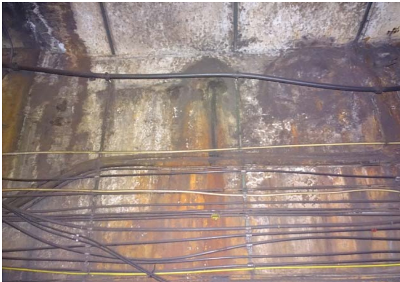
Photograph No. 39 Station 70+80 - stains on the east wall.
