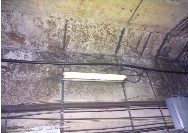
Photograph No. 41 Station 70+80 - stains on the east wall.
