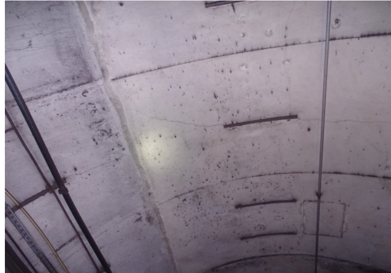
Photograph No. 218 Station 75+25 - crack in ceiling.
