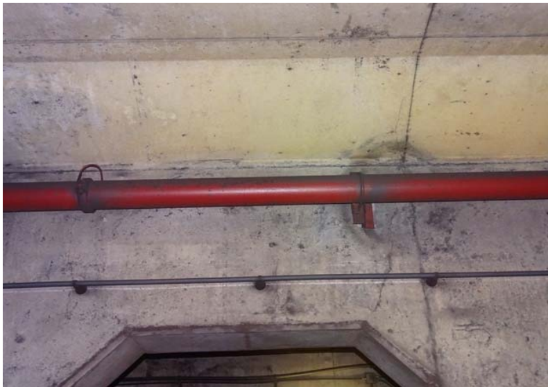
Photograph No. 159 Station 73+60 - cracks and stains above west arch.
