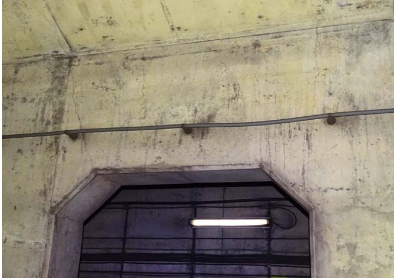
Photograph No. 253 Station 73+60 - cracks above east arch.
