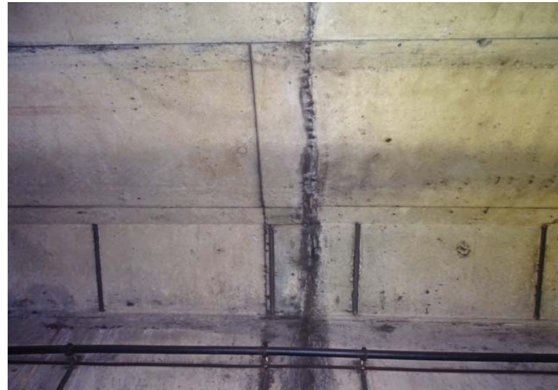
Photograph No. 230 Station 73+20 - stains and efflorescence on west wall.
