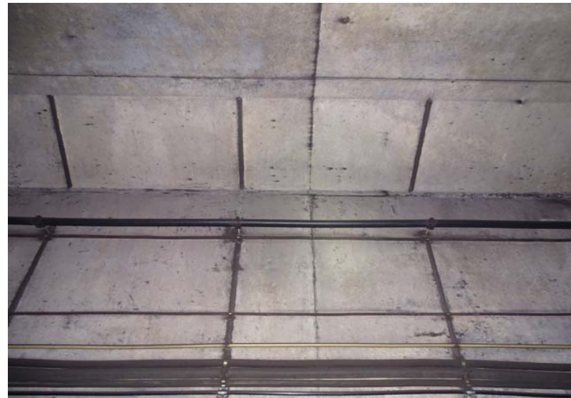
Photograph No. 104 Station 72+40 - joint on the east wall.
