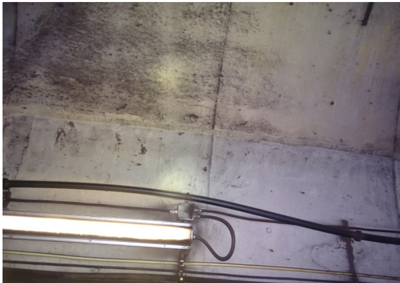
Photograph No. 291 Station 76+82 - vertical crack in east wall.
