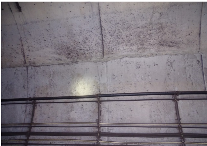
Photograph No. 443 Station 76+22 - vertical crack in west wall.
