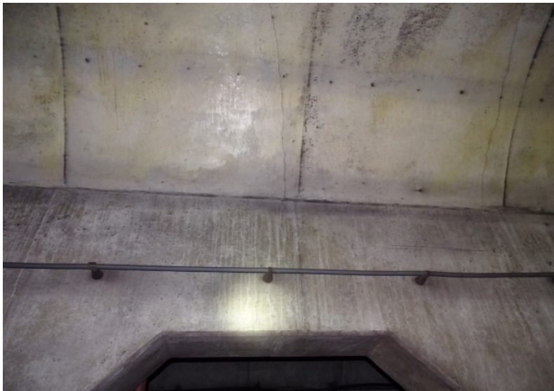
Photograph No. 383 Station 75+44 - vertical crack on east wall.
