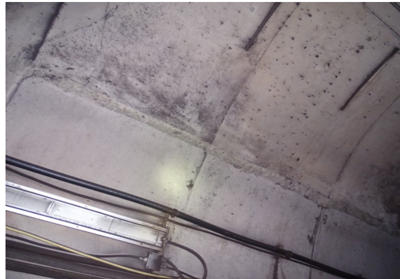
Photograph No. 268 Station 76+41 - vertical crack in east wall.
