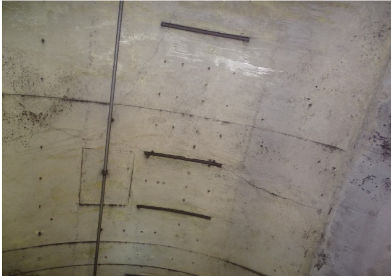
Photograph No. 501 Station 77+12 - crack in ceiling.
