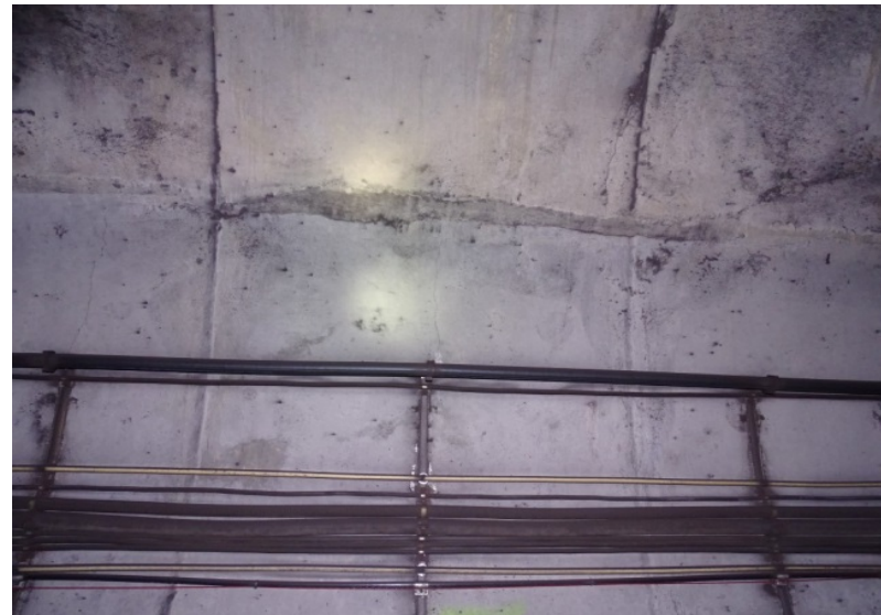
Photograph No. 284 Station 76+70 - crack in east wall.
