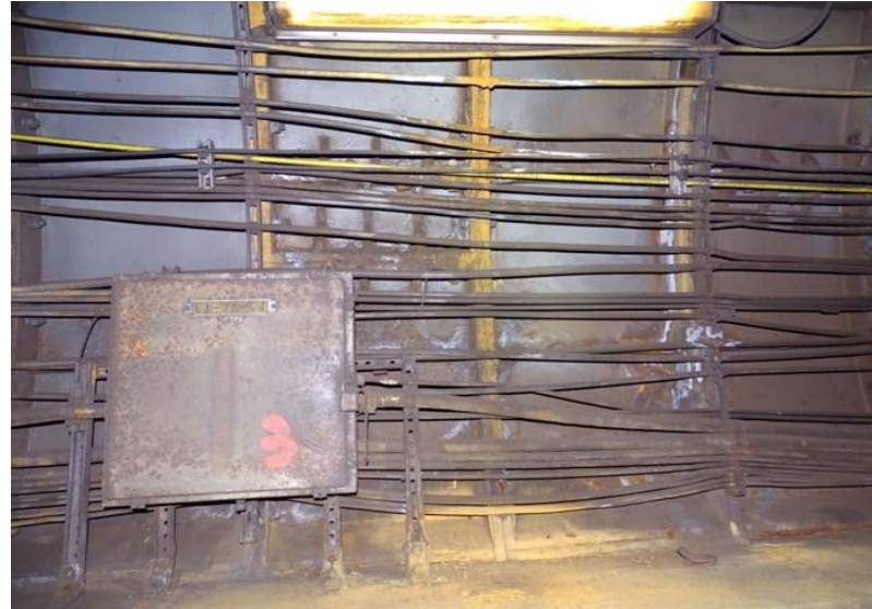
Photograph No. 10 Station 69+80 - corrosion on the east wall.
