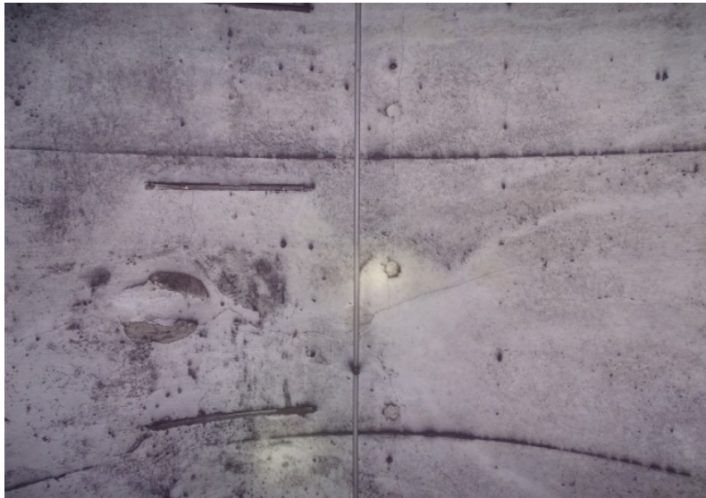
Photograph No. 333 Station 77+85 - crack in ceiling.
