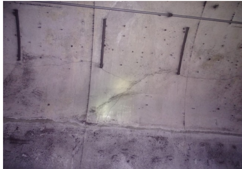
Photograph No. 346 Station 78+25 - transverse crack in east wall.
