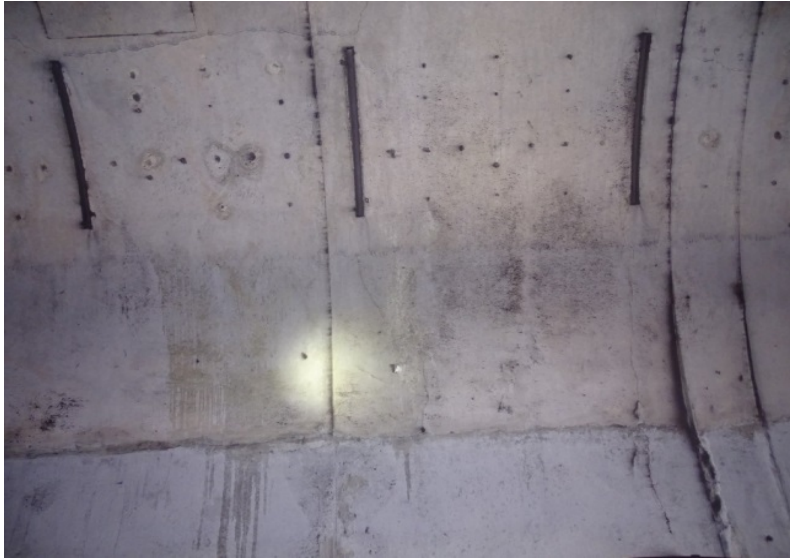
Photograph No. 481 Station 76+85 - vertical crack in upper portion of west wall.
