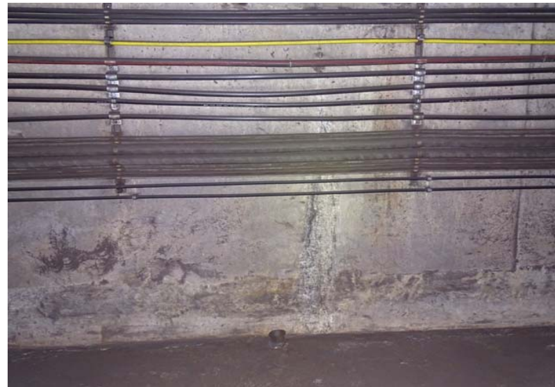
Photograph No. 112 Station 72+60 - crack on the east wall.
