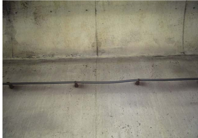
Photograph No. 334 Station 74+80 - crack on east wall.
