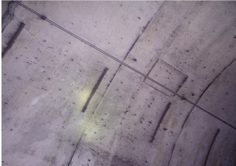
Photograph No. 281 Station 76+61 - crack in ceiling.
