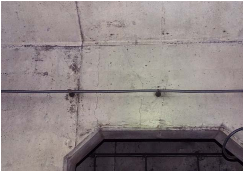
Photograph No. 191 Station 72+70 - cracks above east arch.
