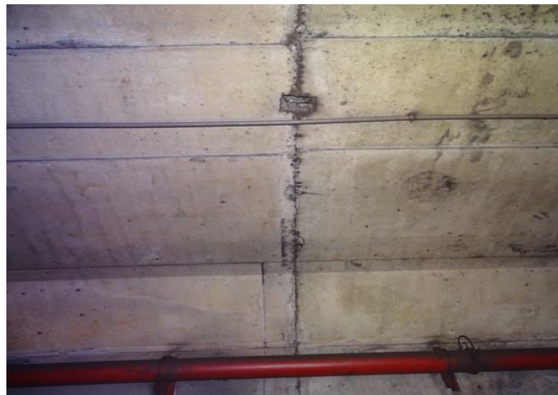
Photograph No. 142 Station 73+20 - crack and stains on the west wall.
