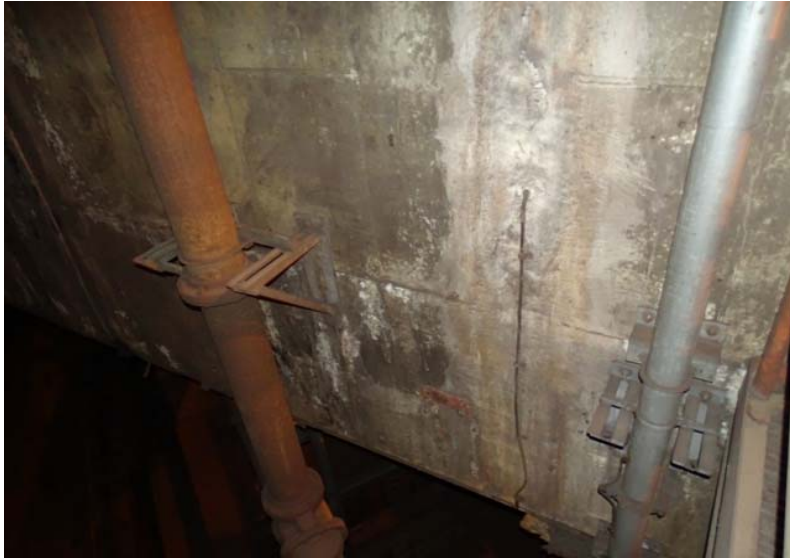
Photograph No. 73 Main room, west wall, close up of efflorescence.
