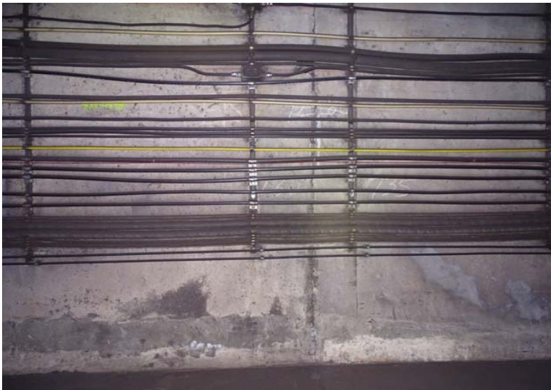
Photograph No. 139 Station 73+20 - crack and stains on the east wall.
