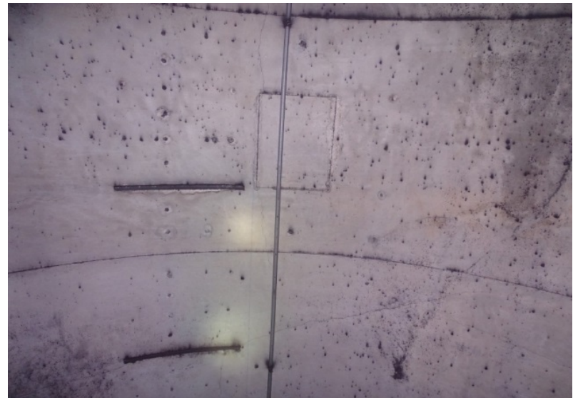
Photograph No. 272 Station 76+45 - crack in ceiling.
