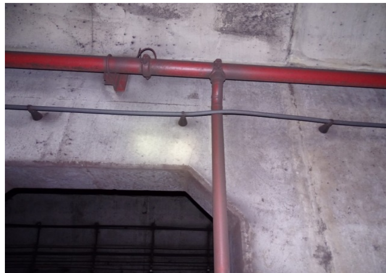
Photograph No. 318 Station 77+41 - vertical crack above west arch.
