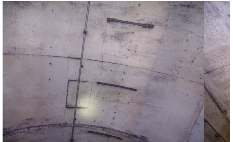
Photograph No. 488 Station 76+95 - crack in ceiling.
