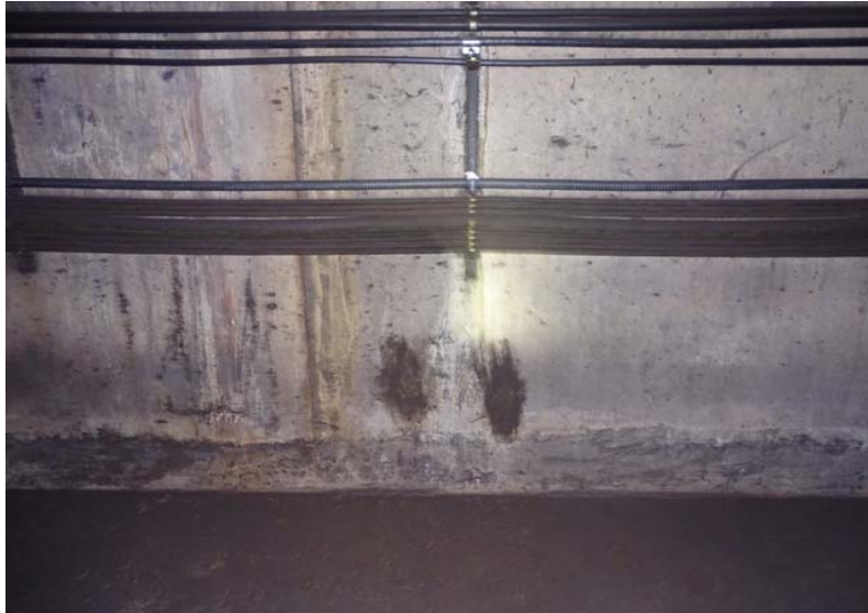
Photograph No. 293 Station 74+20 - stains and efflorescence on west wall.
