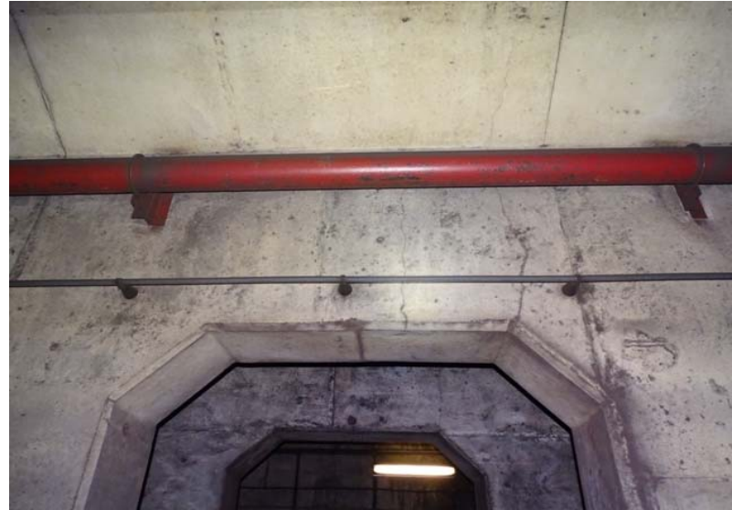
Photograph No. 62 Station 71+40 - cracks above west arch.
