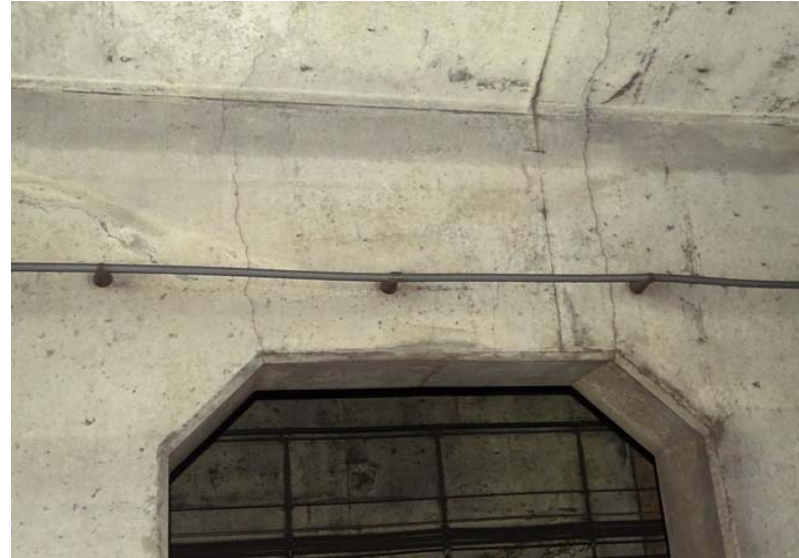
Photograph No. 282 Station 74+10 - cracks above east arch.
