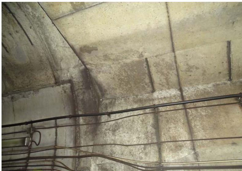
Photograph No. 299 Station 74+30, upper portion of west wall. Note the stains and efflorescence.
