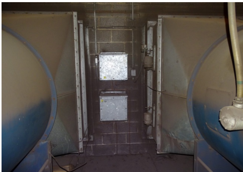
Photograph No. 123 Main room, upper level, west wall, between south and south-center fan units.
