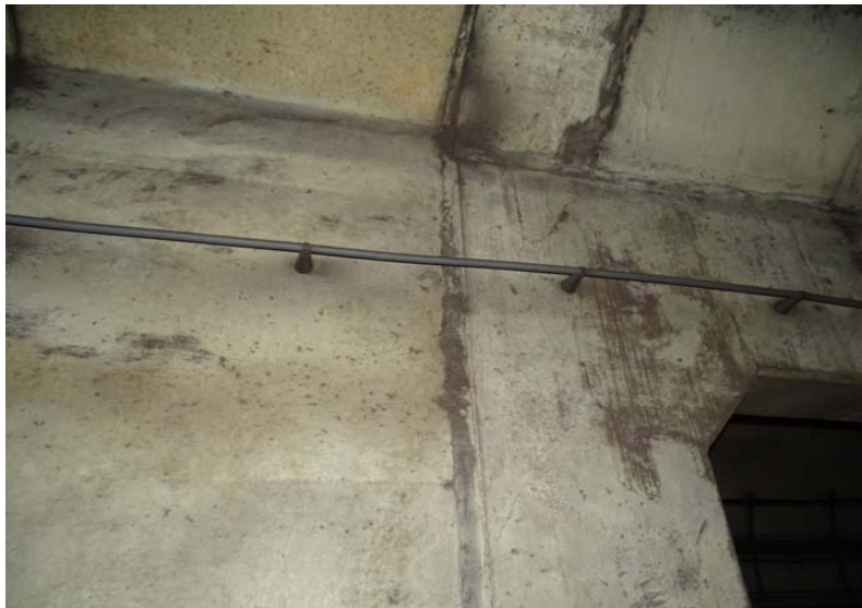
Photograph No. 297 Station 74+30 - crack on east wall.
