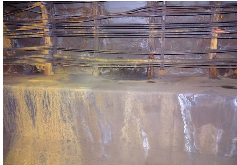
Photograph No. 24 Station 70+10 - stains and efflorescence on the west wall.
