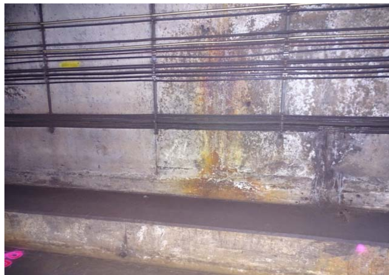
Photograph No. 104 Station 71+40, lower portion of west wall. Note the stains.
