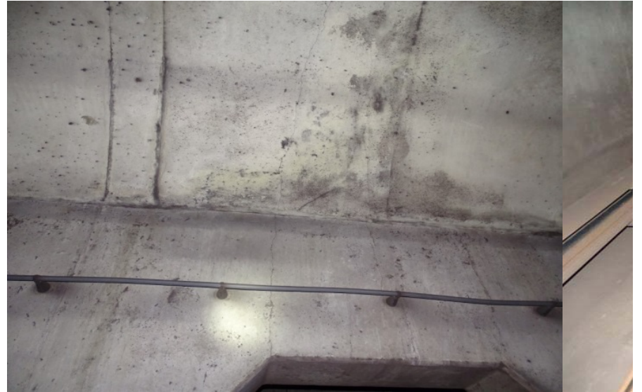
Photograph No. 362 Station 75+15 - vertical crack on east wall.
