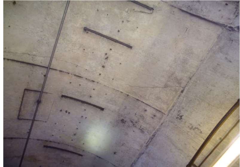
Photograph No. 426 Station 76+00 - crack in west portion of ceiling.
