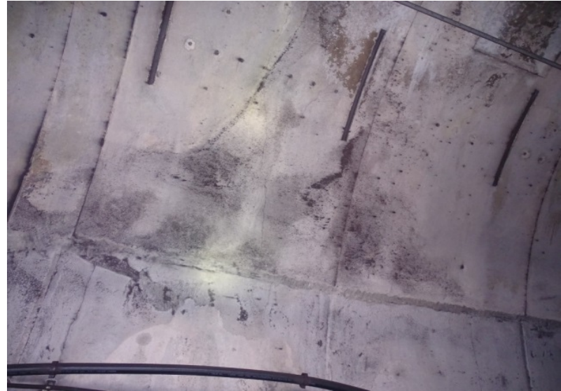
Photograph No. 310 Station 77+22 - vertical crack in east wall.
