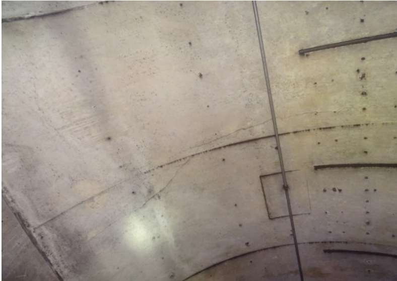
Photograph No. 425 Station 76+00 - crack in east portion of ceiling.
