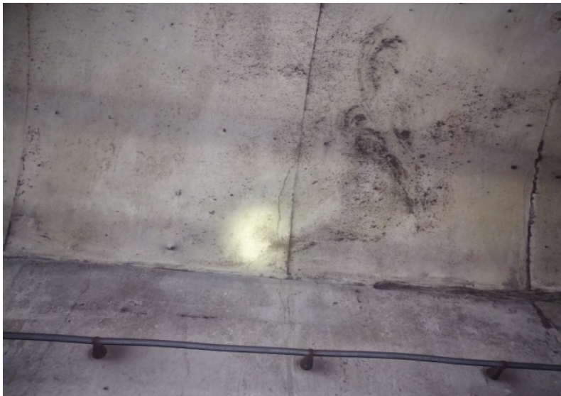
Photograph No. 475 Station 76+75 - vertical crack in upper portion of east wall.
