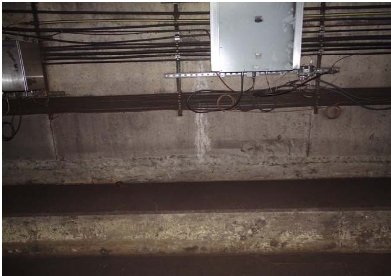
Photograph No. 137 Station 71+90, lower portion of west wall. Note the crack and efflorescence.
