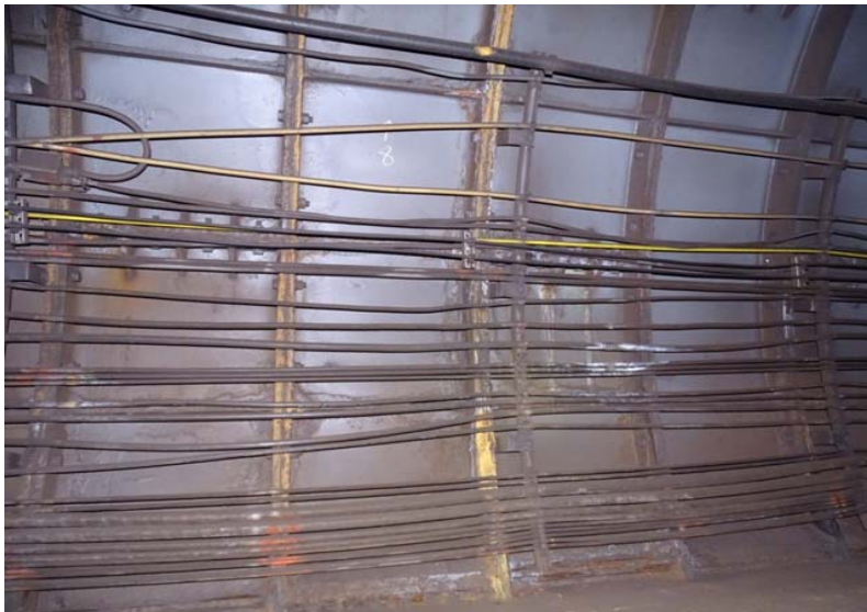
Photograph No. 3 Station 69+60 - corrosion on the east wall.
