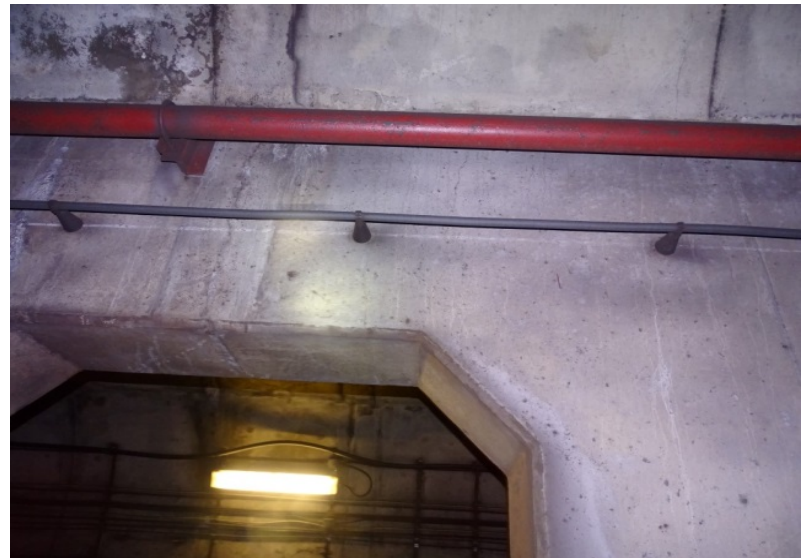
Photograph No. 304 Station 77+20 - vertical crack above west arch.
