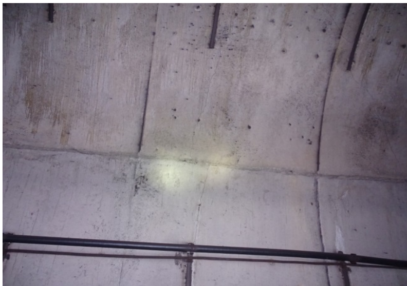
Photograph No. 241 Station 75+82 - vertical crack in east wall.
