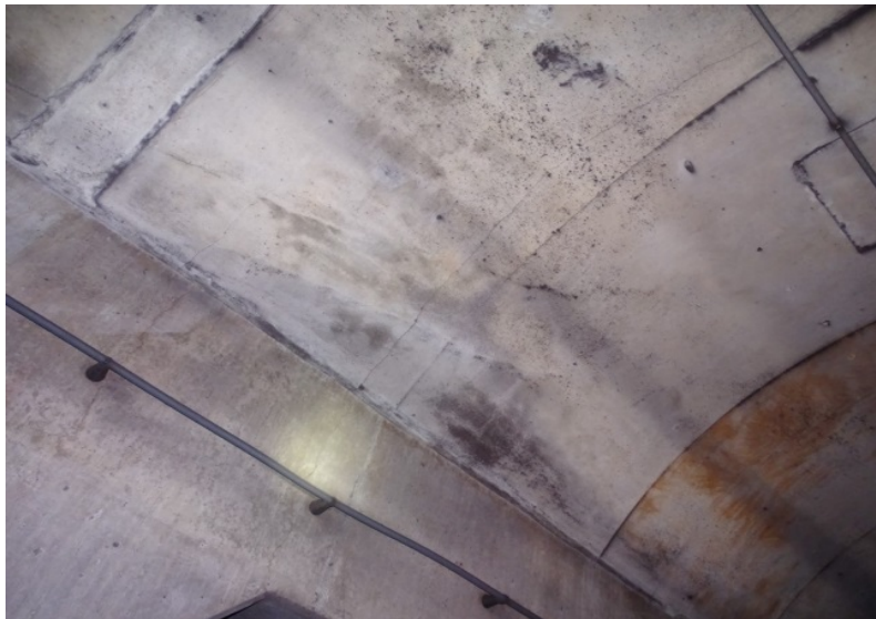
Photograph No. 455 Station 76+40 - vertical crack in east wall.
