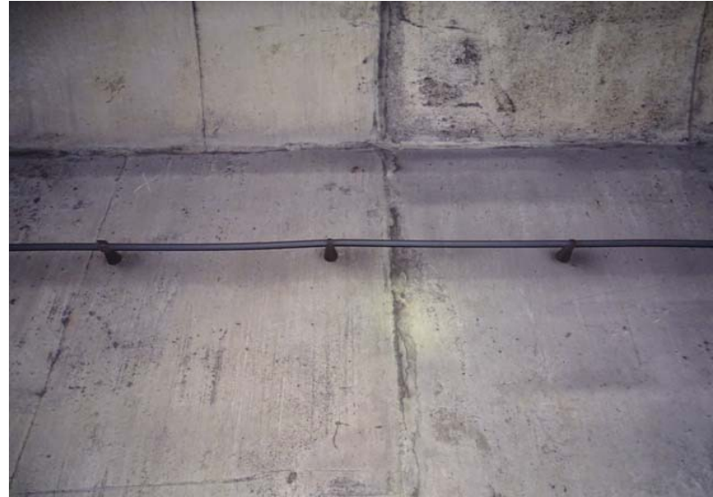
Photograph No. 310 Station 74+50 - crack on east wall.
