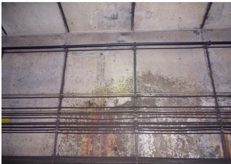
Photograph No. 103 Station 71+40, upper portion of west wall. Note the stains.
