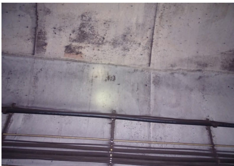
Photograph No. 319 Station 77+48 - vertical crack in east wall.
