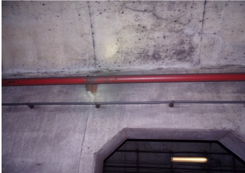
Photograph No. 273 Station 76+45 - crack above west arch.
