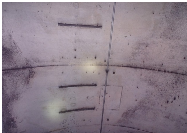
Photograph No. 320 Station 77+50 - transverse crack in ceiling.
