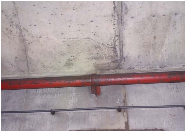
Photograph No. 203 Station 74+80 - cracks on the west wall.
