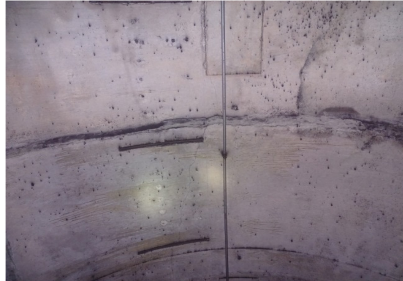
Photograph No. 274 Station 76+56 - crack in ceiling.
