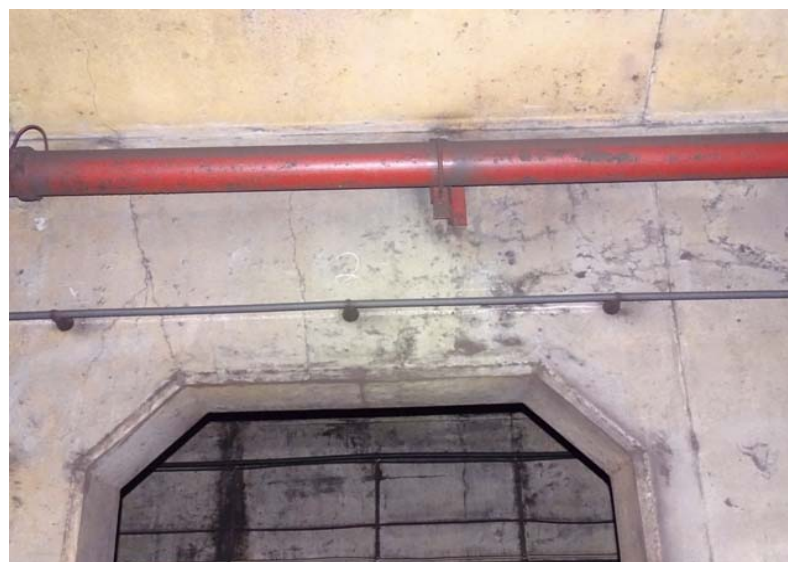
Photograph No. 144 Station 73+20 - cracks and stains above west arch.
