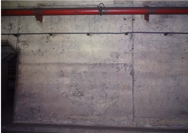
Photograph No. 61 Station 71+40 - crack on the west wall.
