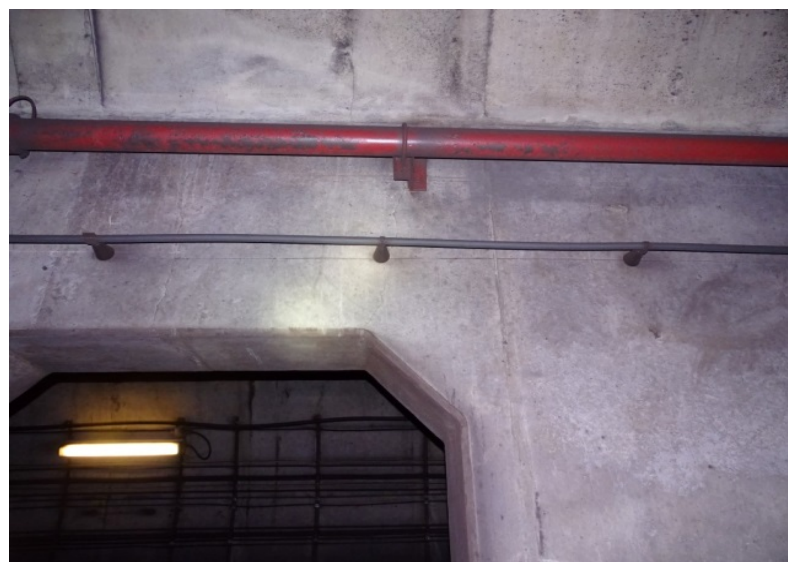
Photograph No. 244 Station 75+91 - vertical crack above west arch.
