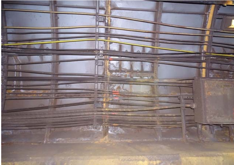
Photograph No. 9 Station 69+80 - corrosion on the east wall.
