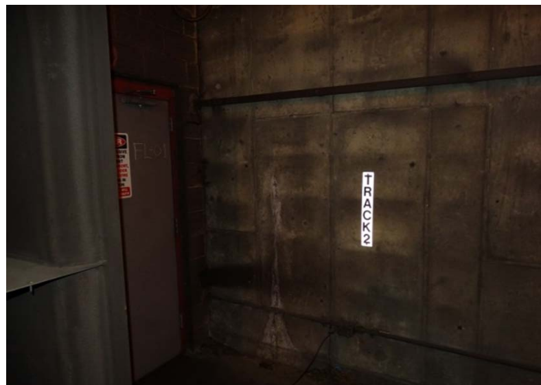
Photograph No. 156 Upper fan room, south wall, lower-east portion - vertical crack and efflorescence.
