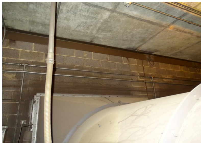
Photograph No. 124 Main room, upper level, west wall, above south-center fan unit.
