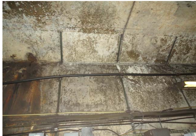
Photograph No. 40 Station 70+80 - stains on the east wall.
