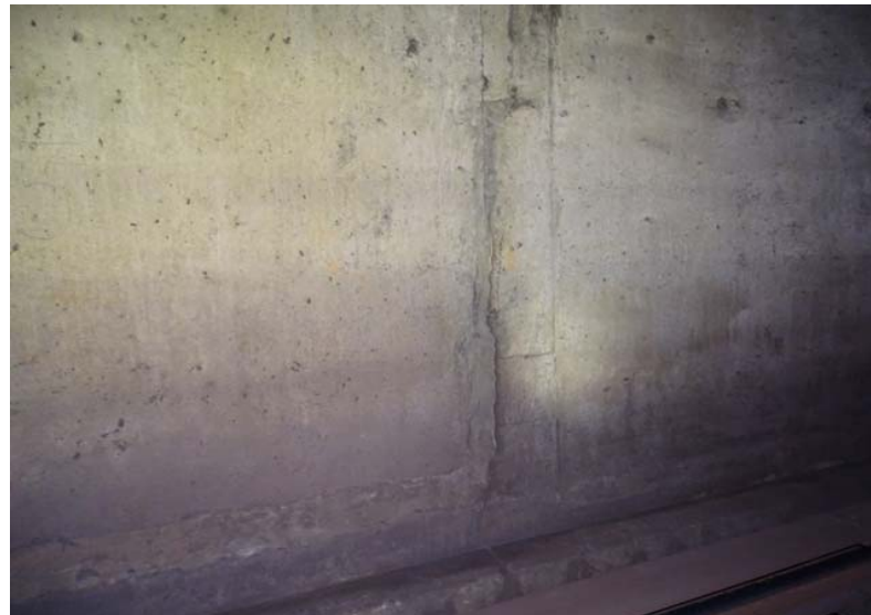
Photograph No. 226 Station 73+20 - crack on east wall.
