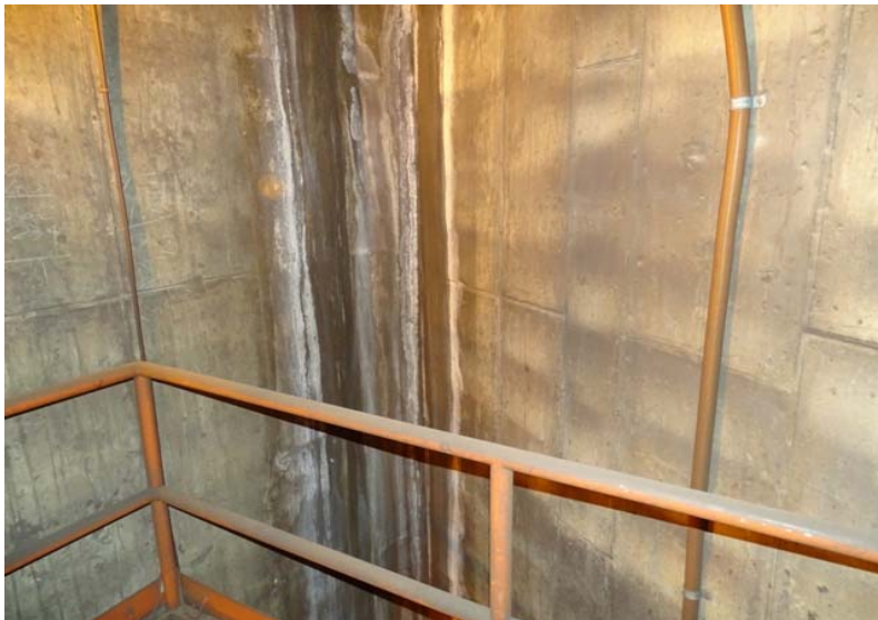
Photograph No. 79 Main room, northwest corner, close up of efflorescence.
