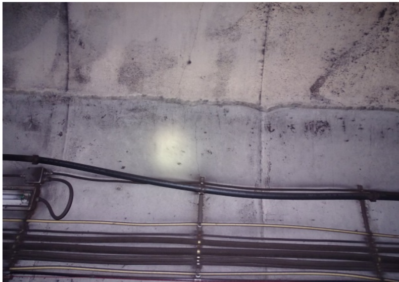
Photograph No. 327 Station 77+70 - vertical crack in east wall.
