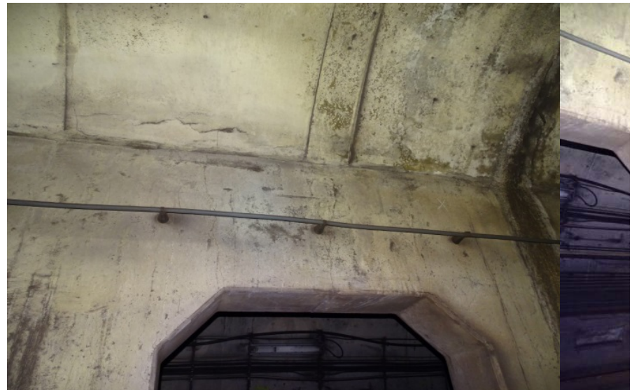
Photograph No. 500 Station 77+12 - vertical crack above east arch.
