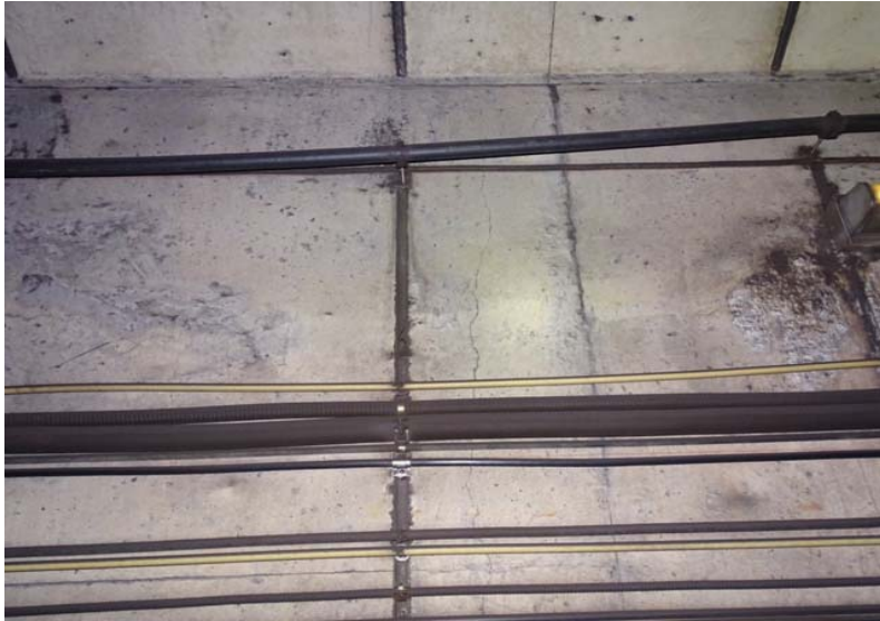
Photograph No. 57 Station 71+40 - crack on the east wall.
