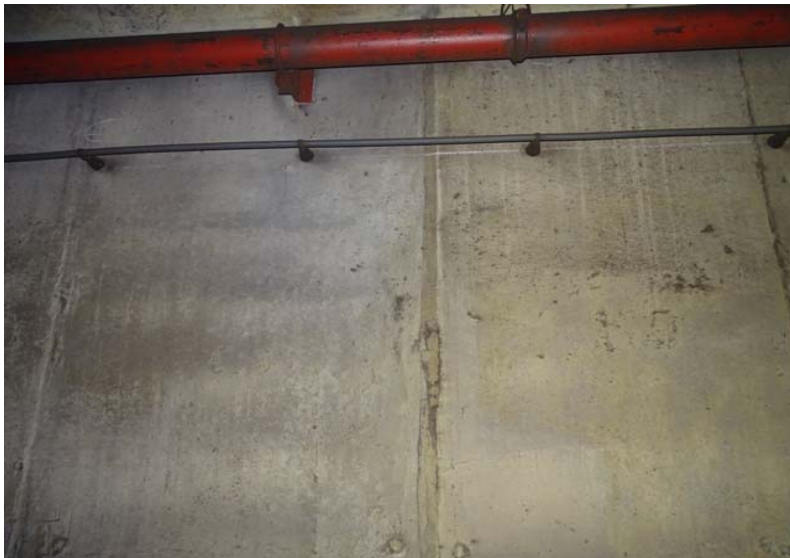
Photograph No. 187 Station 74+40 - previous repair at the joint.
