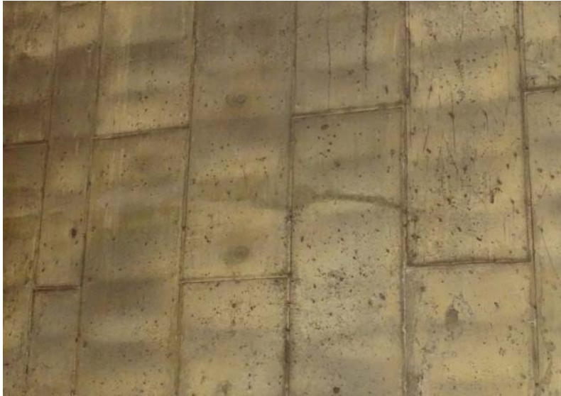
Photograph No. 65 Main room, east wall, close up of stain.
