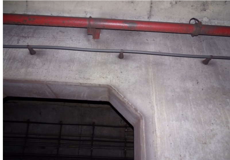
Photograph No. 326 Station 77+66 - vertical crack above west arch.
