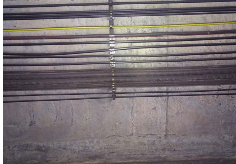
Photograph No. 58 Station 71+40 - crack on the east wall.
