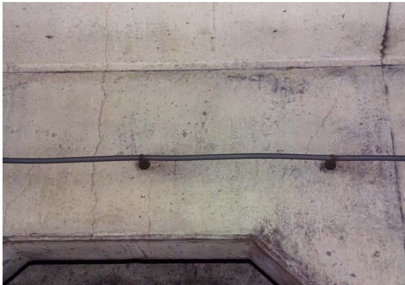
Photograph No. 101 Station 71+40 - cracks above east arch.
