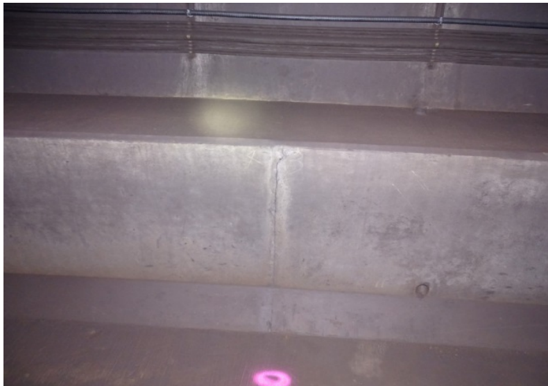
Photograph No. 417 Station 75+90 - crack in safety walkway.
