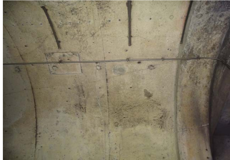
Photograph No. 178 Station 74+20 - cracks on the ceiling, looking west.
