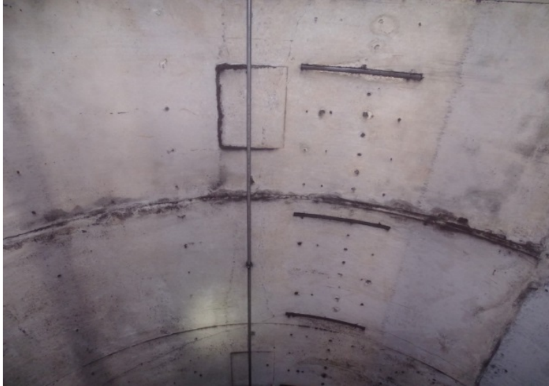
Photograph No. 461 Station 76+55 - longitudinal crack in ceiling.
