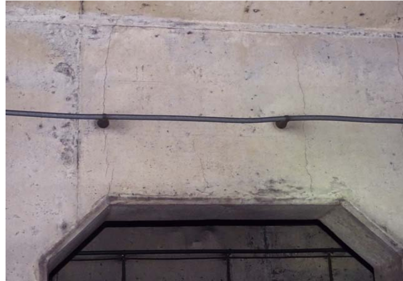
Photograph No. 150 Station 72+10 - cracks above east arch.
