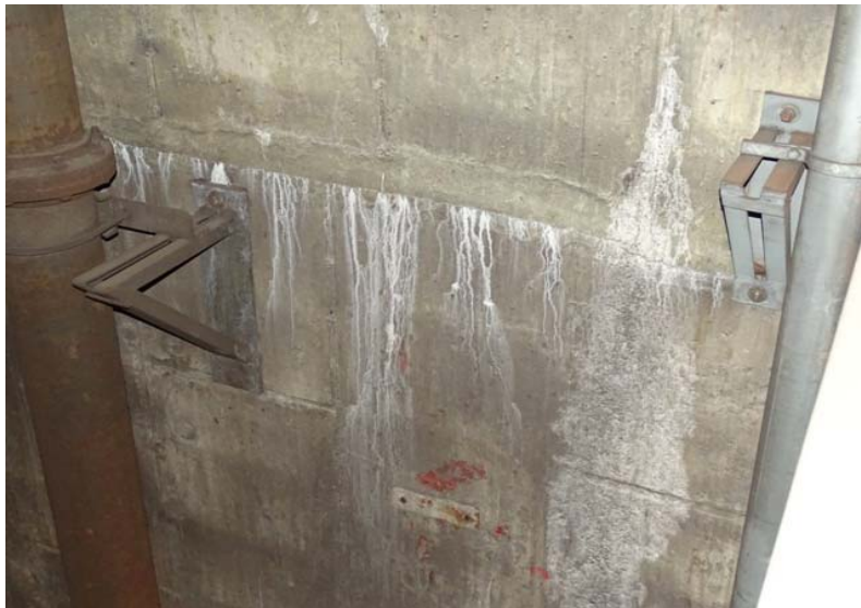
Photograph No. 99 Main room, upper portion, west wall at the stair, close up of efflorescence.
