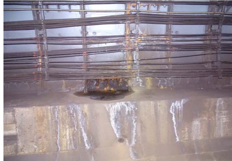
Photograph No. 14 Station 69+90 - active leak, stains, and efflorescence on the west wall.
