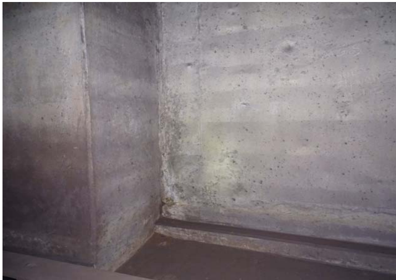
Photograph No. 127 Station 71+80 - stains and efflorescence at the lower portion of the east wall.
