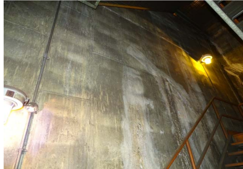
Photograph No. 82 Main room, west wall, top of the stair. Note the efflorescence.
