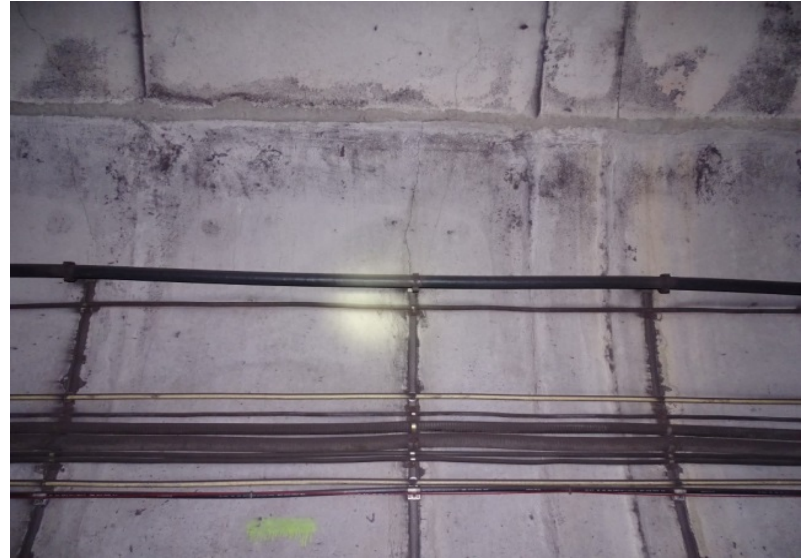
Photograph No. 210 Station 75+10 - crack on east wall.
