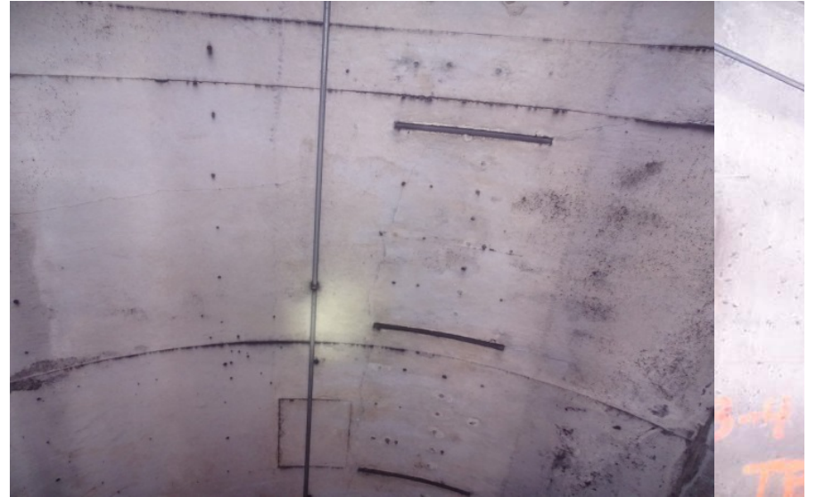
Photograph No. 530 Station 77+65 - transverse crack in ceiling.
