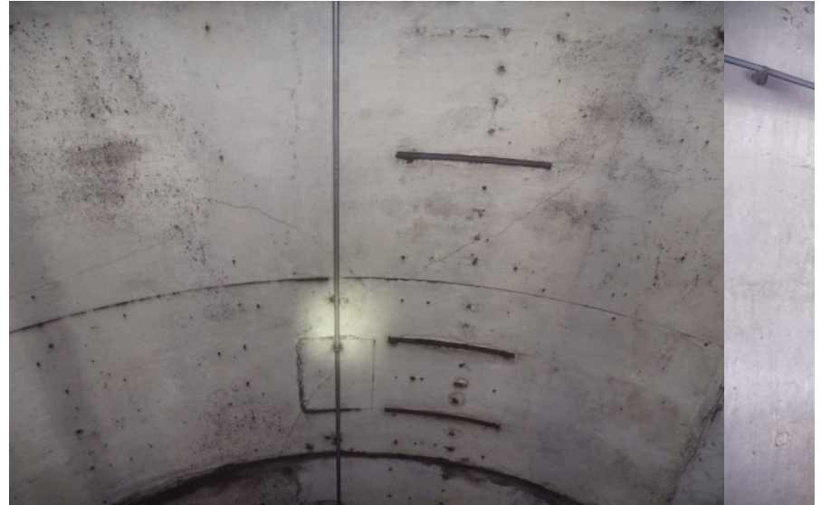
Photograph No. 370 Station 75+28 - cracks in ceiling.
