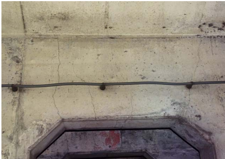
Photograph No. 115 Station 71+60 - cracks above east arch.
