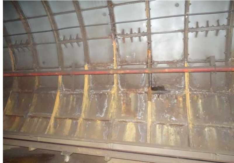
Photograph No. 6 Station 69+60 - active leak and corrosion on the west wall.
