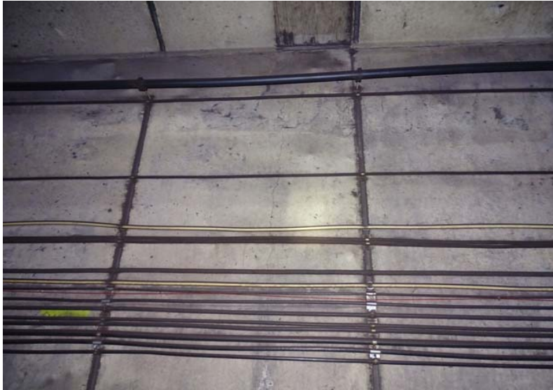
Photograph No. 181 Station 72+50 - crack and efflorescence on west wall.
