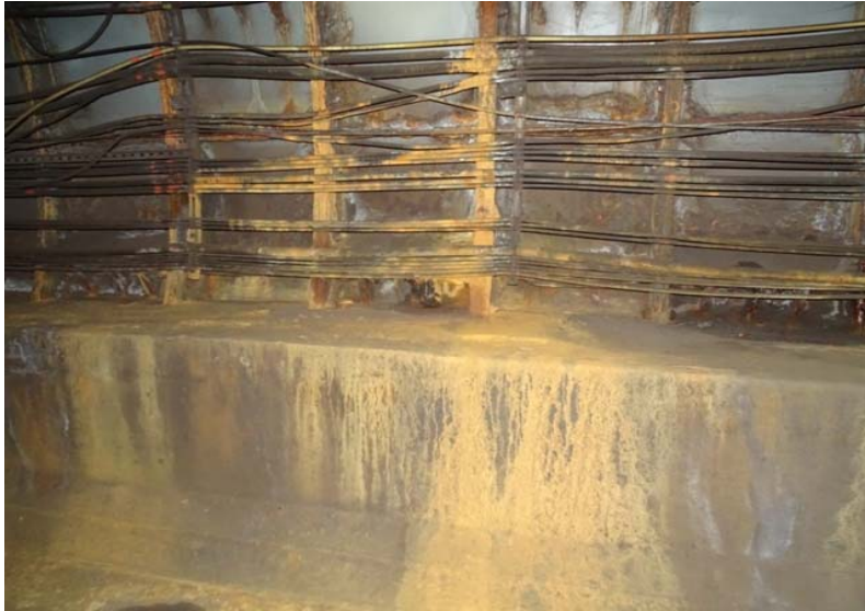
Photograph No. 29 Station 70+20 - stains and efflorescence on the west wall.
