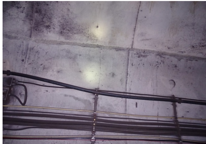
Photograph No. 312 Station 77+28 - vertical crack in east wall.
