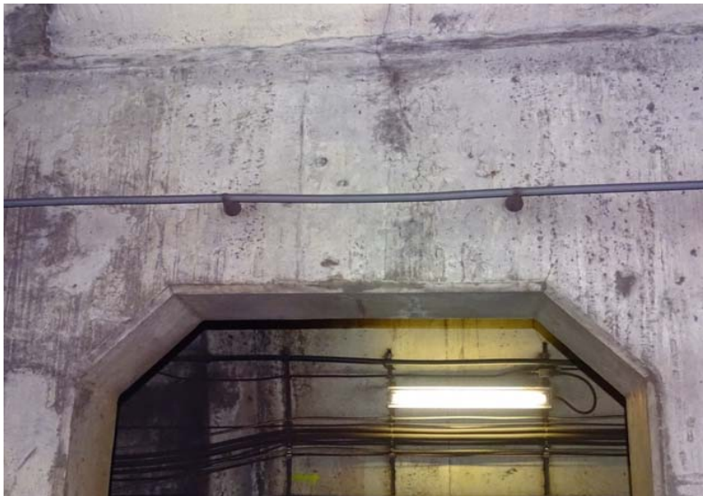
Photograph No. 303 Station 74+40 - cracks and stains above east arch.
