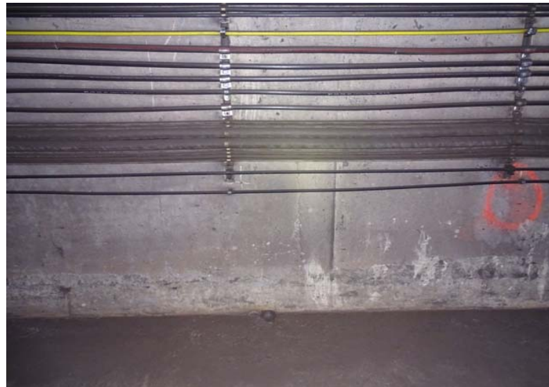
Photograph No. 86 Station 72+00 - crack on the east wall.
