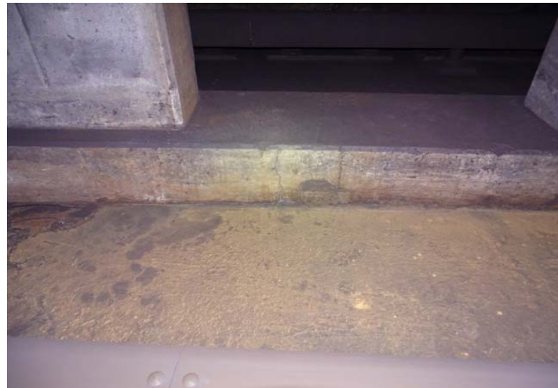
Photograph No. 80 Station 71+80 - crack in the concrete.
