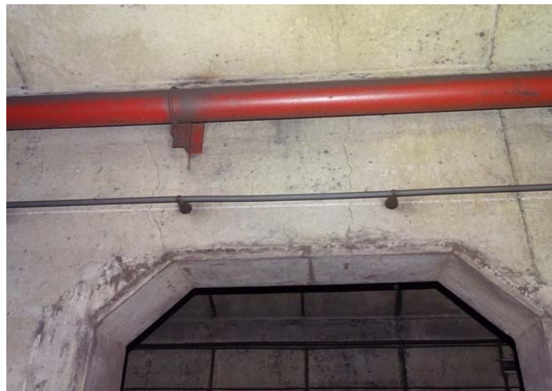
Photograph No. 126 Station 72+80 - cracks above west arch.
