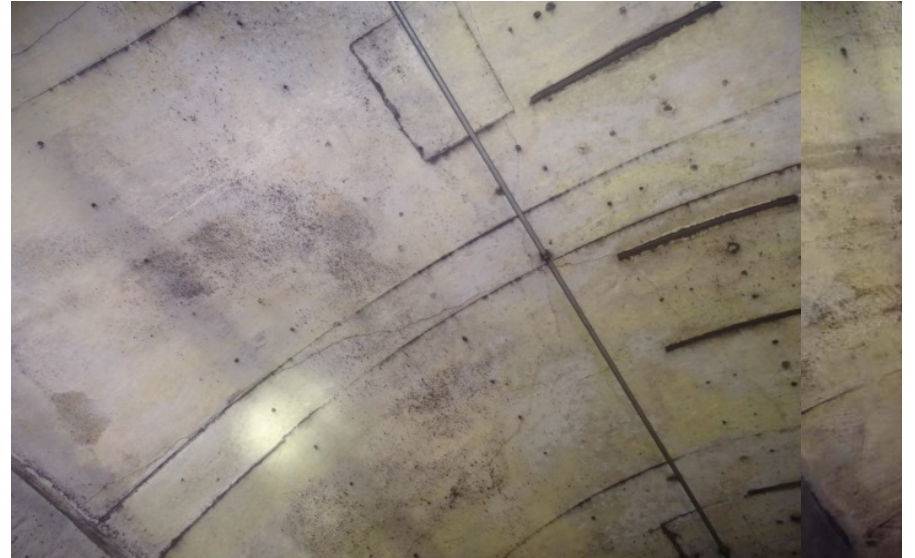
Photograph No. 390 Station 75+55 - crack in ceiling.
