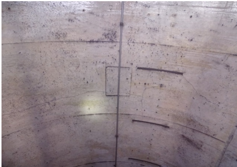
Photograph No. 411 Station 75+85 - cracks in ceiling.
