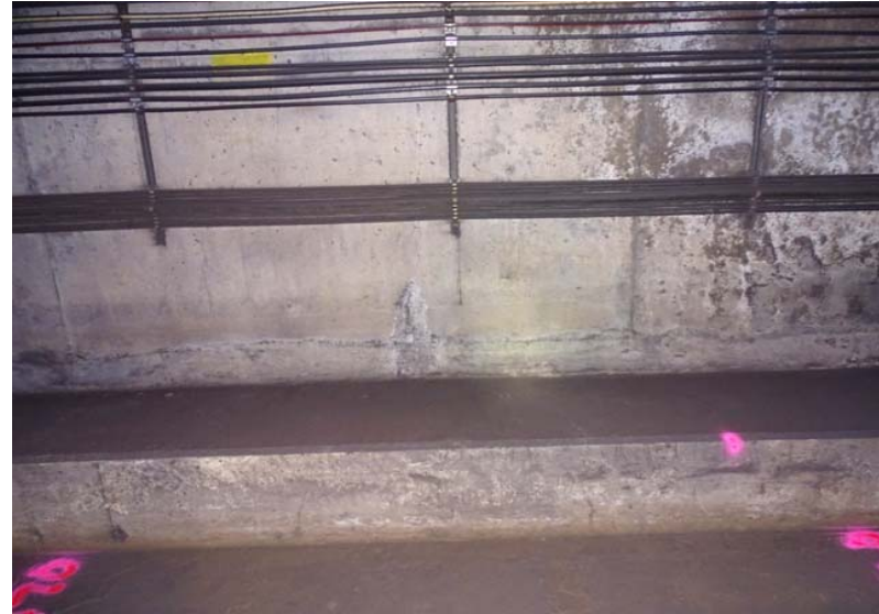
Photograph No. 118 Station 71+60, lower portion of west wall. Note the cracks and stains.
