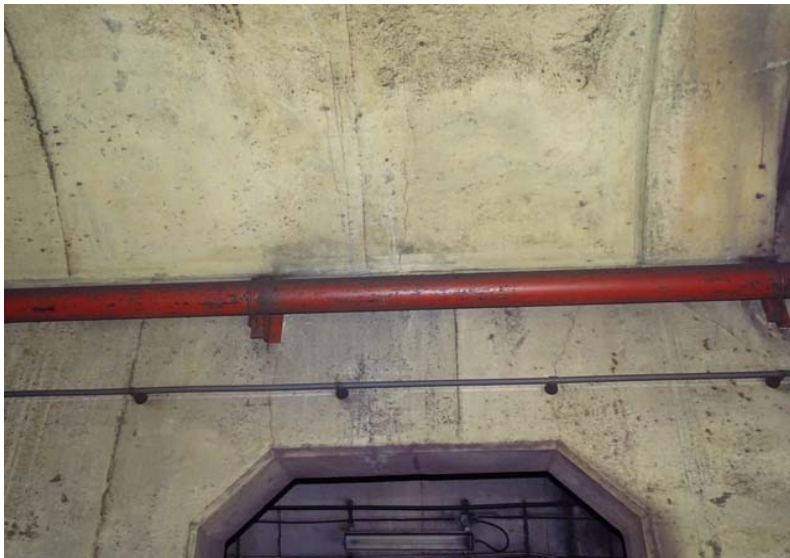
Photograph No. 179 Station 74+20 - cracks above west arch.
