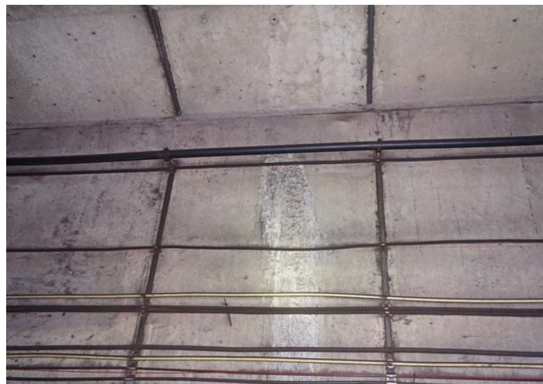
Photograph No. 268 Station 73+80 - efflorescence on the west wall.
