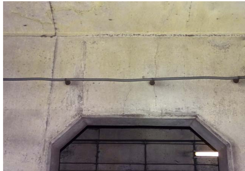
Photograph No. 172 Station 72+40 - cracks above east arch.
