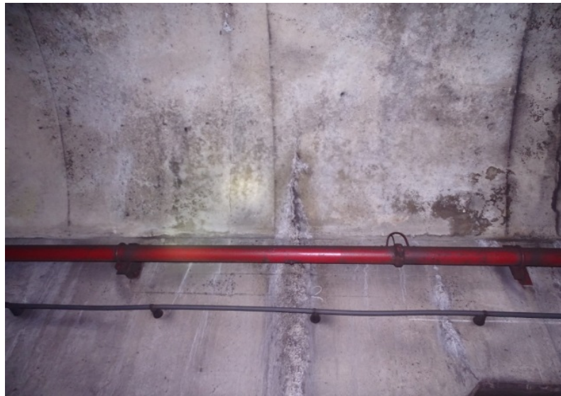
Photograph No. 311 Station 77+25 - vertical crack in west wall.
