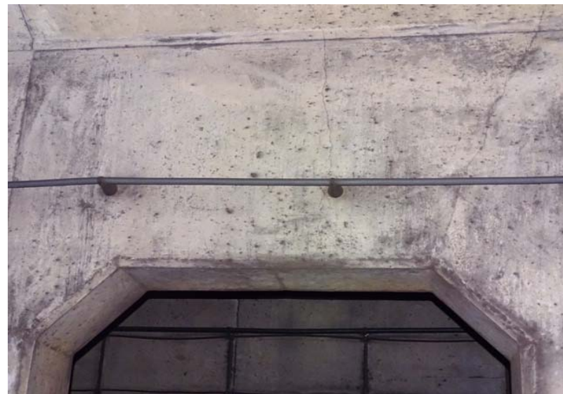
Photograph No. 240 Station 73+40 - cracks above east arch.
