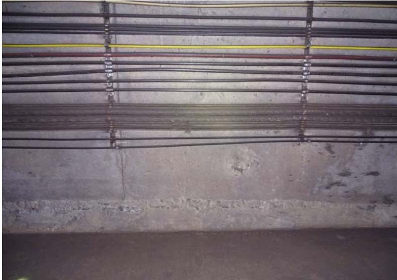
Photograph No. 73 Station 71+80 - crack on the east wall.
