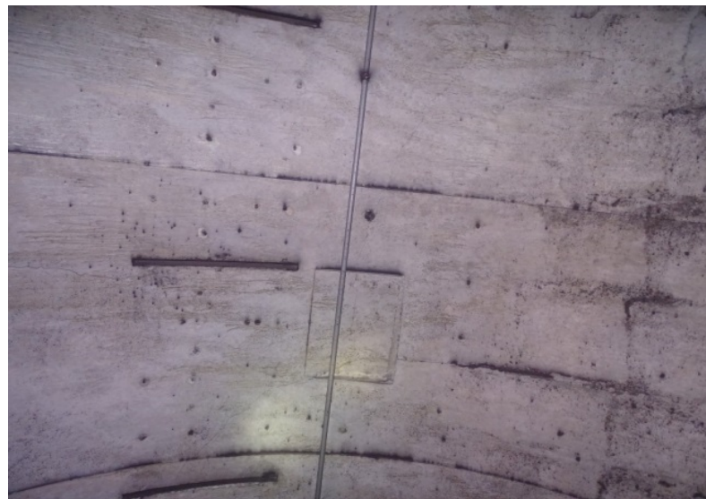
Photograph No. 242 Station 75+82 - transverse crack in ceiling.
