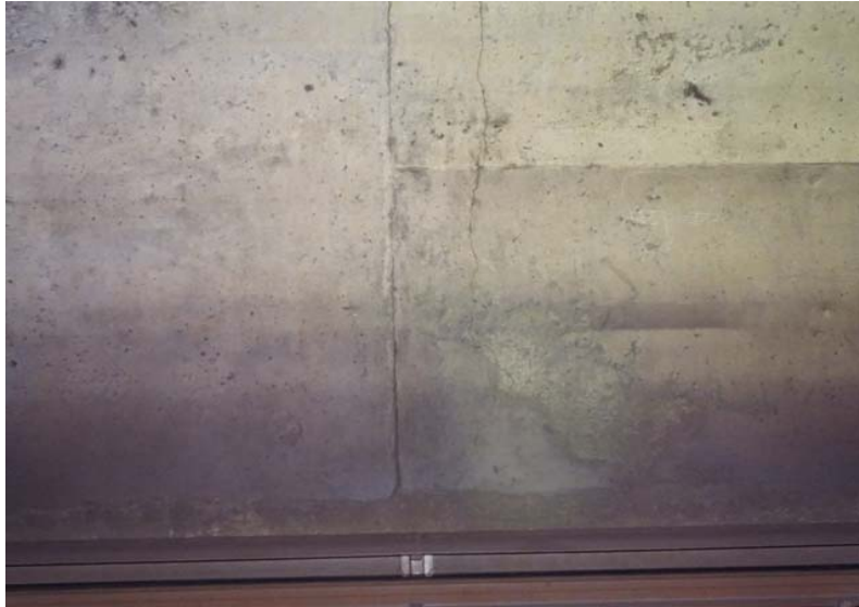
Photograph No. 109 Station 71+50 - crack on the east wall.
