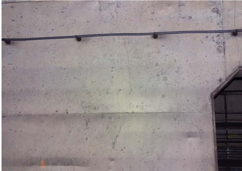
Photograph No. 149 Station 72+10 - crack on east wall.
