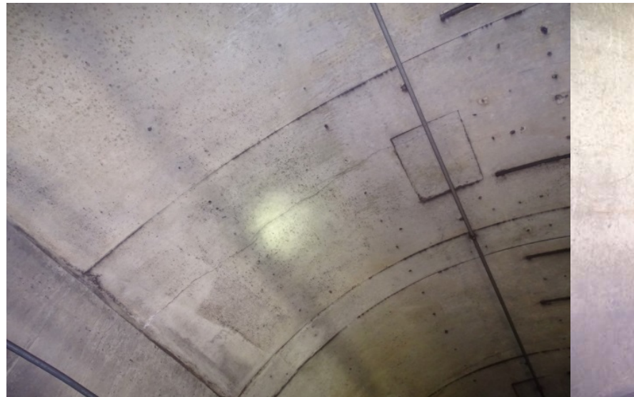
Photograph No. 418 Station 75+94 - crack in east portion of ceiling.
