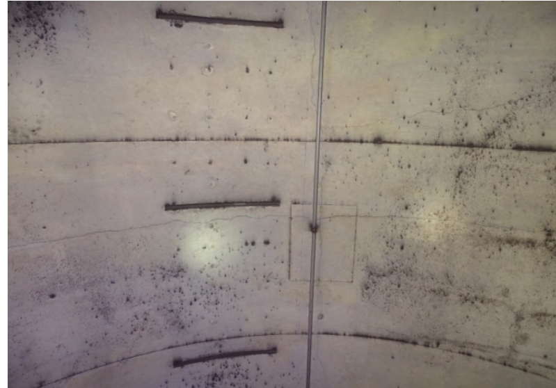
Photograph No. 234 Station 75+61 - transverse crack in ceiling.
