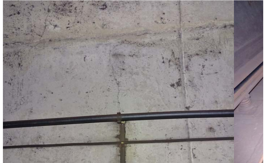
Photograph No. 346 Station 74+90 - crack on west wall.
