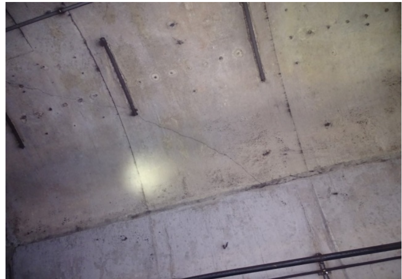
Photograph No. 428 Station 76+08 - crack in west portion of ceiling.
