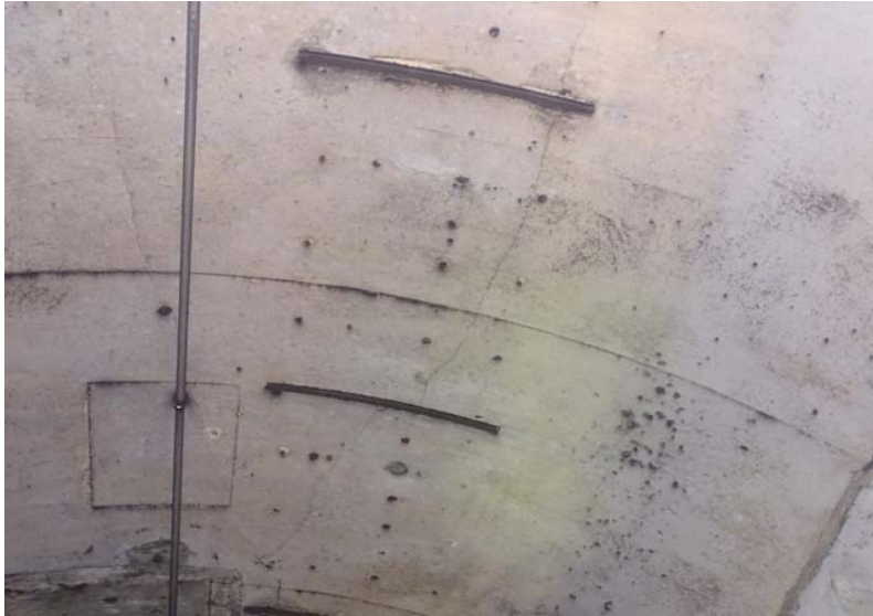
Photograph No. 313 Station 74+50 - crack on ceiling.
