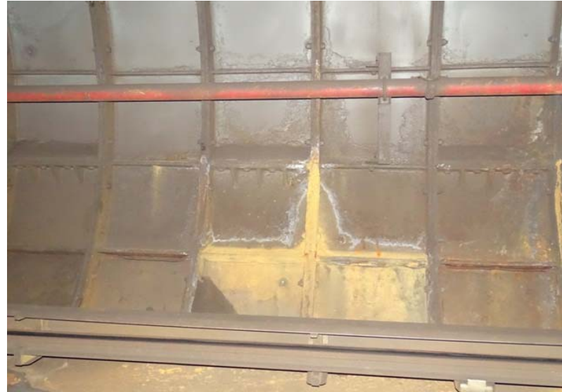
Photograph No. 14 Station 69+80 - corrosion on the west wall.
