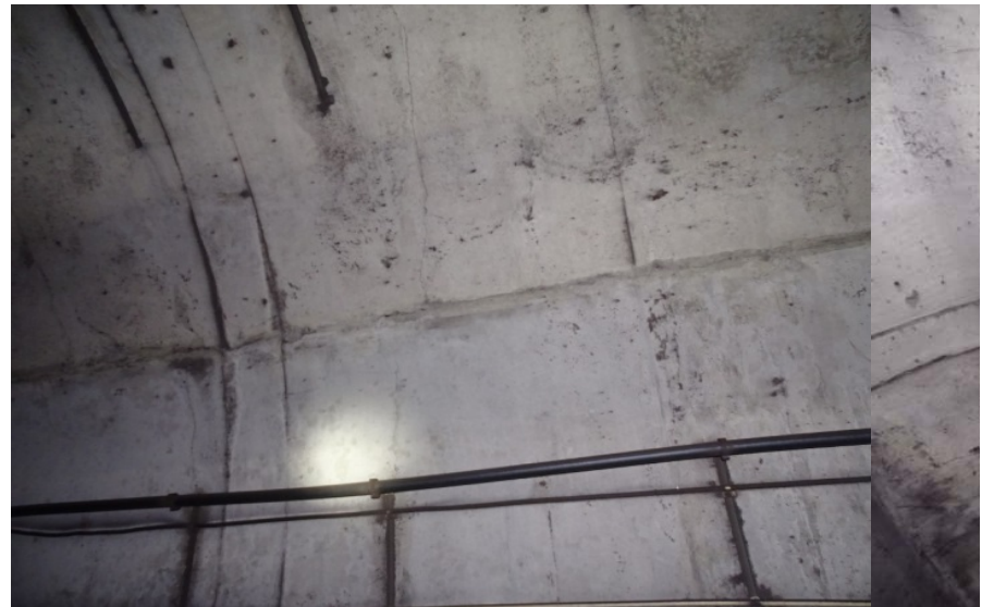
Photograph No. 356 Station 75+09 - crack on upper portion of west wall.
