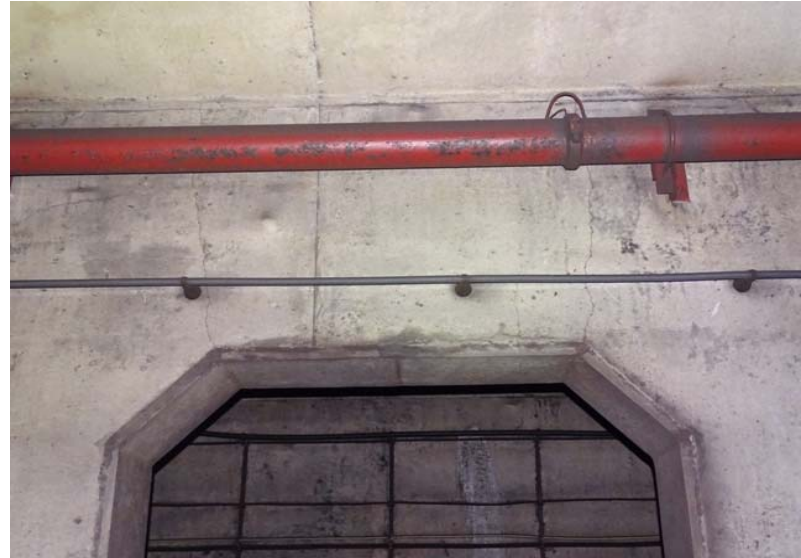
Photograph No. 166 Station 73+80 - cracks above west arch.
