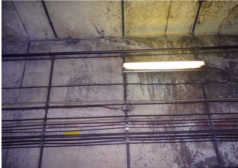
Photograph No. 117 Station 71+60, upper portion of west wall. Note the stains.
