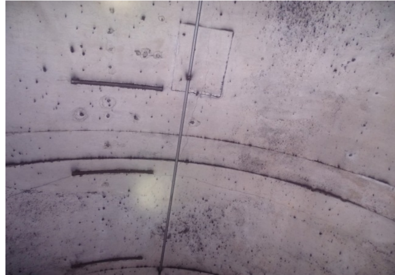
Photograph No. 262 Station 76+35 - transverse crack in ceiling.
