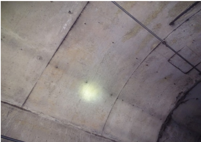
Photograph No. 427 Station 76+08 - crack in east portion of ceiling.
