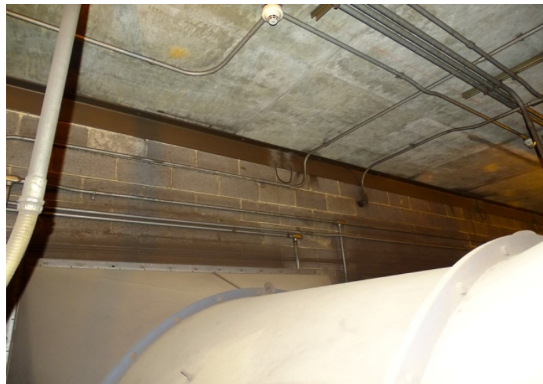
Photograph No. 122 Main room, upper level, west wall, above south fan unit.
