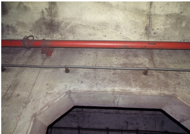
Photograph No. 353 Station 78+43 - vertical cracks above west arch.
