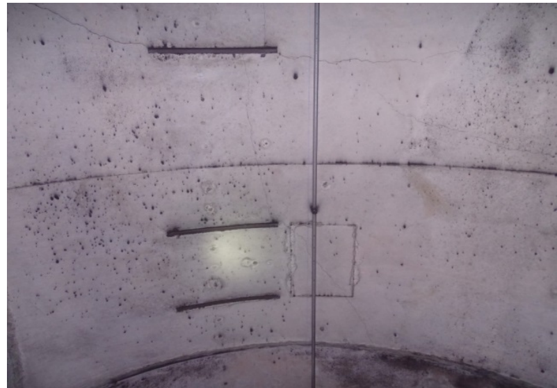
Photograph No. 220 Station 75+30 - crack in ceiling.
