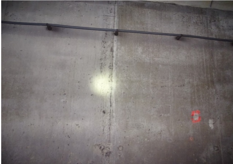
Photograph No. 377 Station 75+35 - vertical crack in east wall.
