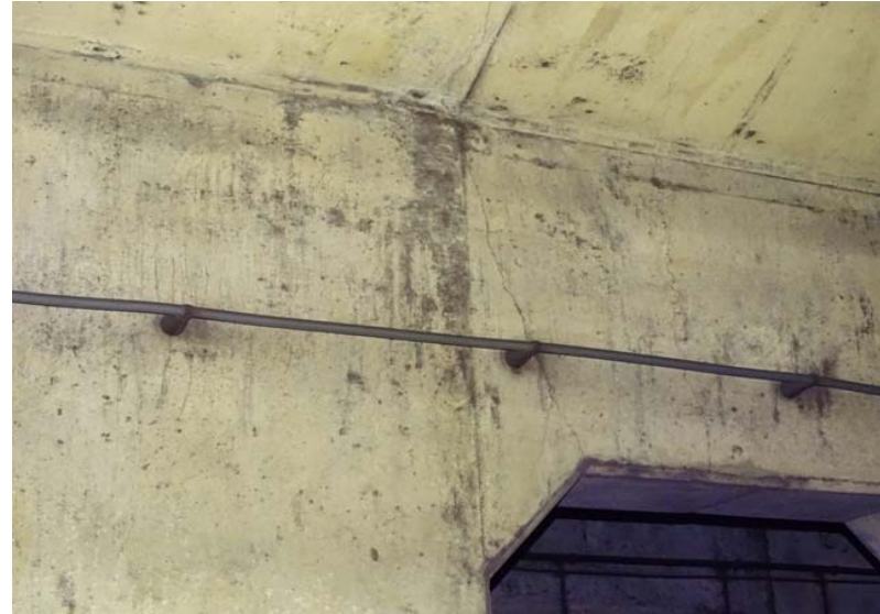
Photograph No. 246 Station 73+50 - cracks above east arch.
