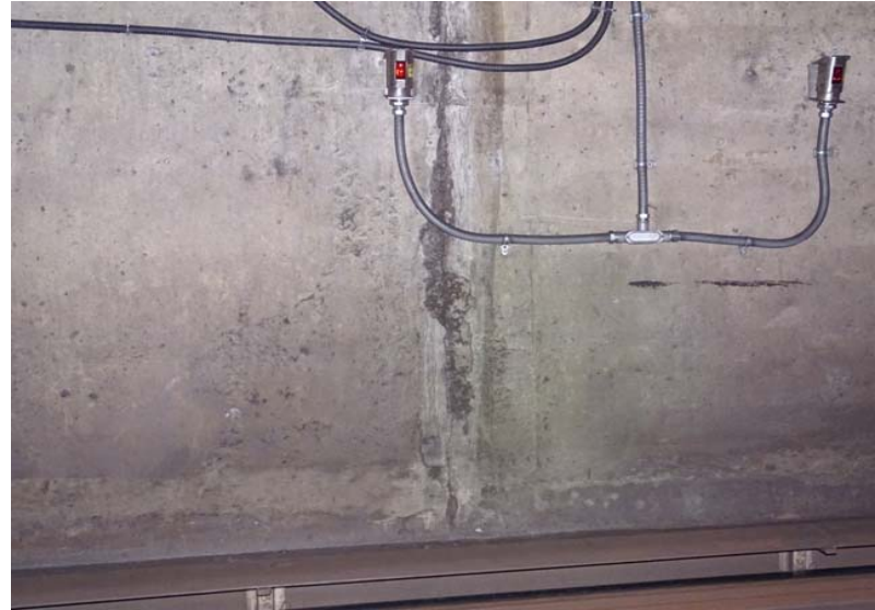
Photograph No. 198 Station 72+80 - stains and efflorescence on east wall.
