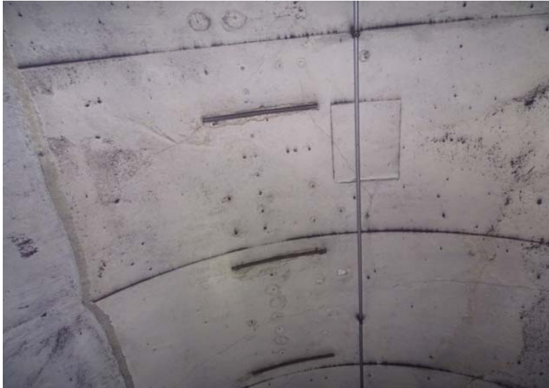
Photograph No. 201 Station 74+80 - cracks on the ceiling.
