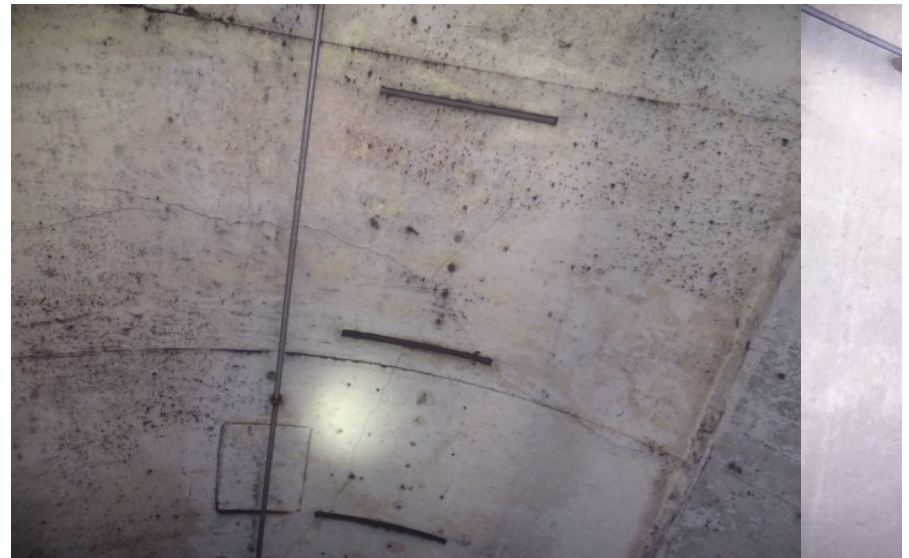
Photograph No. 404 Station 75+70 - cracks in ceiling.
