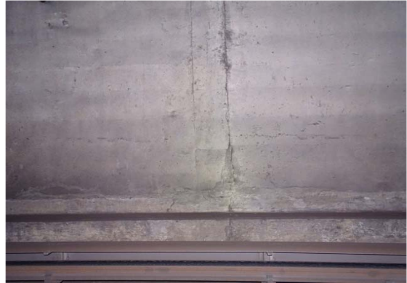
Photograph No. 98 Station 72+20 - crack on the west wall.
