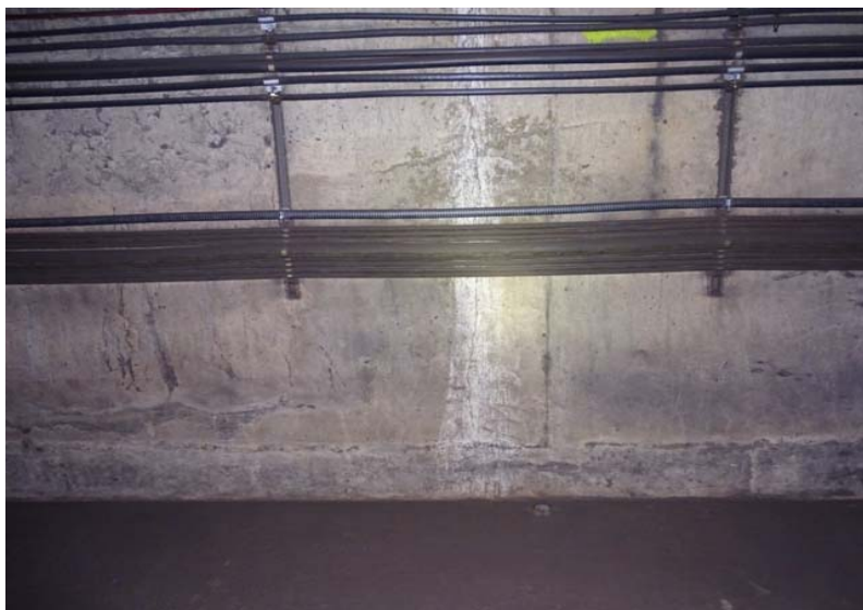
Photograph No. 287 Station 74+10 - crack and efflorescence on west wall.
