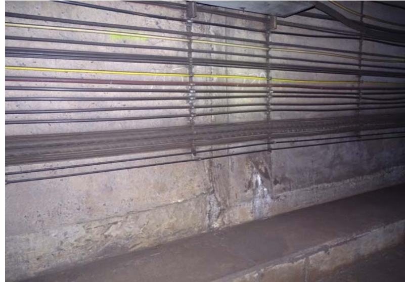
Photograph No. 66 Station 71+60 - efflorescence on the east wall.
