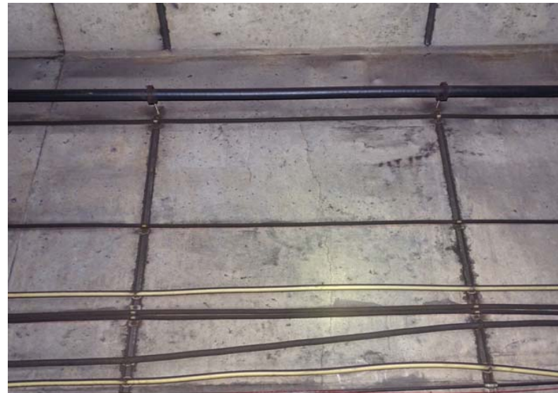
Photograph No. 154 Station 72+10 - crack on west wall.
