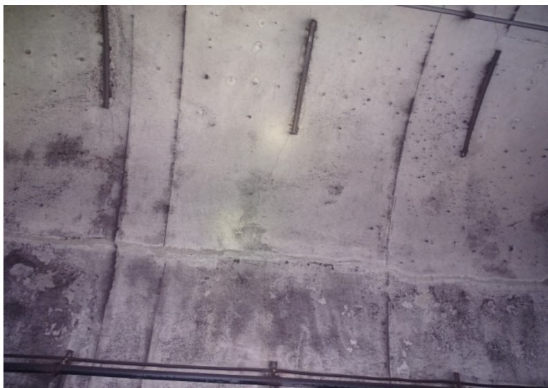
Photograph No. 355 Station 78+57 - crack in east wall.
