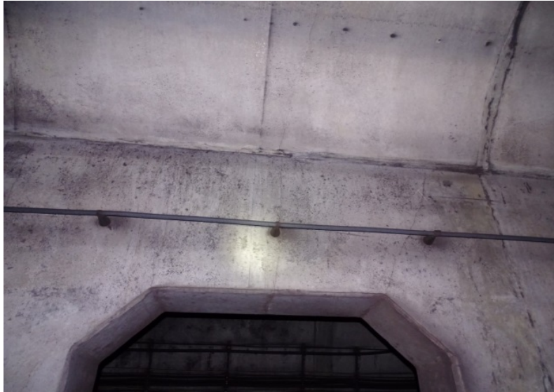
Photograph No. 565 Station 78+75 - vertical crack above east arch.
