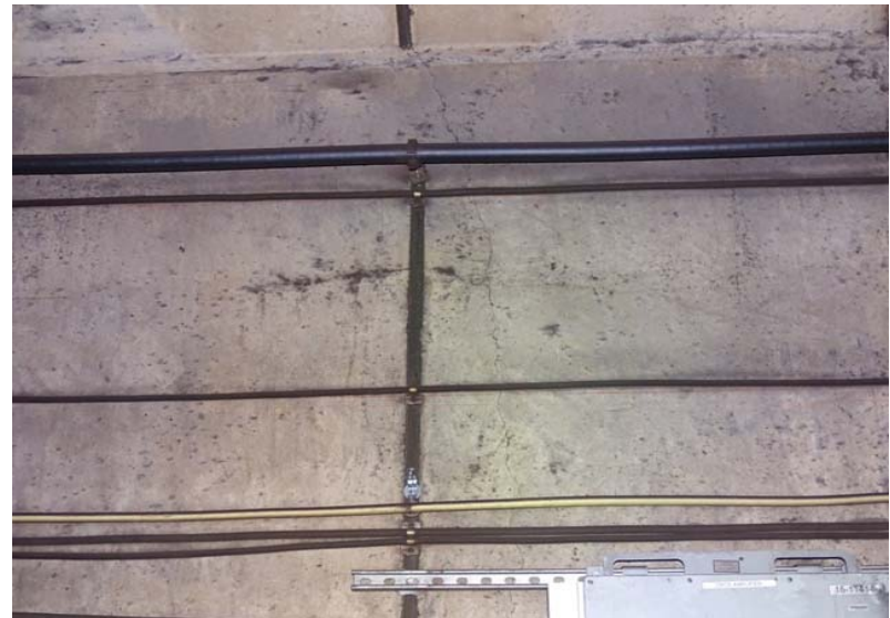
Photograph No. 136 Station 71+90 - crack on the west wall.
