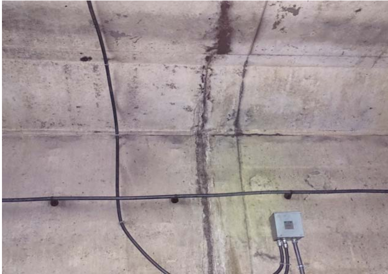
Photograph No. 197 Station 72+80 - stains and efflorescence on east wall.
