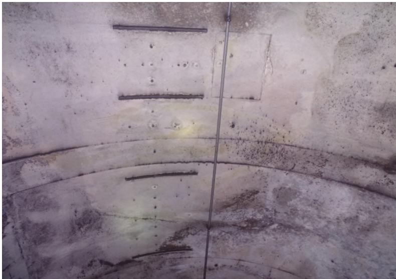
Photograph No. 303 Station 77+20 - transverse crack in ceiling.
