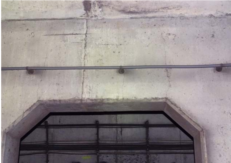
Photograph No. 341 Station 74+90 - cracks above east arch.
