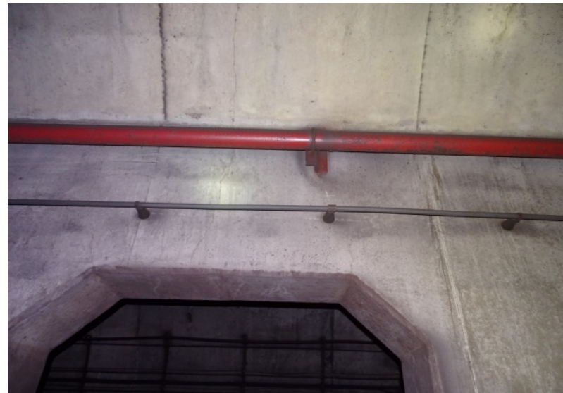
Photograph No. 236 Station 75+66 - vertical crack above west arch.
