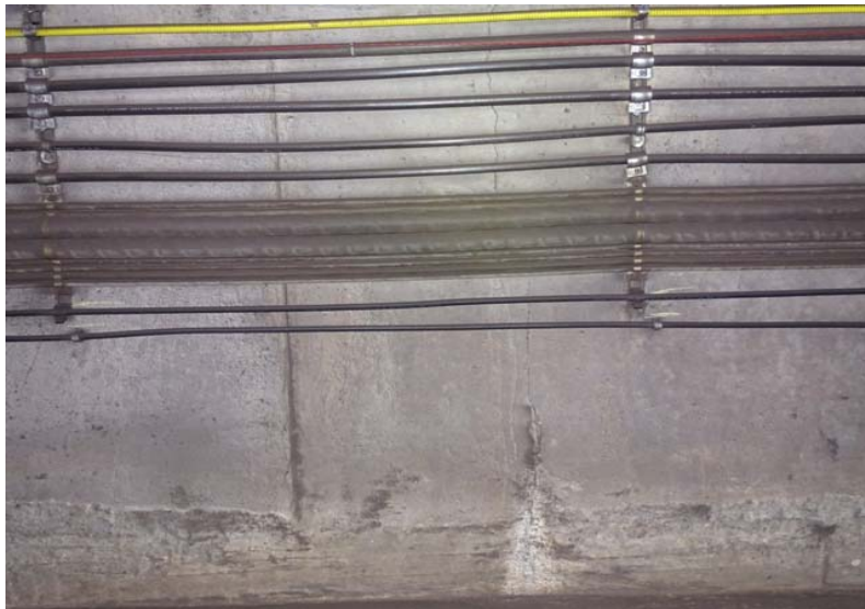
Photograph No. 85 Station 72+00 - crack on the east wall.
