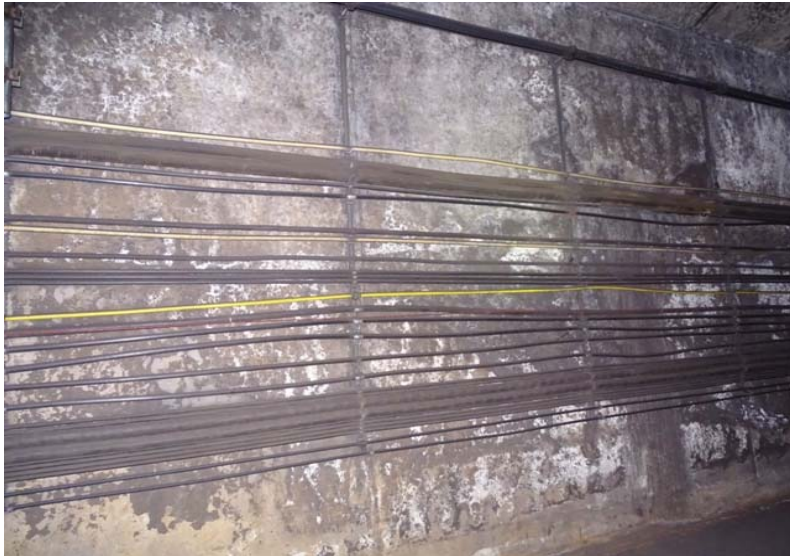
Photograph No. 51 Station 71+20 - stains on the east wall.
