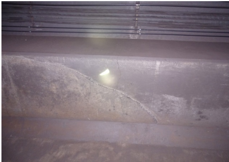
Photograph No. 279 Station 76+61 - crack in east walkway.
