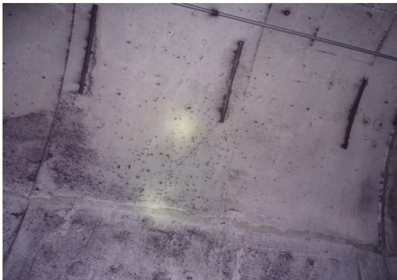
Photograph No. 361 Station 78+67 - crack in east wall.
