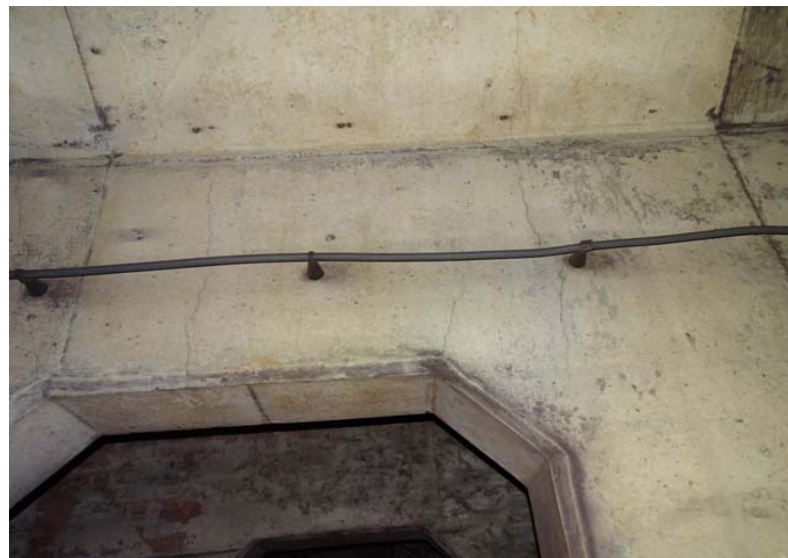
Photograph No. 86 Station 71+20 - cracks above east arch.
