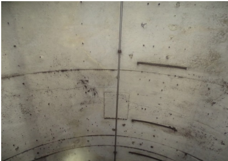
Photograph No. 355 Station 75+07 - crack on ceiling.
