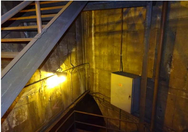
Photograph No. 75 Main room, northwest corner. Note the efflorescence.
