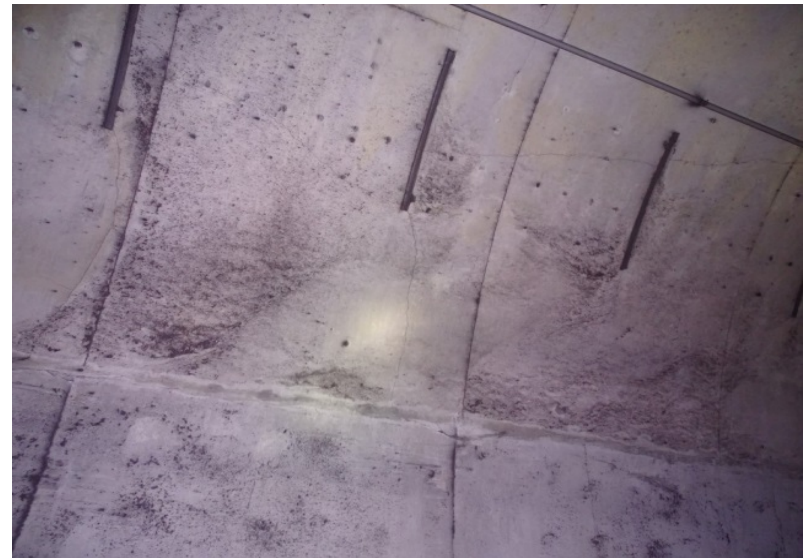
Photograph No. 376 Station 79+04 - vertical crack in east wall.
