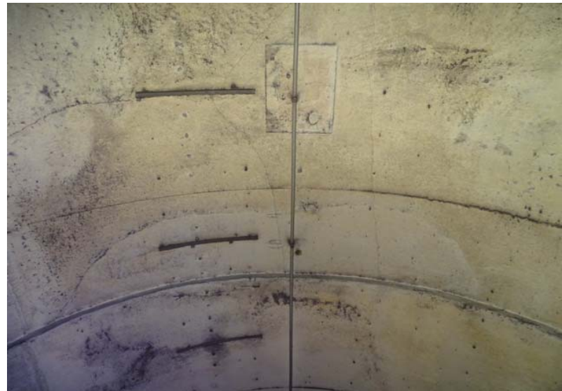
Photograph No. 184 Station 74+40 - cracks on the ceiling.
