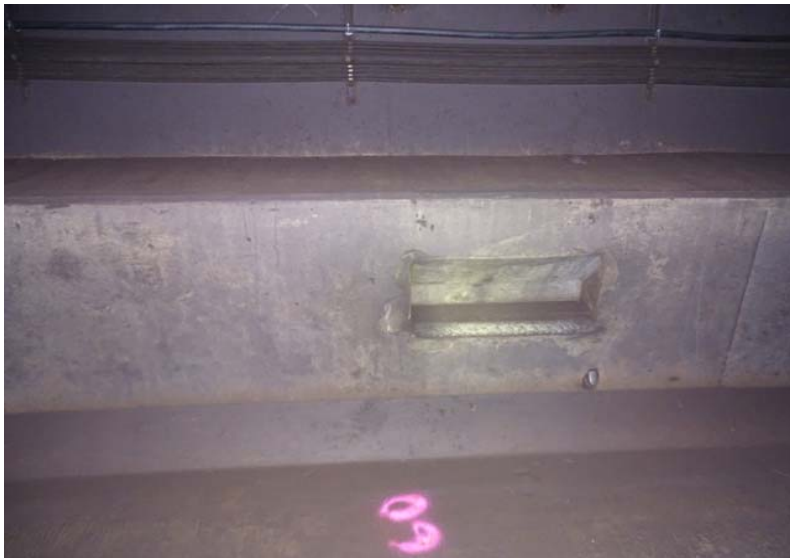
Photograph No. 323 Station 74+60 - typical foothold at side of catwalk.
