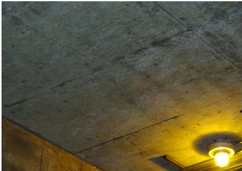
Photograph No. 107 Main room, ceiling, section 3, close up of cracks.
