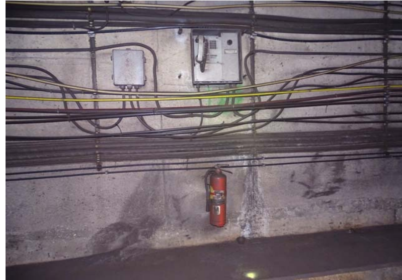
Photograph No. 130 Station 73+00 - stains and efflorescence on the east wall.
