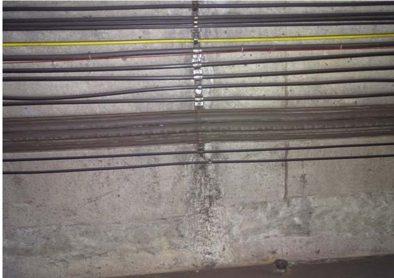
Photograph No. 153 Station 73+60 - stains and efflorescence on the east wall.
