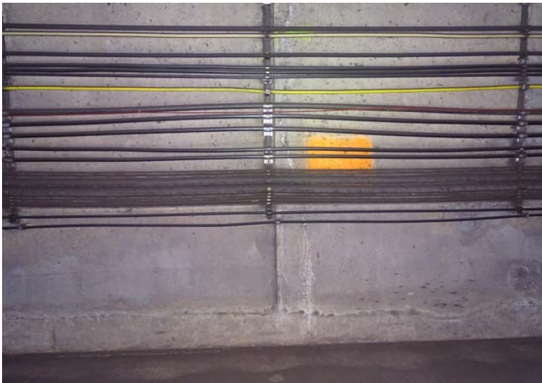
Photograph No. 123 Station 72+80 - crack on the east wall.
