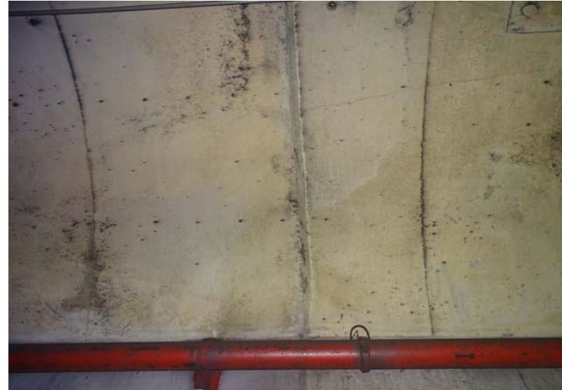
Photograph No. 186 Station 74+40 - crack and previous repair at the joint.
