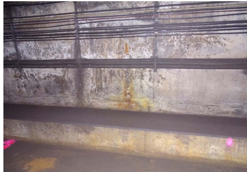
Photograph No. 112 Station 71+50, lower portion of west wall. Note the stains.
