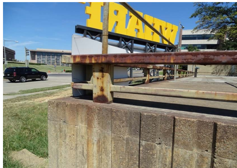
Photograph No. 180 Exterior of main vent shaft, south wall, close up of rust stains.
