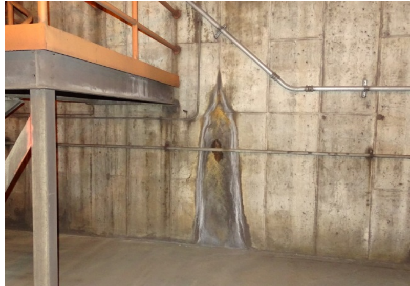
Photograph No. 166 Upper fan room, west wall, middle-north section, lower portion. Note efflorescence.
