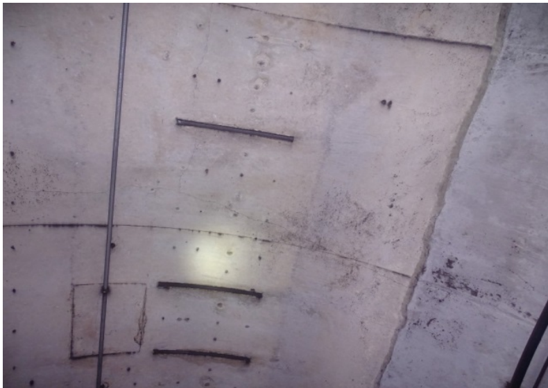
Photograph No. 523 Station 77+51 - crack in ceiling.
