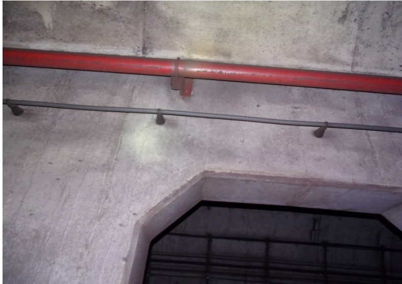
Photograph No. 285 Station 76+70 - crack above west arch.
