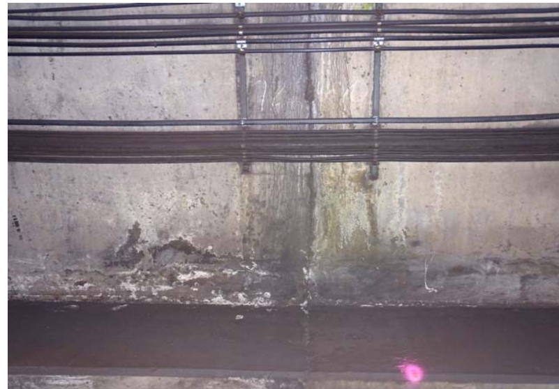
Photograph No. 232 Station 73+20 - stains and efflorescence on west wall.
