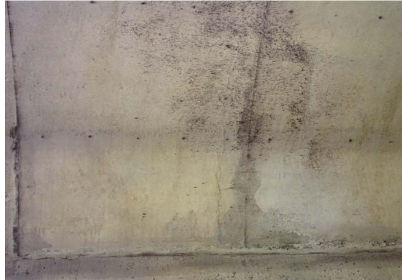
Photograph No. 326 Station 74+70 - crack and stains on ceiling, looking east.
