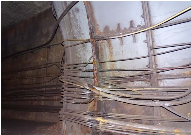
Photograph No. 35 Station 70+30 - active leak, stains, and corrosion on the west wall.
