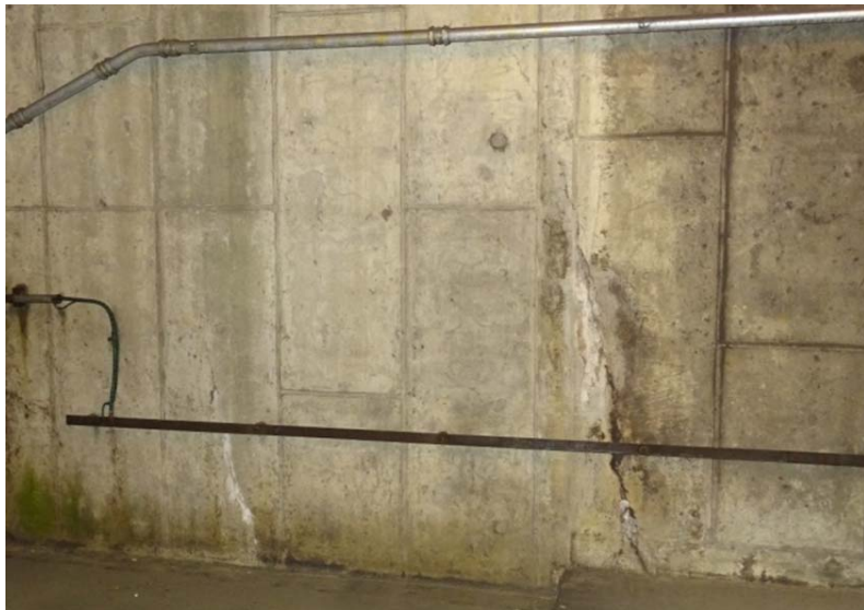
Photograph No. 135 Upper fan room, north wall, lower-west portion - vertical cracks and efflorescence.
