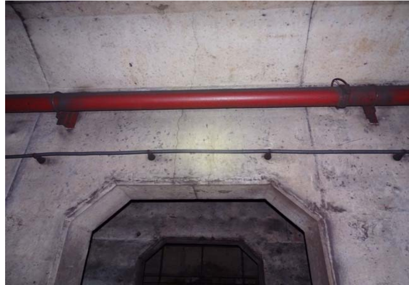
Photograph No.54 Station 71+20 - cracks above west arch.
