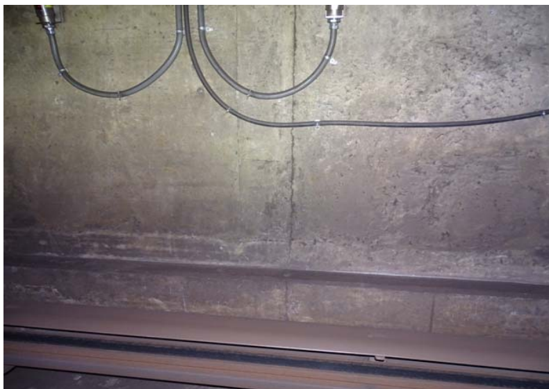
Photograph No. 119 Station 72+60 - crack on the west wall.
