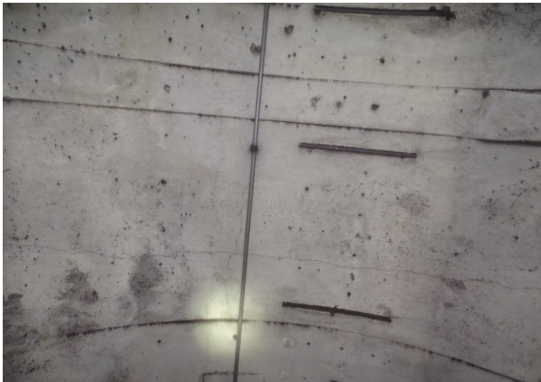
Photograph No. 363 Station 75+15 - crack in ceiling.
