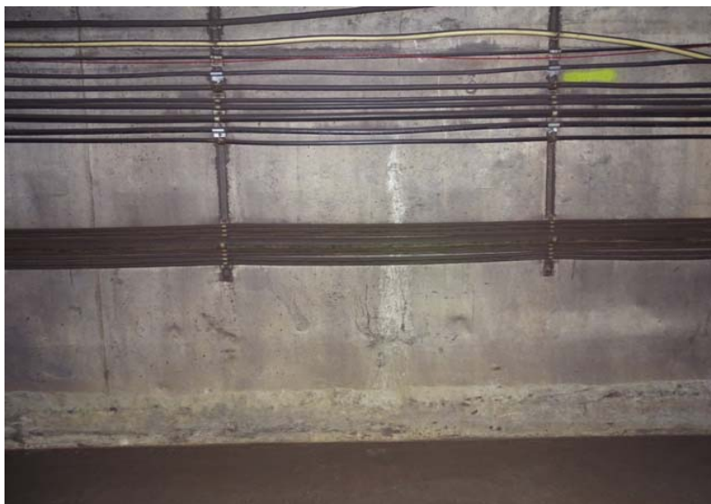
Photograph No. 155 Station 72+10 - crack and efflorescence on west wall.
