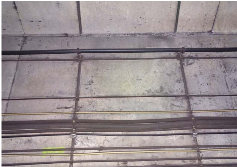
Photograph No. 111 Station 72+60 - crack on the east wall.
