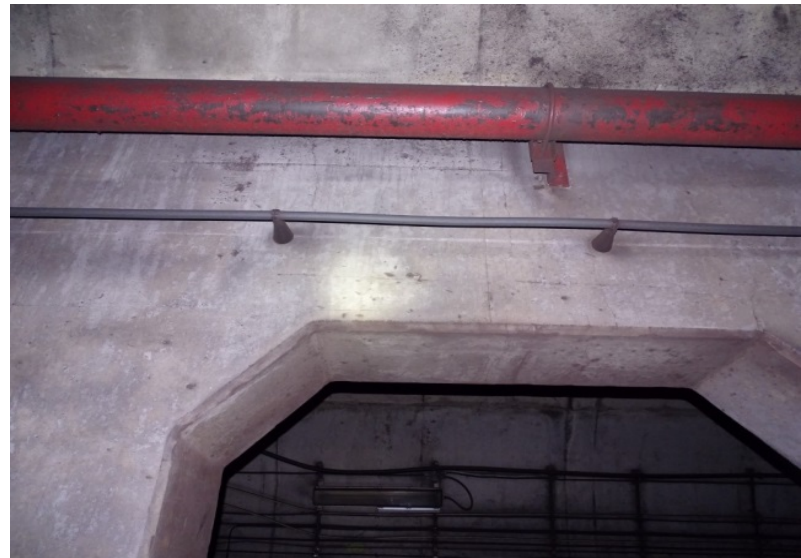
Photograph No. 216 Station 75+20 - crack above west arch.
