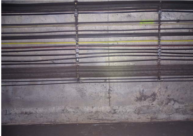
Photograph No. 105 Station 72+40 - joint on the east wall.
