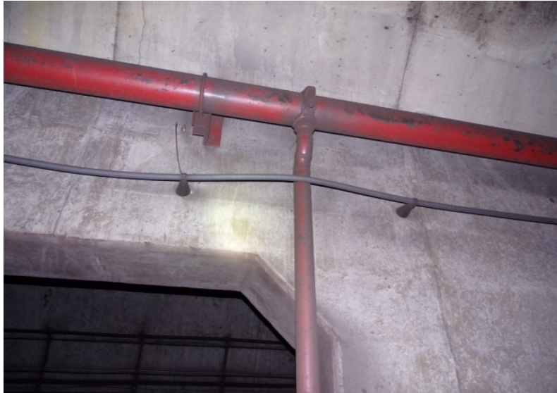
Photograph No. 225 Station 75+40 - crack above west arch.
