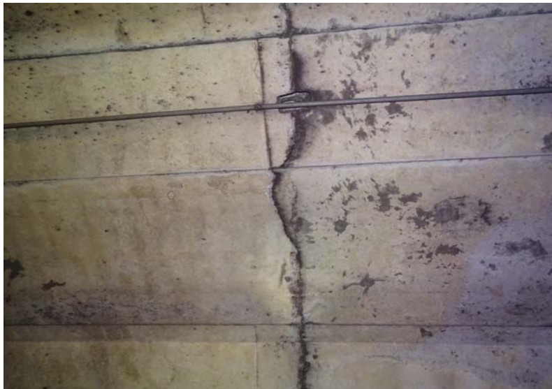
Photograph No. 117 Station 72+60 - crack on the ceiling.
