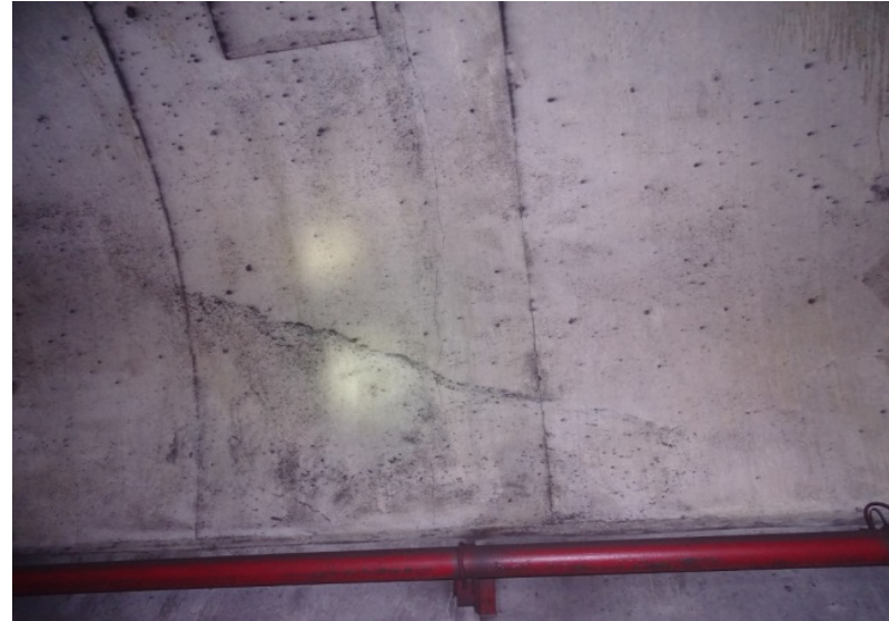
Photograph No. 282 Station 76+61 - crack in west wall.
