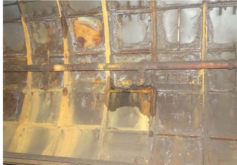
Photograph No. 22 Station 70+00 - active leak, stains, and corrosion on the west wall.
