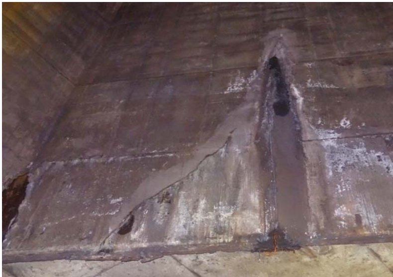
Photograph No. 35 Main room, southwest wall. Close up of the crack, stains, and efflorescence.
