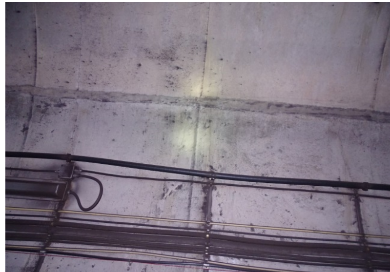
Photograph No. 252 Station 76+05 - vertical crack in east wall.
