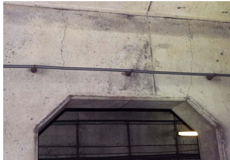
Photograph No. 264 Station 73+80 - cracks above east arch.
