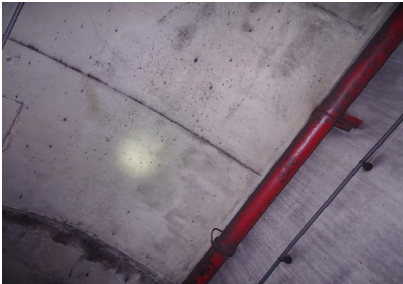
Photograph No. 219 Station 75+30 - crack in ceiling.
