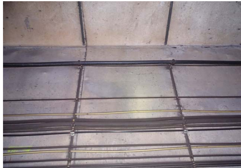
Photograph No. 72 Station 71+80 - crack on the east wall.
