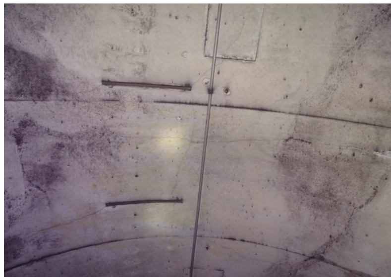
Photograph No. 368 Station 78+85 - crack in ceiling.
