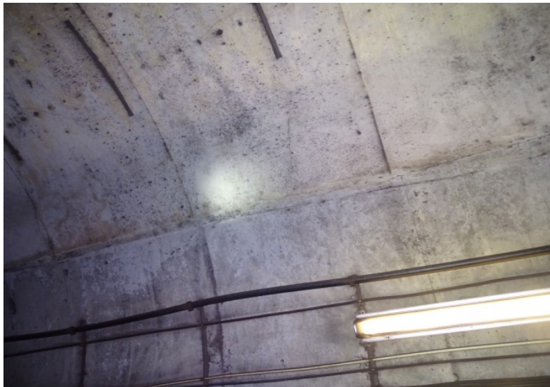
Photograph No. 397 Station 75+60 - crack in west portion of ceiling.
