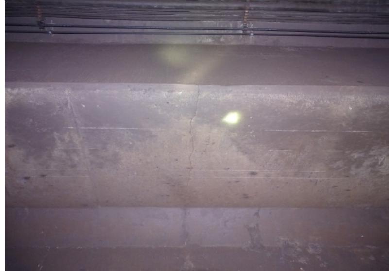
Photograph No. 302 Station 77+10 - vertical crack in east walkway.
