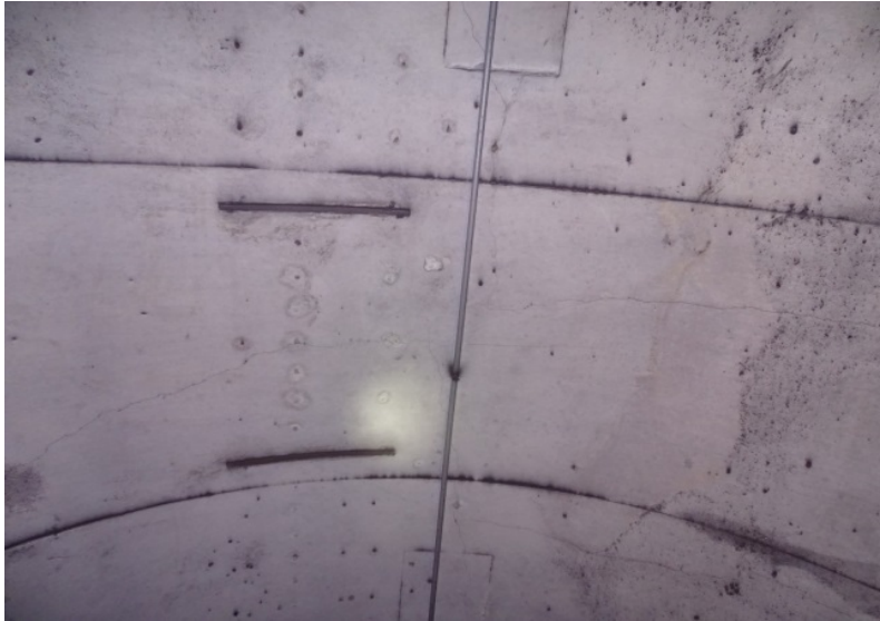
Photograph No. 209 Station 75+03 - transverse ceiling crack.
