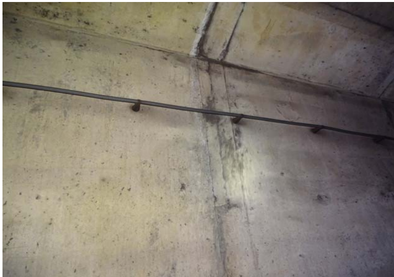
Photograph No. 225 Station 73+20 - crack and efflorescence on east wall.
