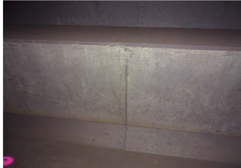
Photograph No. 330 Station 74+70 - crack on catwalk.
