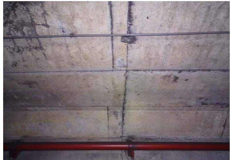
Photograph No. 96 Station 72+20 - crack on the ceiling, looking west.
