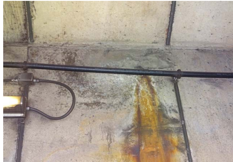
Photograph No. 90 Station 71+20 - stain and previous concrete repair on west wall.
