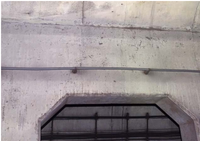
Photograph No. 319 Station 74+60 - cracks above east arch.
