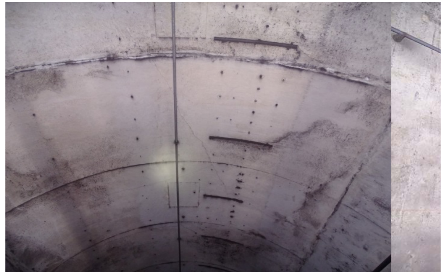
Photograph No. 556 Station 78+40 - crack in ceiling.
