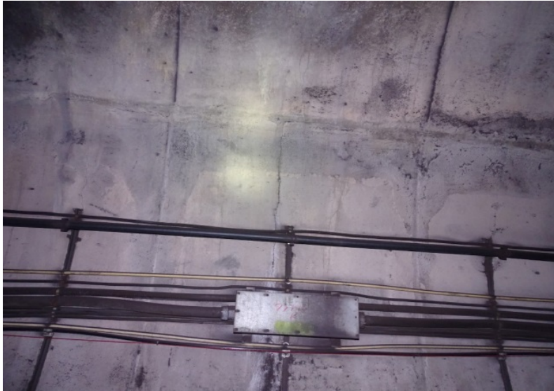
Photograph No. 301 Station 77+10 - vertical crack in east wall.
