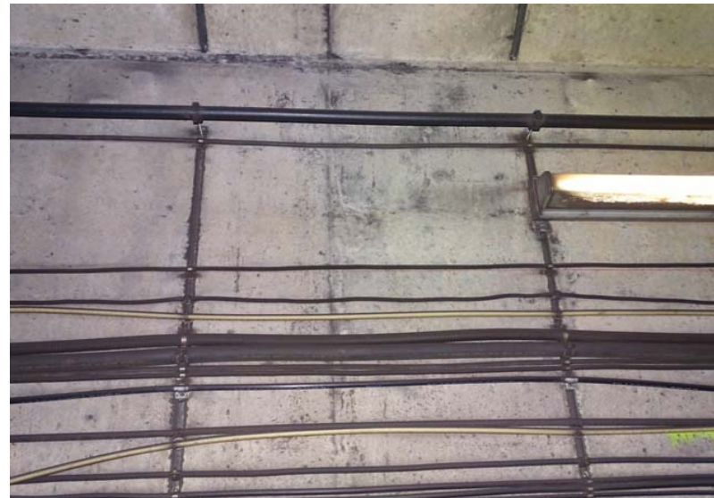
Photograph No. 132 Station 73+00 - stains on the east wall.
