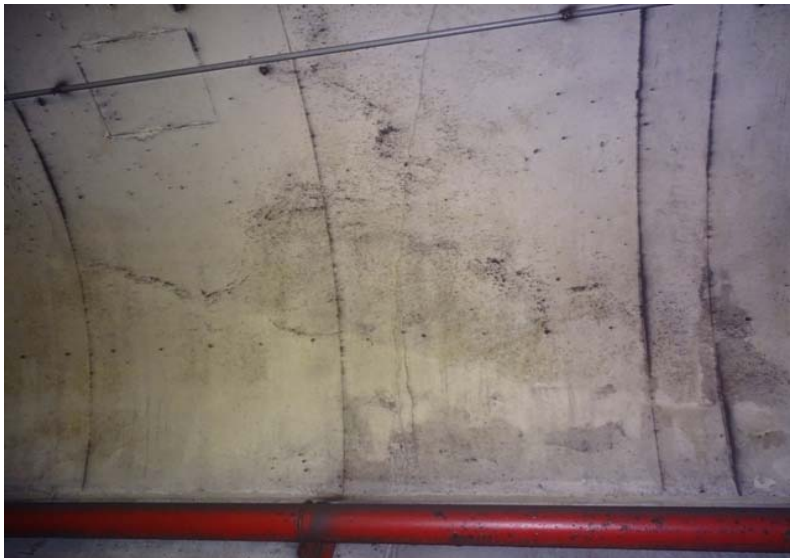
Photograph No. 195 Station 74+60 - crack on the ceiling, looking west.
