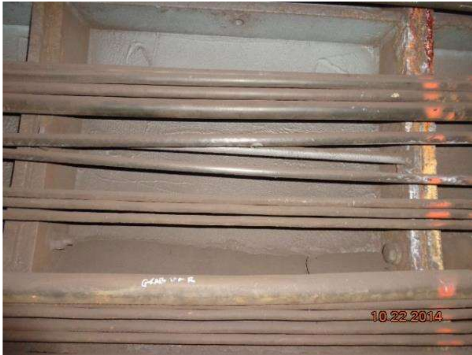
Photo 9 Grab bar covered by wires at L2 70+00
