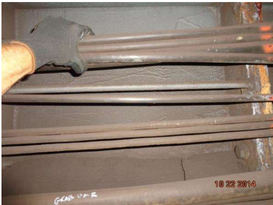
Photo 10 Grab bar covered by wires at L2 70+00
