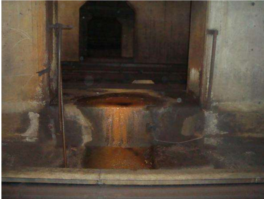
Photo 5 Overall of area of leak.
