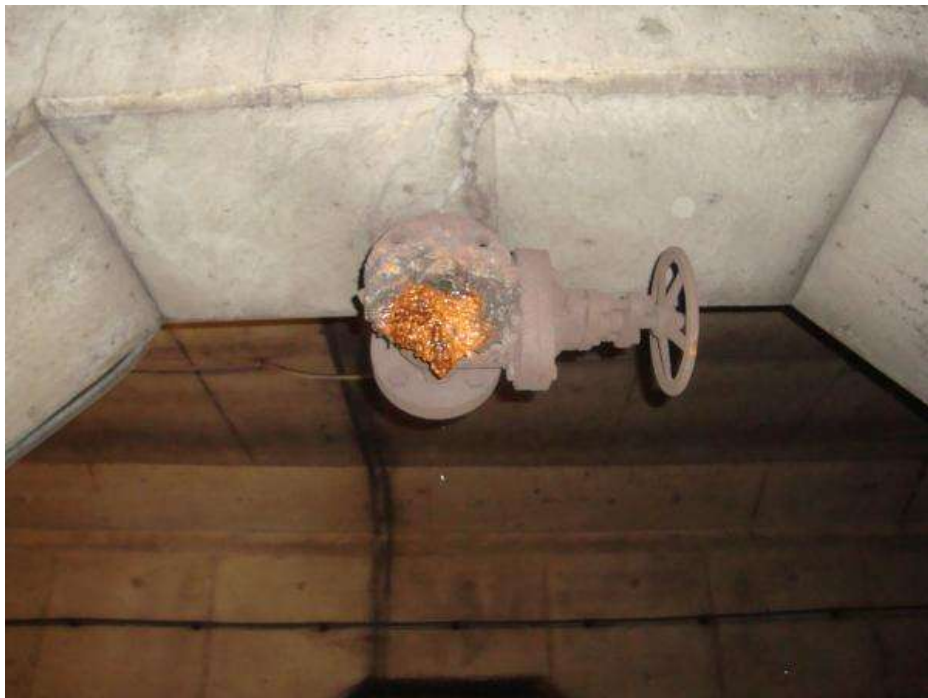
Photo 6 Pipe that is the source of leak and rusting components.
