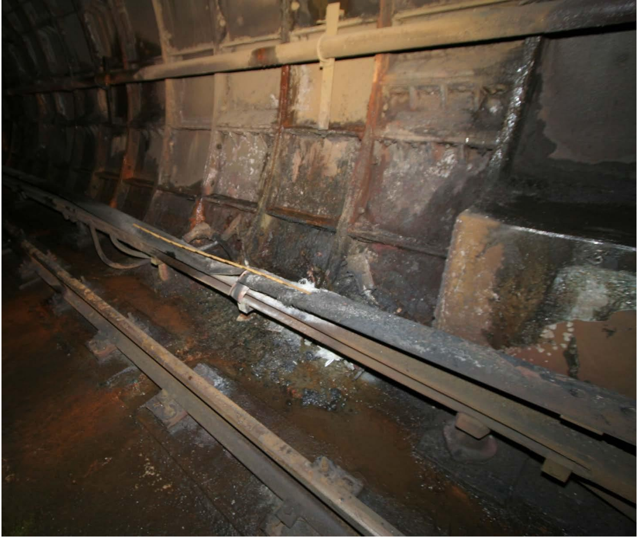
Figure: Third Rail location inside of Metrorail tunnel
