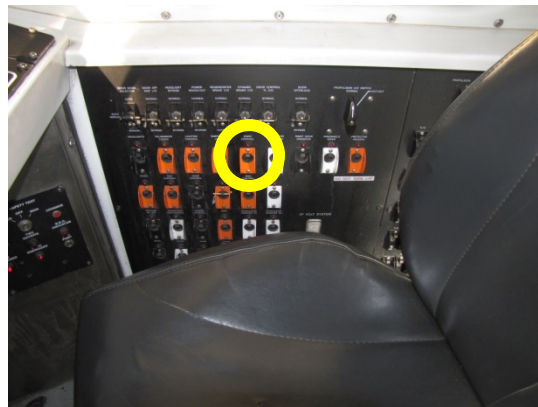
Figure 3-Circuit breaker panel of railcar 3031 with the environmental control circled
