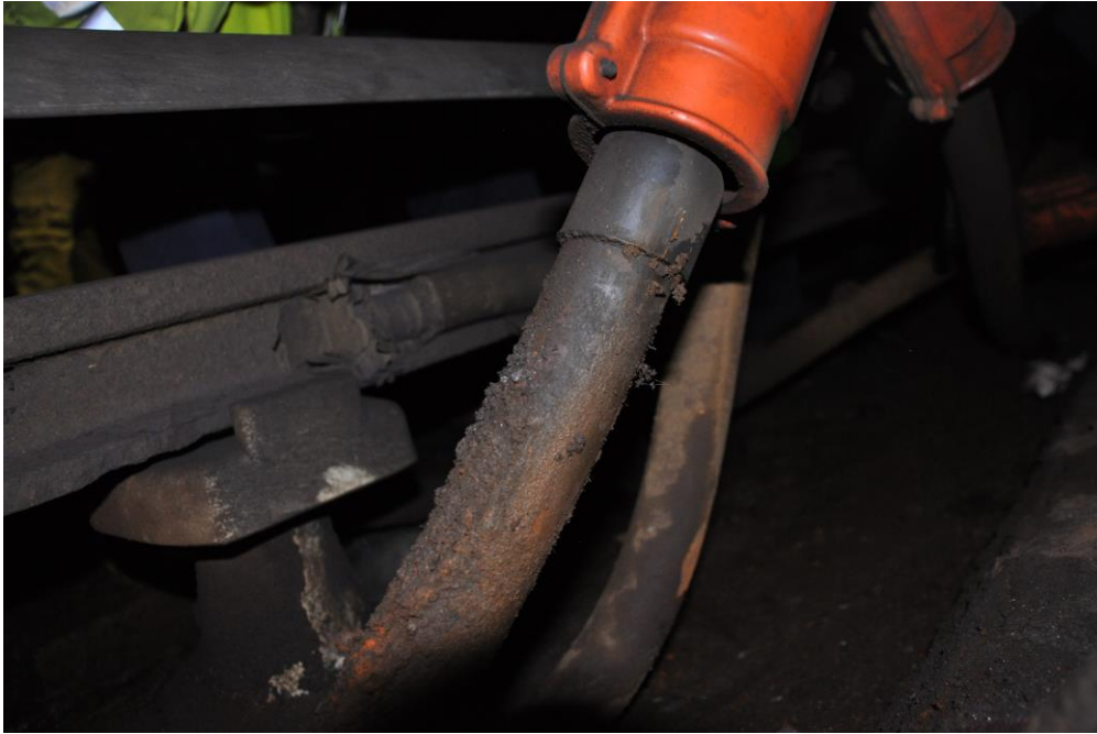
Figure 10: Jumper cable with moist debris adhering to the insulation surface.
