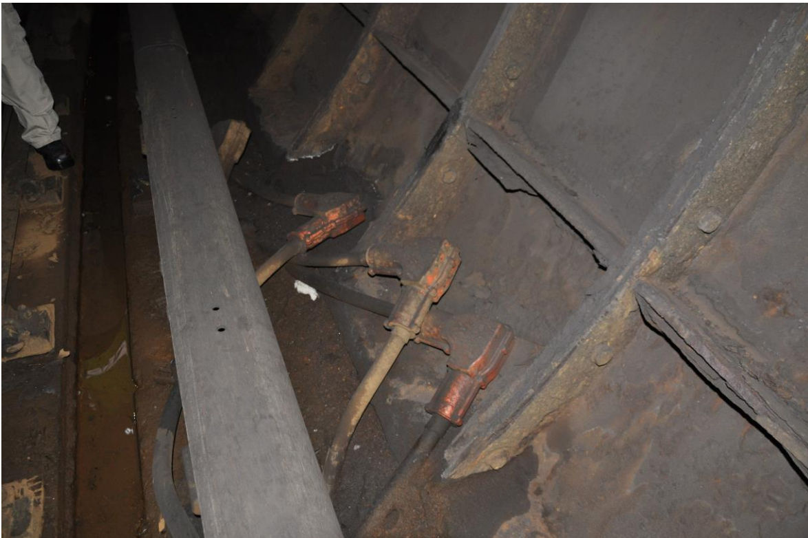
Figure 9: Jumper cable connections and boots on Track #1 of L-line at the North end of FL1.
