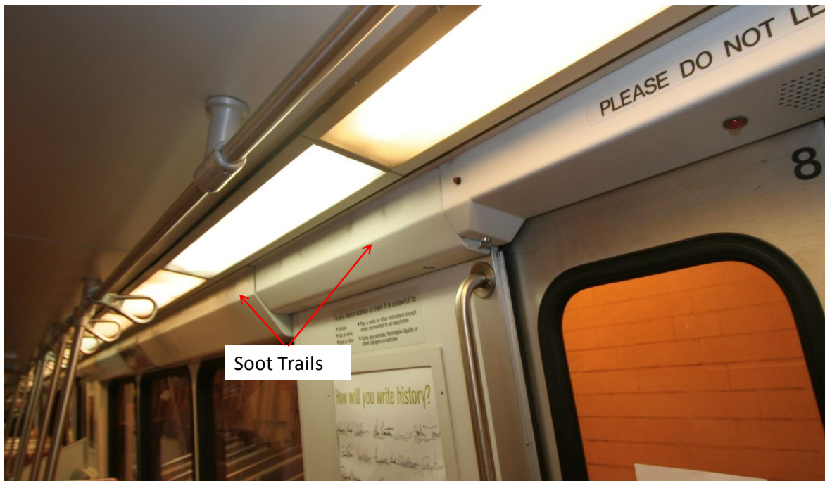
Figure 12: Soot trails seen at the ceiling vents.
