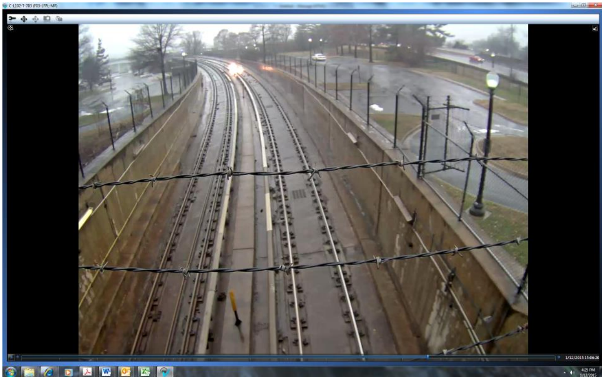
Figure 11: Arc flash captured on surveillance camera at the L-line portal exit at 15:06:20pm.
