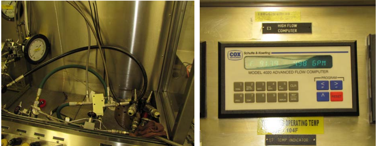
Figure 5. PV101 Setup for ATP Paragraph 5 Flow Test.
