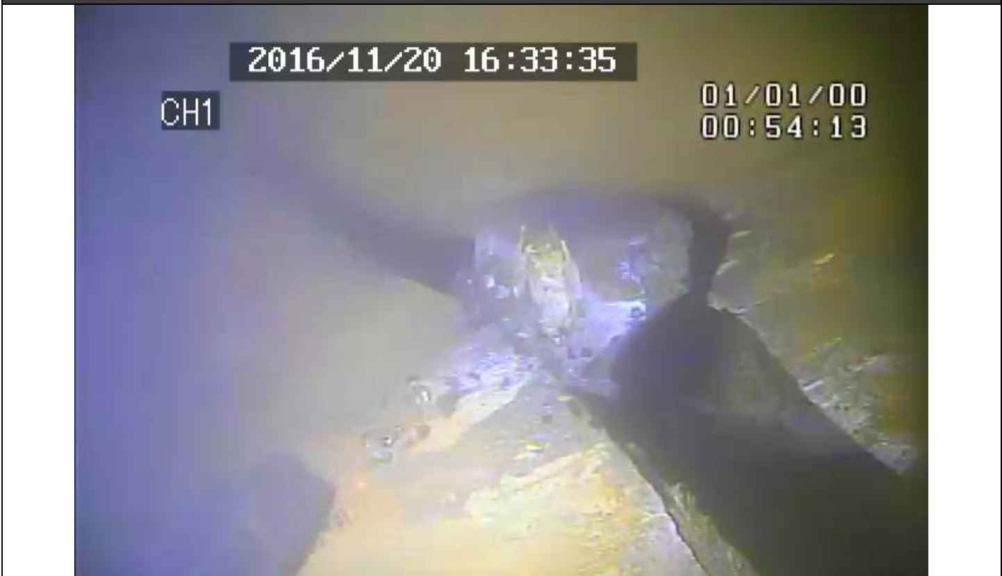
Photo #2: Tear Near Bulbous Bow
