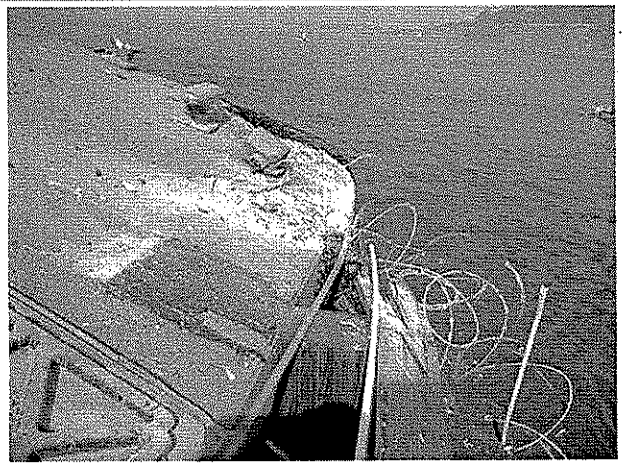
11-07-07 Damage to Pier W5 Fender on the SFOBB
