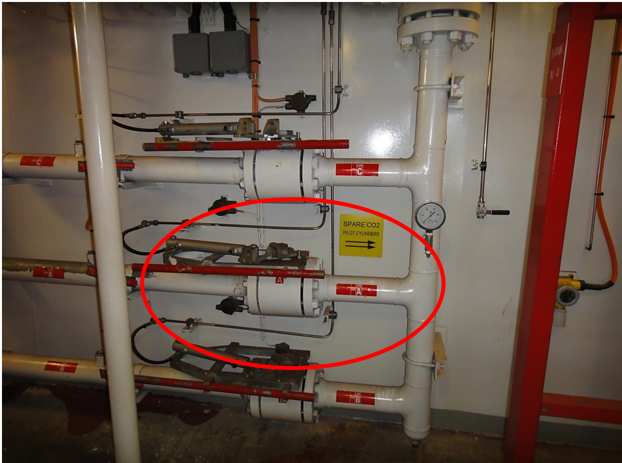
CO 2 directional valve A that had to be kicked to a fully-open position.
