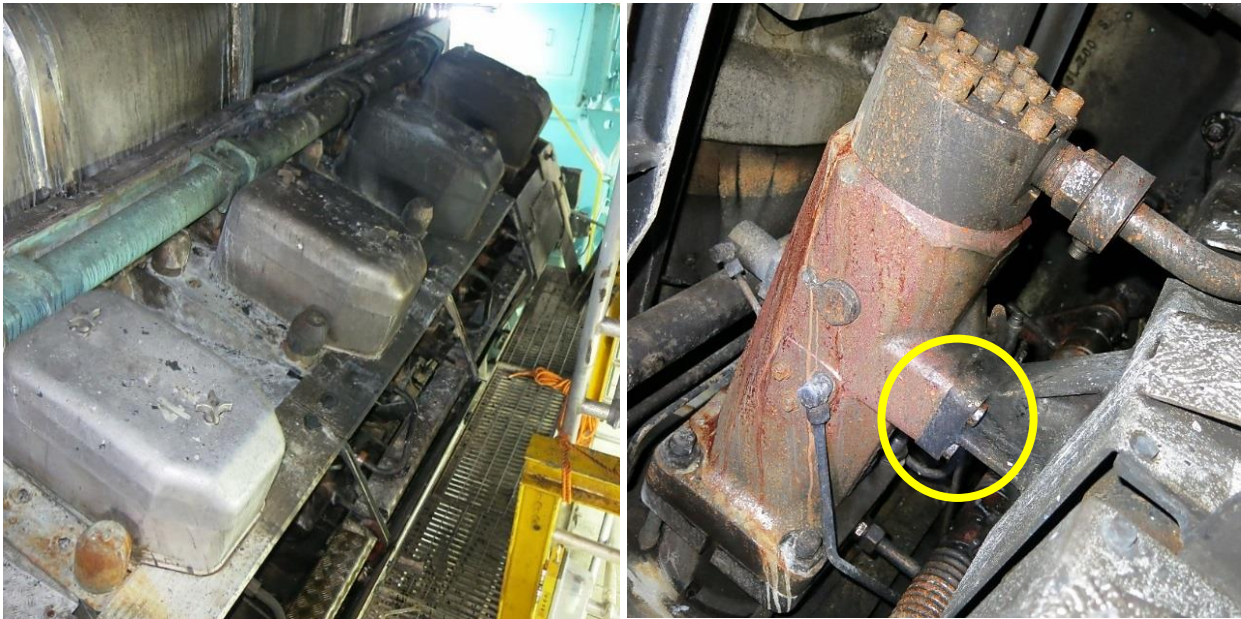
Left, location of the fire in the A bank of DG 4. Right, fuel-injection pump for cylinder A2 with suspect flange circled in yellow after the fire.
