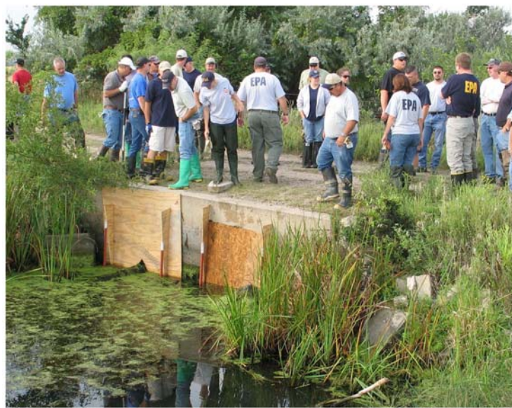
Figure 9: EPA training exercise installing an underflow dam at a culvert, Platte River Whooping Crane Maintenance Trust, Wood River, NE, August 26-27, 2008. Courtesy EPA.
