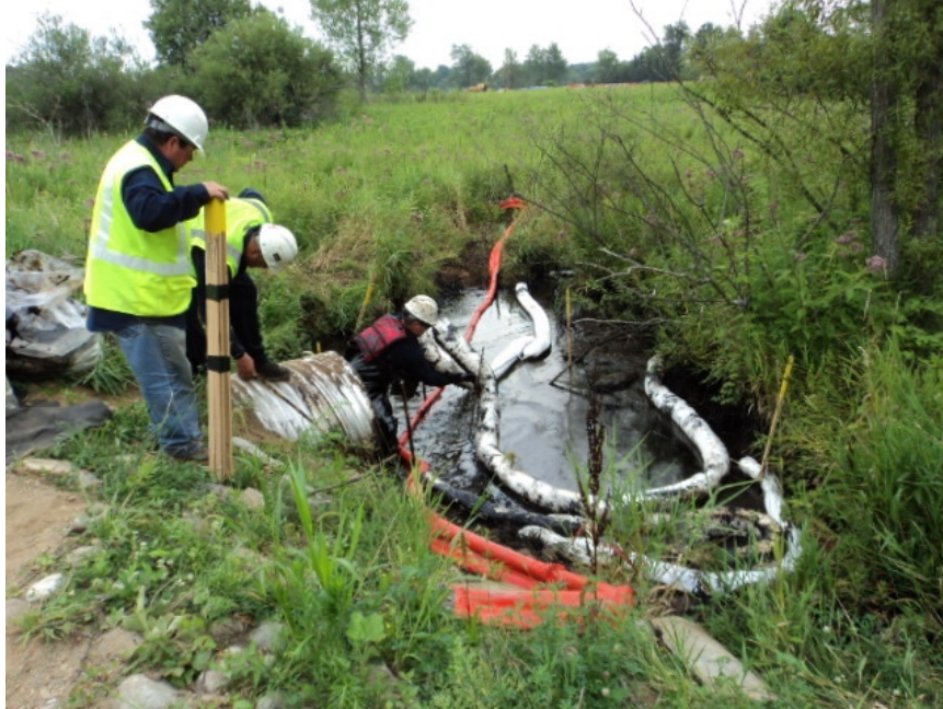
Figure 11: Installation of oil boom upstream of Division Drive culvert, August 3, 2010. State of Michigan Photograph.
