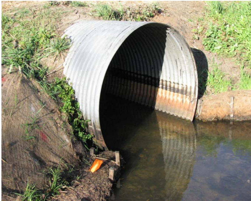
Figure 12: Oil stain line on interior of Division Drive culvert pipe showing the previous elevation of flowing oil in Talmadge Creek. October 27, 2010.
