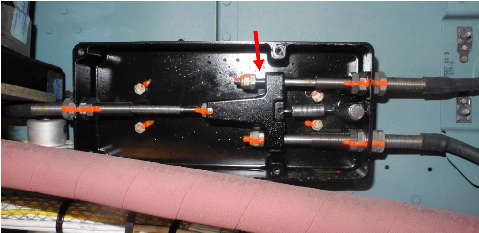
Figure 8. The junction box after removal of its cover. The red arrow points to the gap observed between the aft-upper cable nut, leading to the left reservoir assembly, and the dual cable block.
