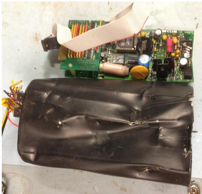
Figure 4. Insight GEM-1200 unit - internal inspection.
