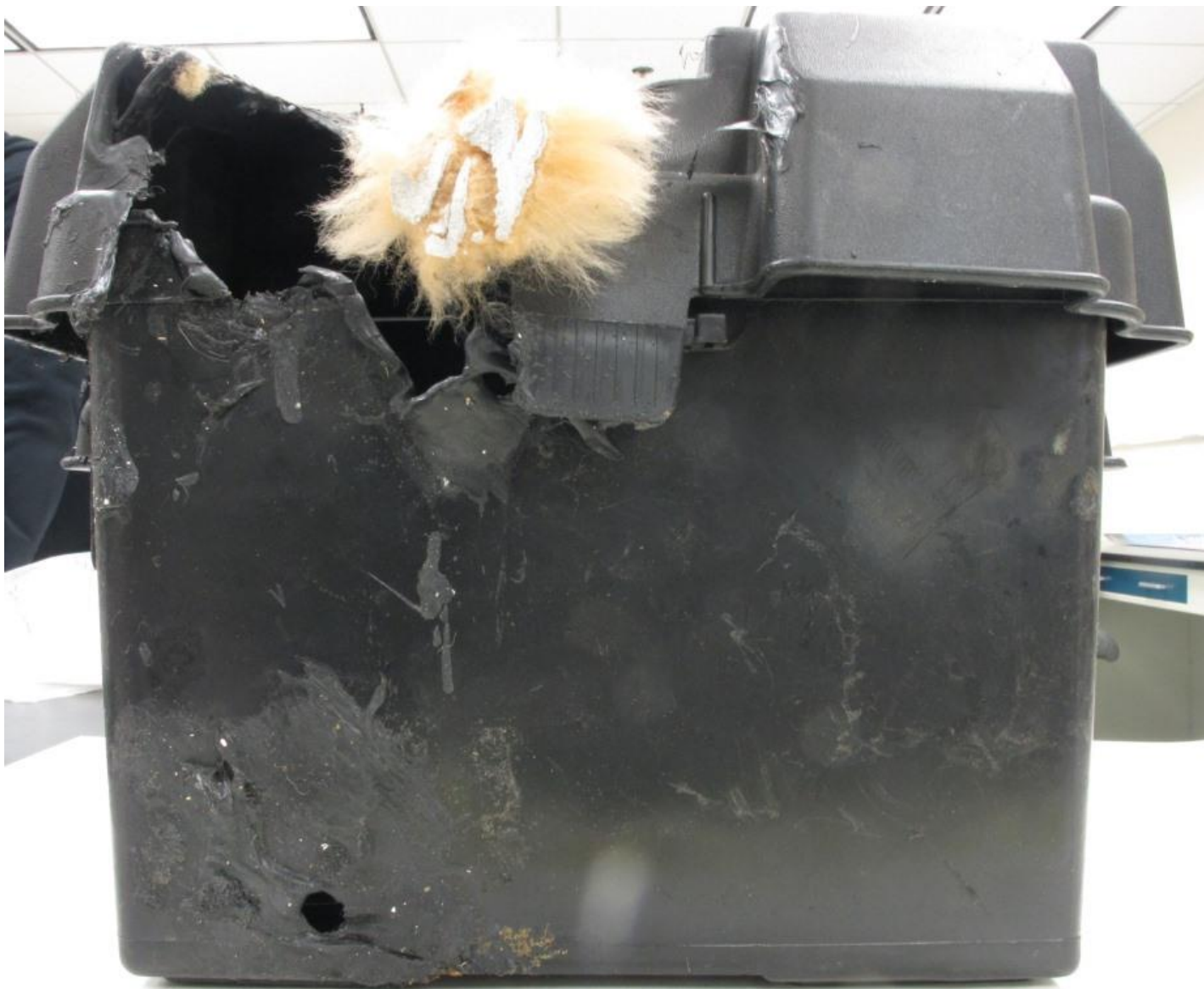
Figure 7 - Front Side of Battery Box
