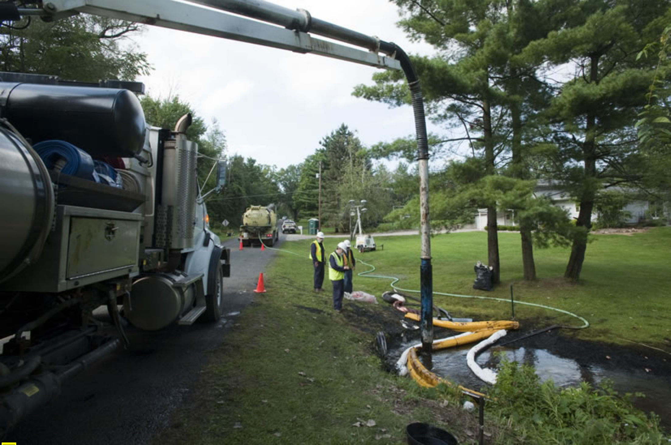
News Vacuum Oil from Talmadge Creek at 15 1/2 Mile Drive, July 28, 2010, Enbridge Photo
