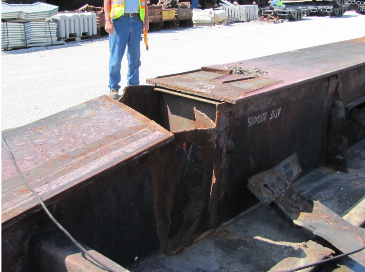
Exhibit 57-Photo Showing A-End of the Centersill Damage on BNSF 927022
