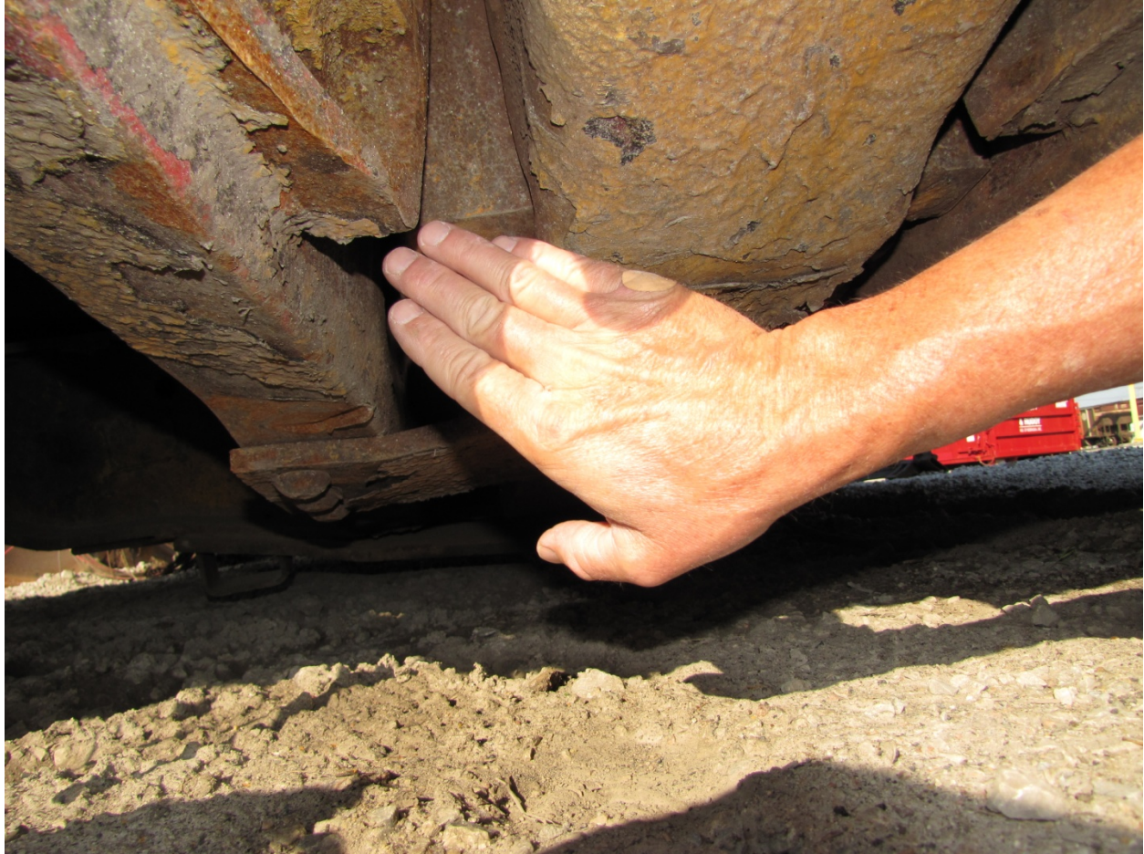
Exhibit 46-Photo Showing Compressed Draft Gear of the Struck End on HZGX-150 Clip Car
