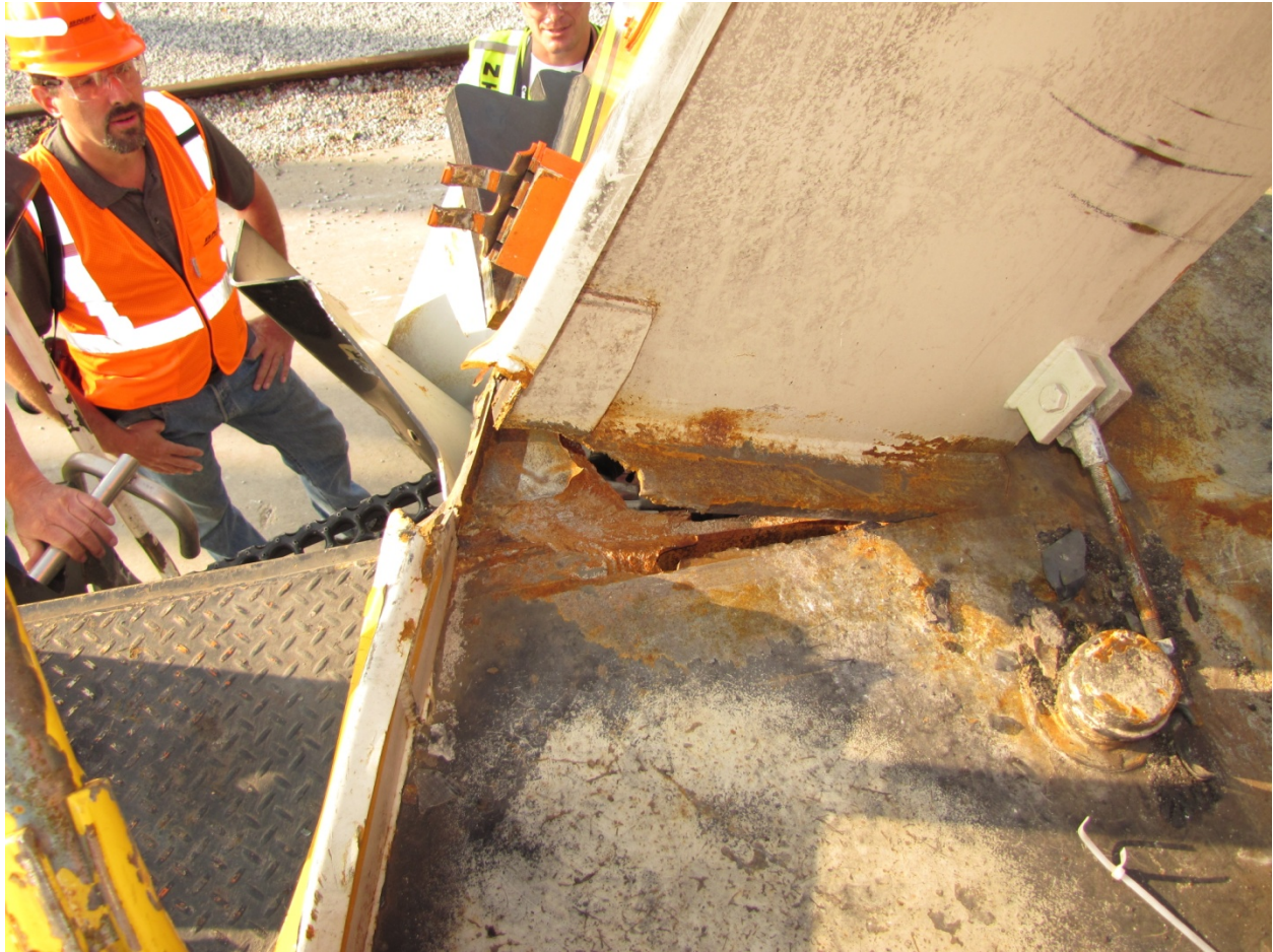
Exhibit 30-Photo Showing Right Side Collision Post Torn Away from Top Plate on BNSF 9159
