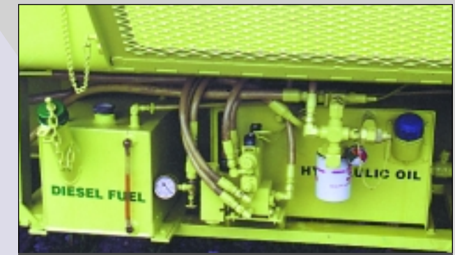
Hydraulic & Fuel Tanks
