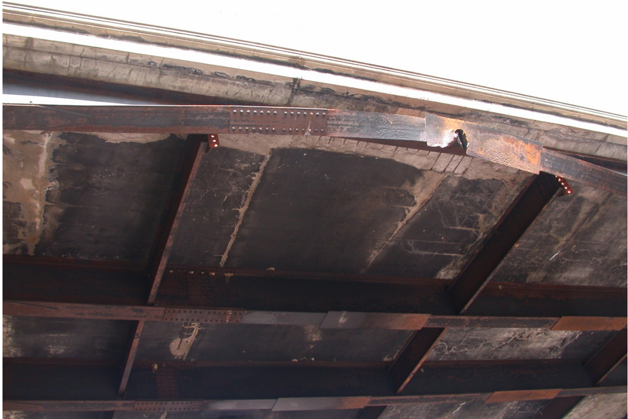
Exhibit 17- Photo Showing East Face of Overpass with Damage to the I-Beam
