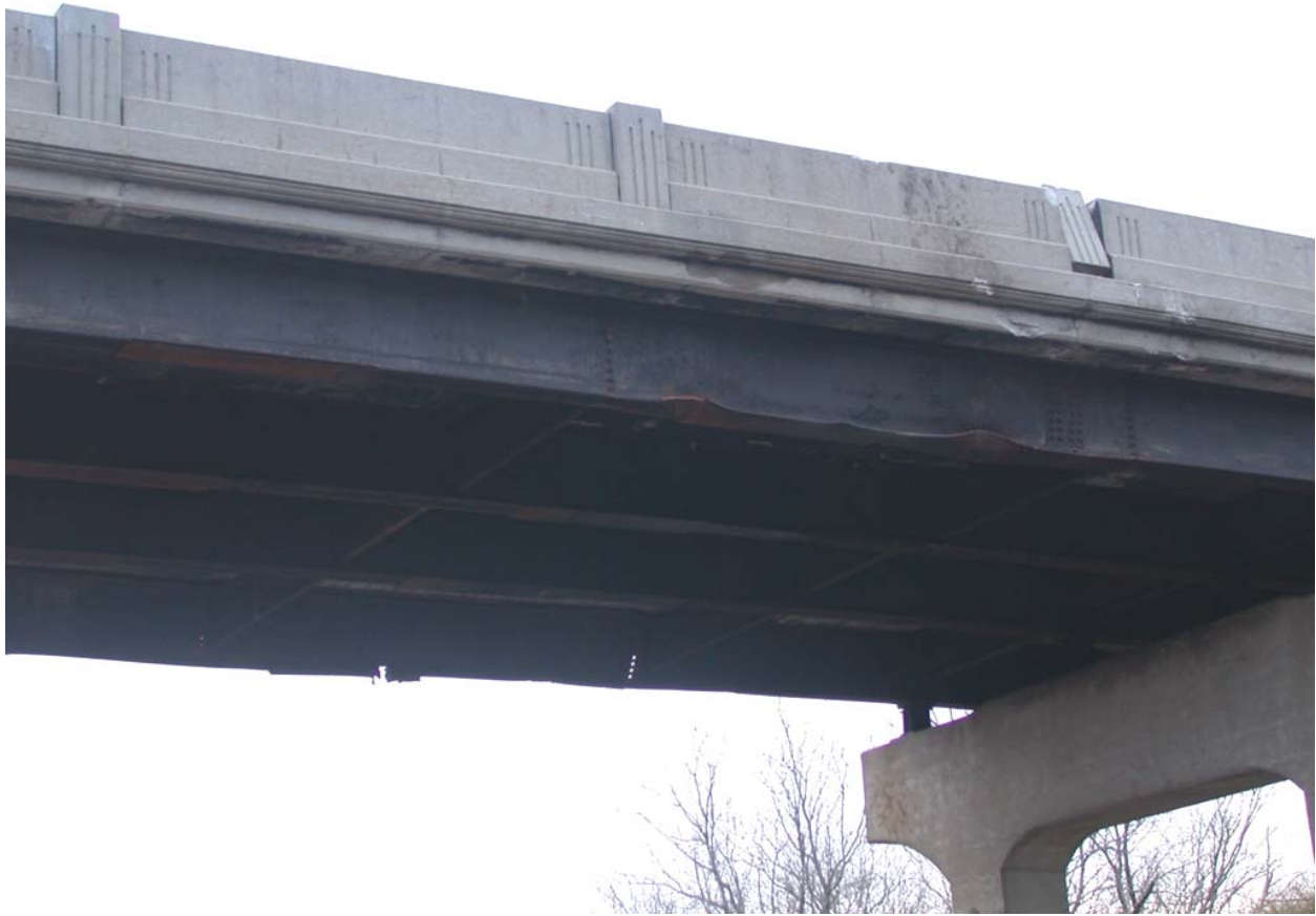
Exhibit 16-Photo Showing West Face of Overpass with Damage to Concrete Span and I-Beam above Centerline of Main Track Number Two
