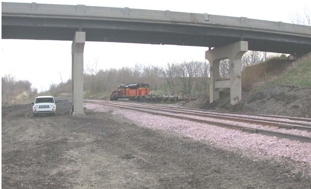
Exhibit 15-Photo Showing West Face of Overpass with Damage to Concrete Span and I-Beam above Centerline of Main Track Number Two
