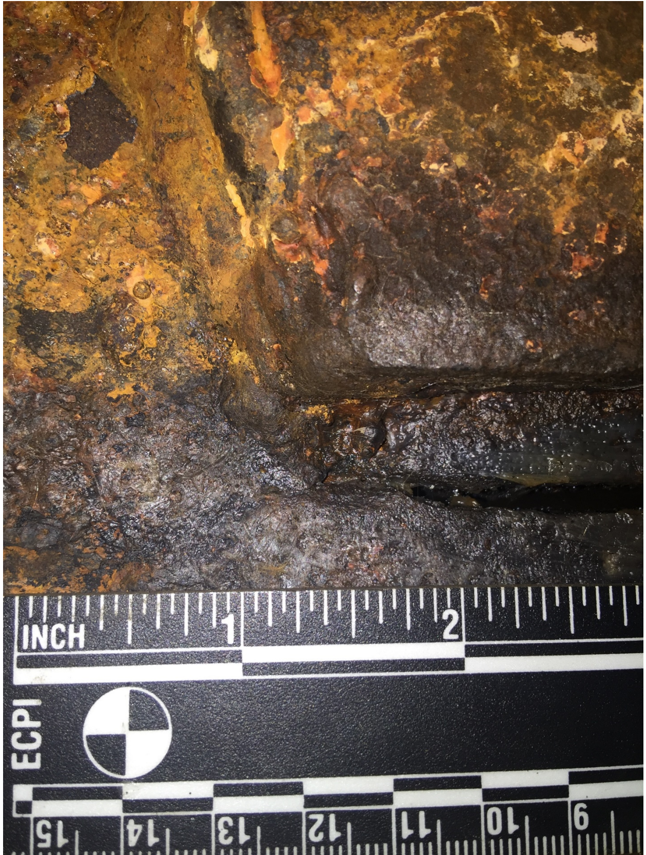
A-R cradle pad termination of A-6 fillet weld and tank shell crack termination point
