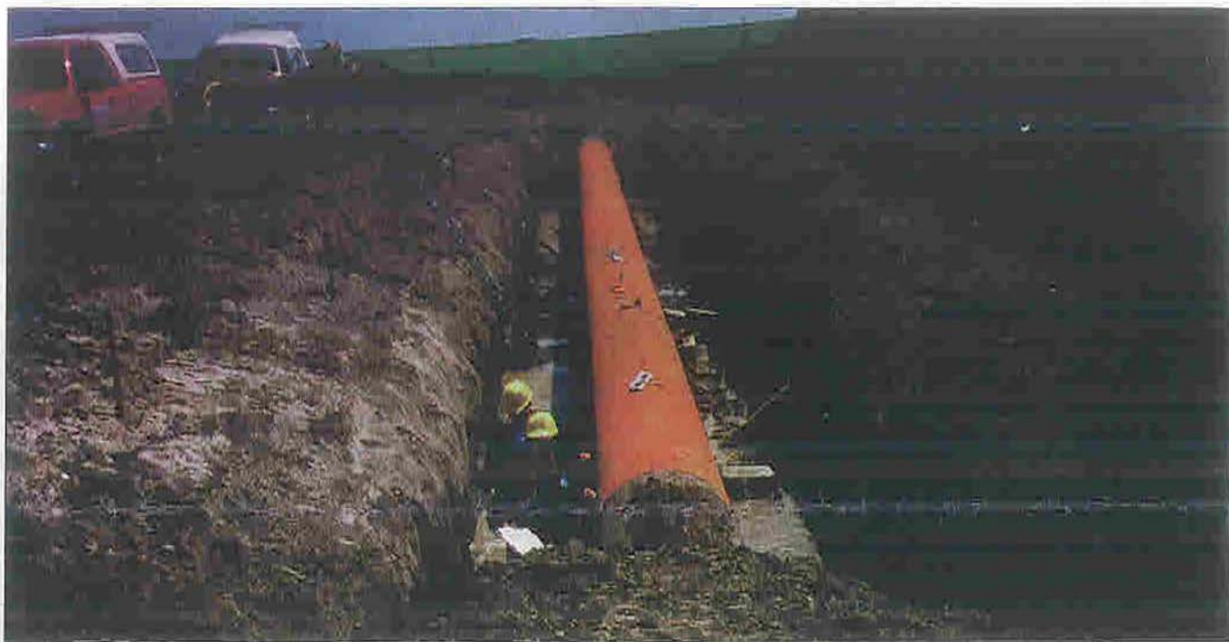
Crews excavate a section of Line 3 to verify results of the EW-vehicle analysis (Fig. 5).
