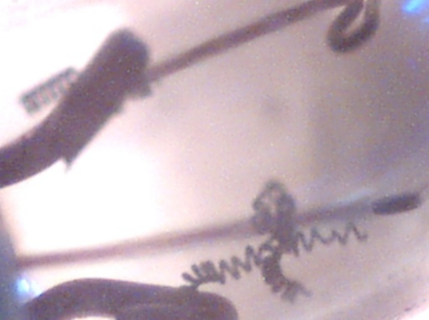
Control Panel Photo 47 - Taxi Lt - Bulb B
