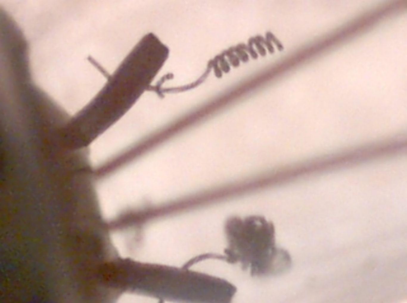
Control Panel Photo 42 - Master SW - Bulb C View 2
