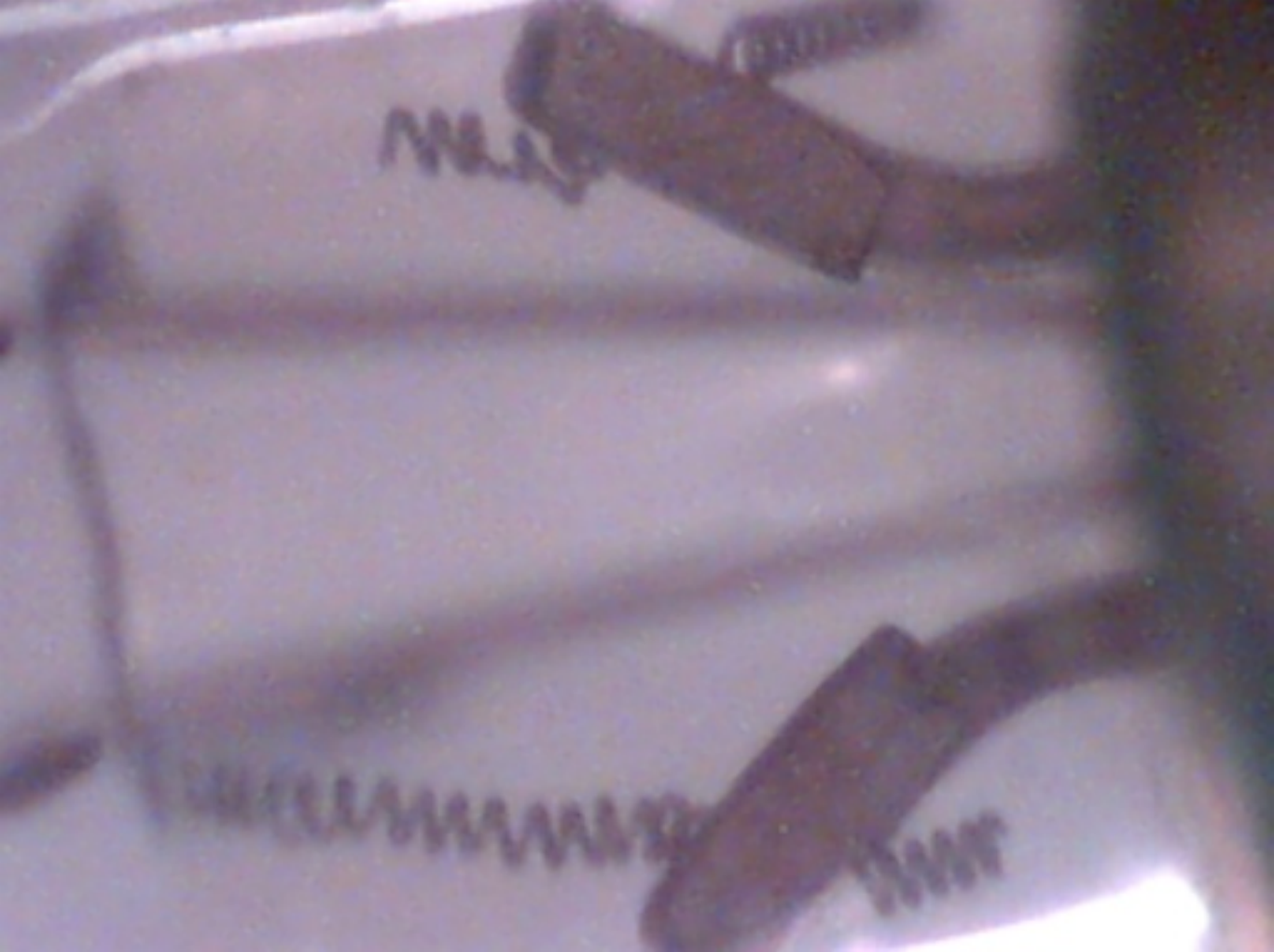
Control Panel Photo 32 - Inst Lights 2 - Bulb B
