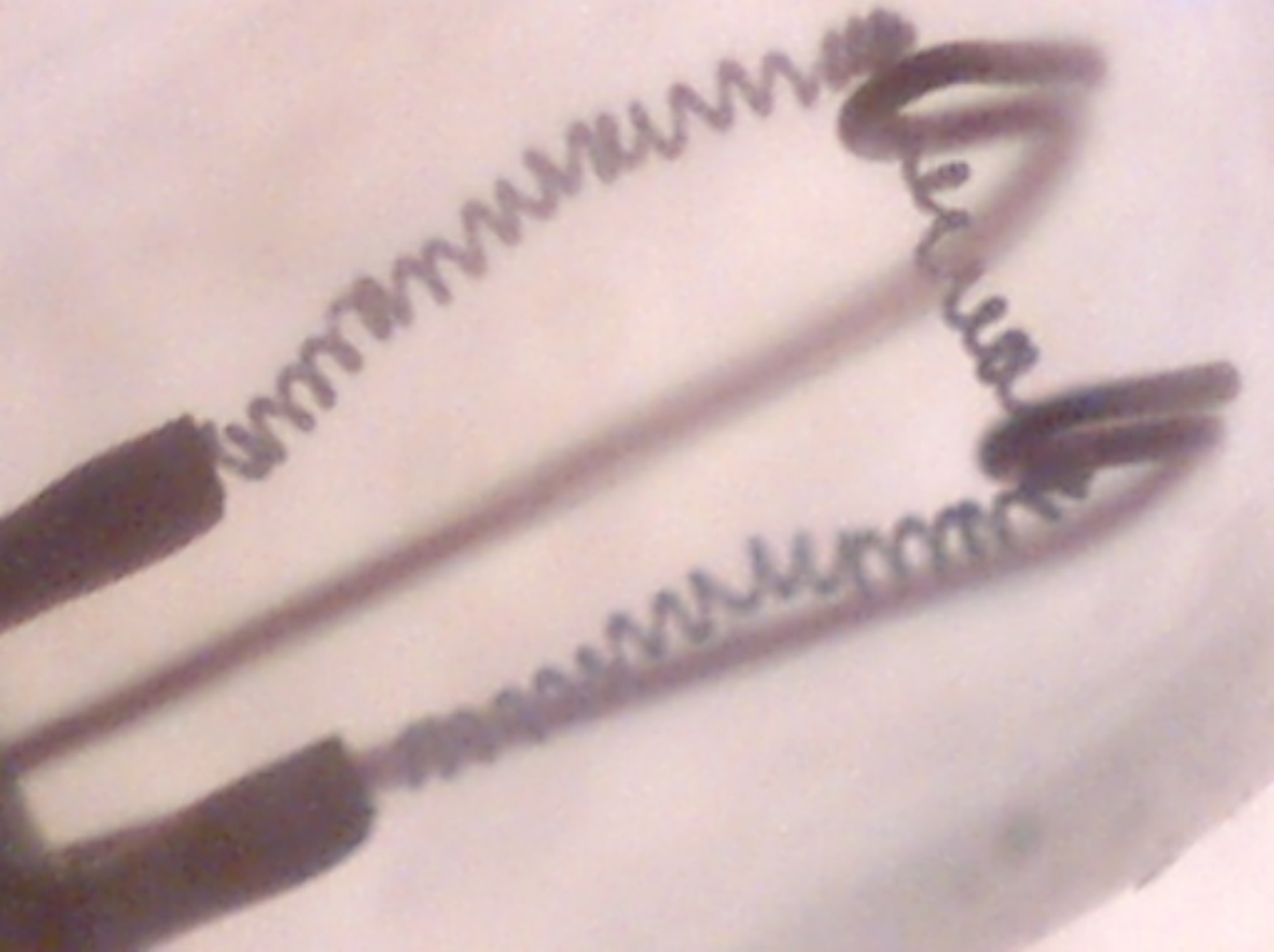
Control Panel Photo 28 - Inst Lights 1 - Bulb B
