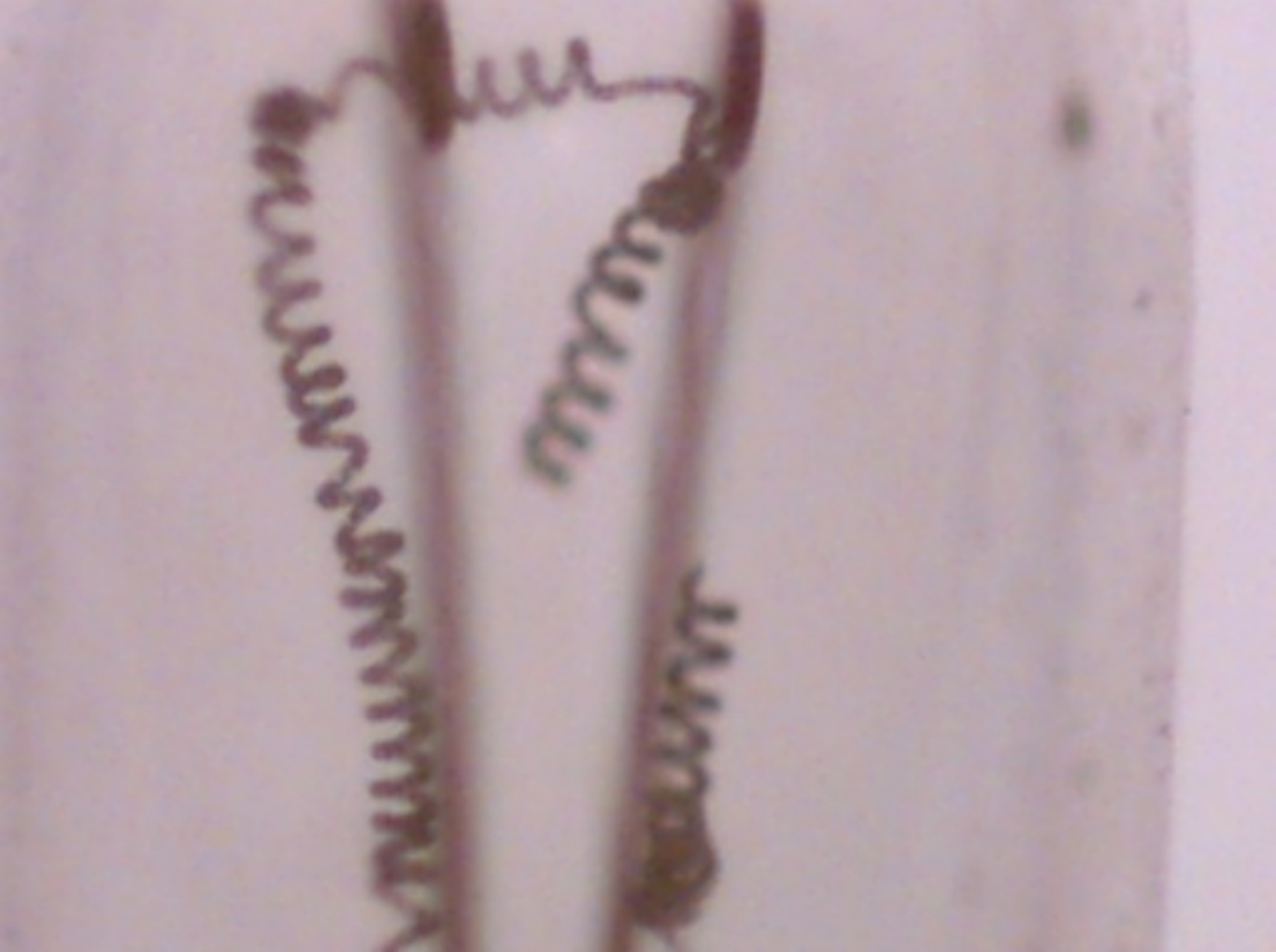
Control Panel Photo 23 - Horn - Bulb A
