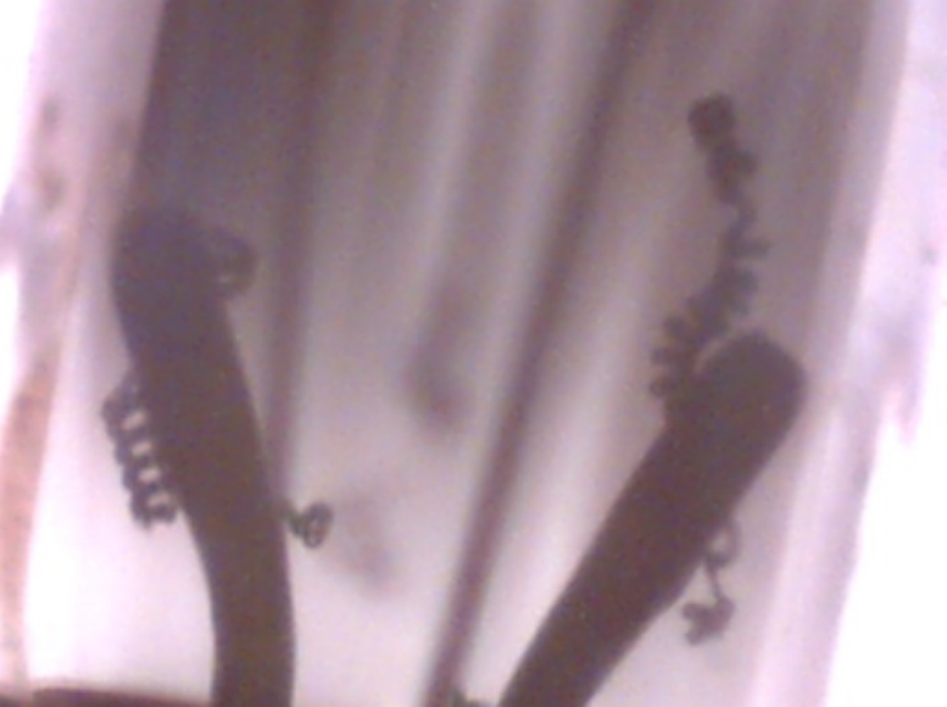
Control Panel Photo 18 - Gen - Bulb A View 2
