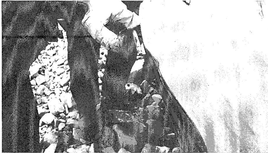
Figure 1: Thinning of shell of UTLX211623
