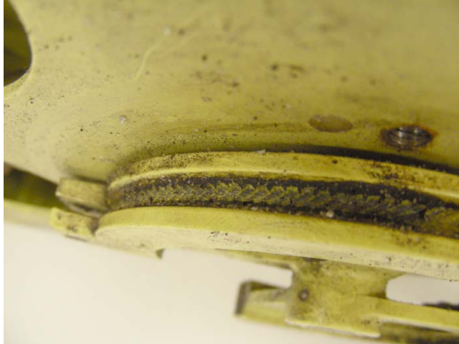
Figure 15. View of the cable groove on the 6261060-6 quadrant assembly showing wear due to contact with the control cable. Wear of the cable groove of the 6261060-5 quadrant assembly was similar.
