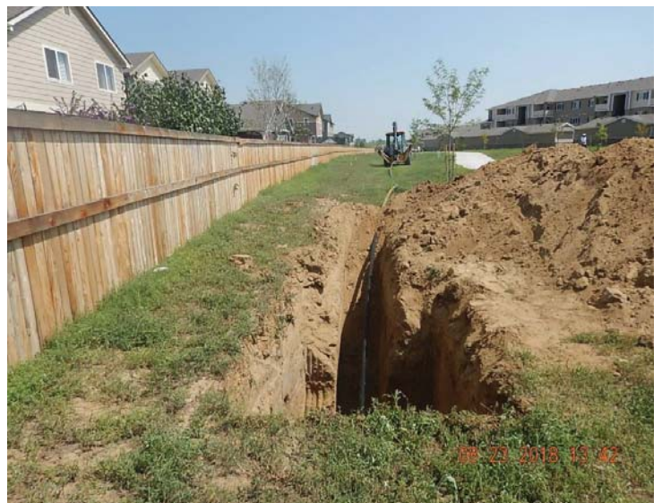
Flowline removal in progress (Previously Active Coors V 6-14JI line) east of Oak Meadows Blvd in ROW south of subdivision.
