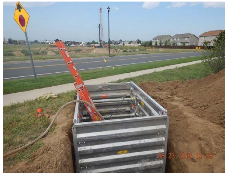
View of excavation/ trench box; Previously abandoned flowline 2" from Coors V 6-13 being cemented (full) at Oak Meadows Blvd; 1: poly line segment abandoned with ends sealed. View to west
