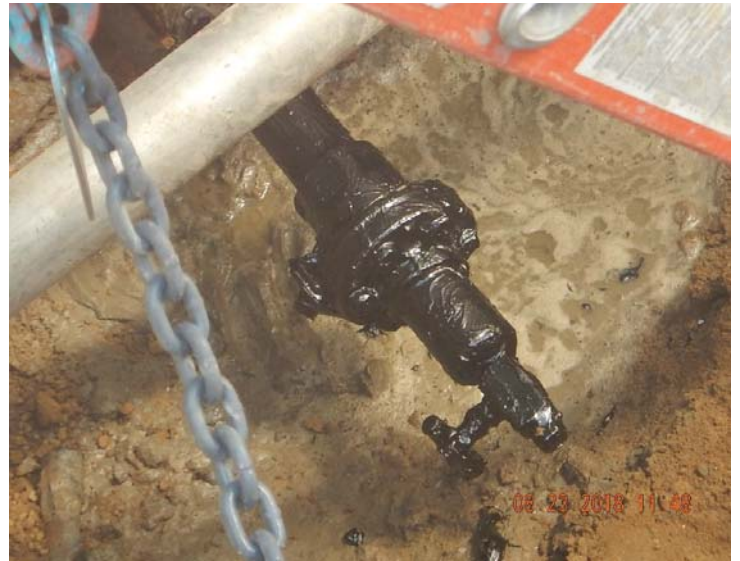
Abandoned flowline segment; ends plugged & sealed. Valves and fittings tar coated.
