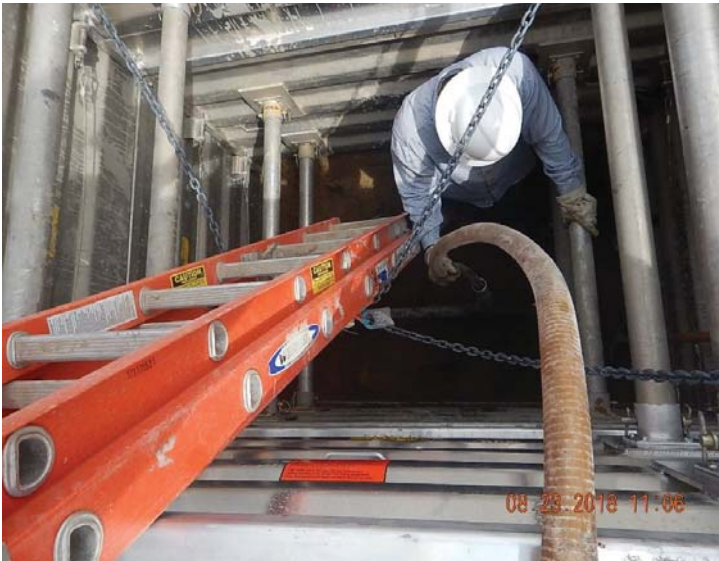
Coors V 6-13 flowline segment (18' long) being cemented, plugged and abandoned in place at Oak Meadows Blvd
