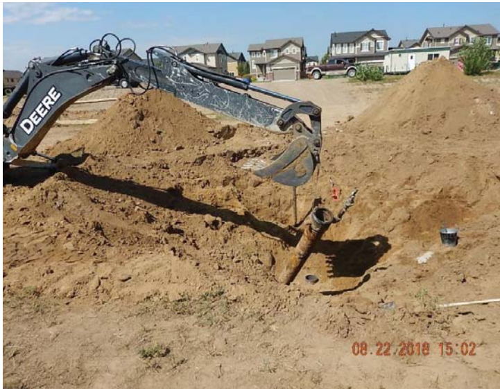
Final stage in plugging and abandonment of the Coors V 6-14JI well – cut and cap of casing after being cemented
